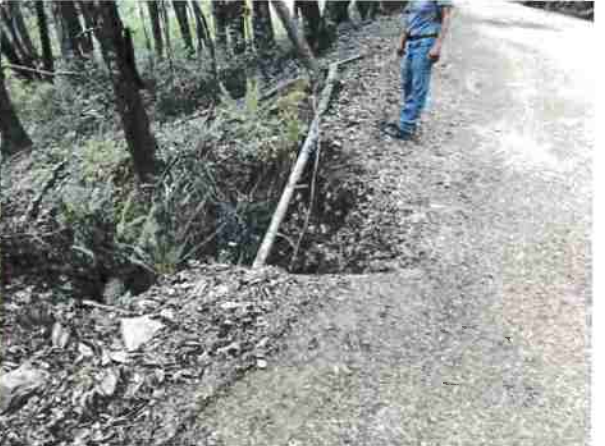
Photo #216, location 53 south side of road 18" cmp outlet.
