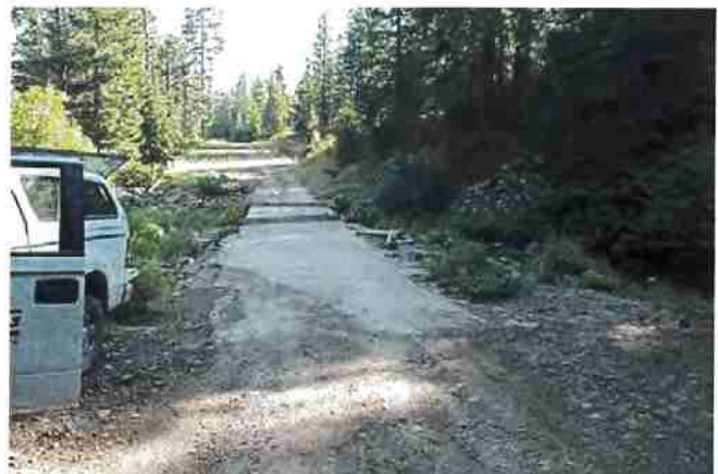
Figure 7. Concreted low-water crossing placed on bedrock outcrop in intermittent stream. Photo: Angela Wilson, Central Valley Regional Water Quality Control Board.
