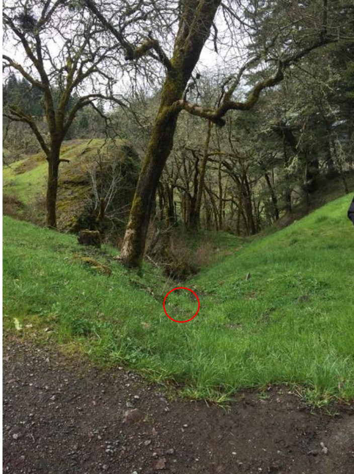
Photo 18. Culvert installation on Road A – location of future outlet marked by red circle
