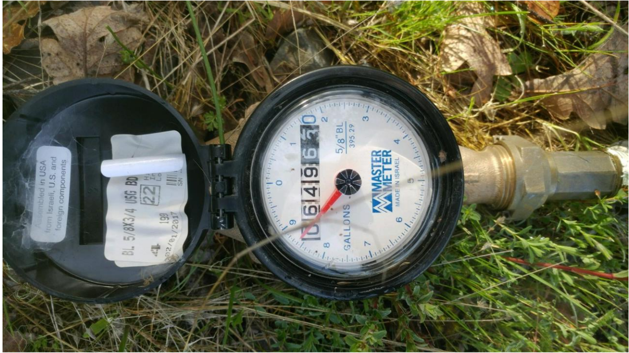
Photo 11. Meter reading – early May
