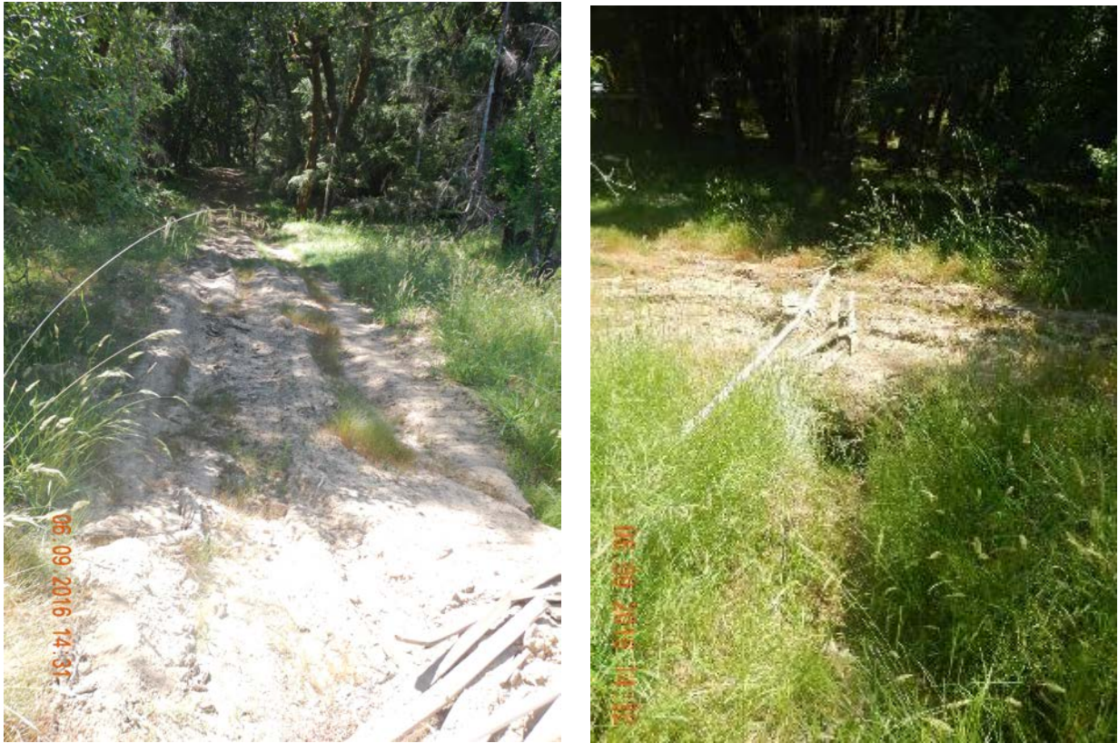
Lower reach of secondary access road. The road fill and 24" culvert has been removed. See Interim Restoration Control Plan for post-removal photographs
