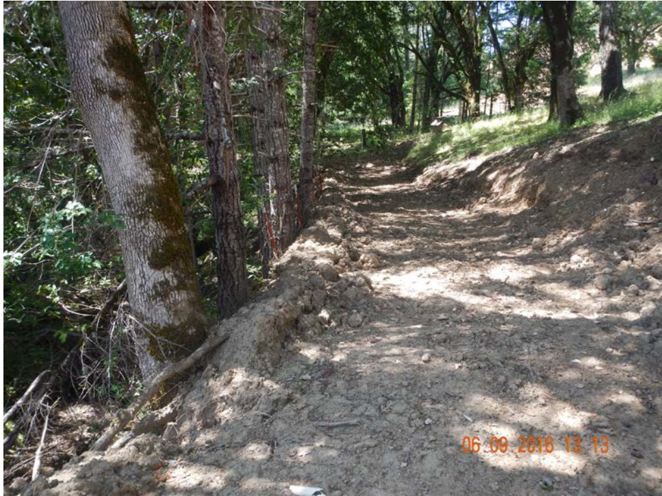
Road graded into hillslope, looking west. The watercourse runs parallel, left of the trees. The perched sediment will be removed by hand.
