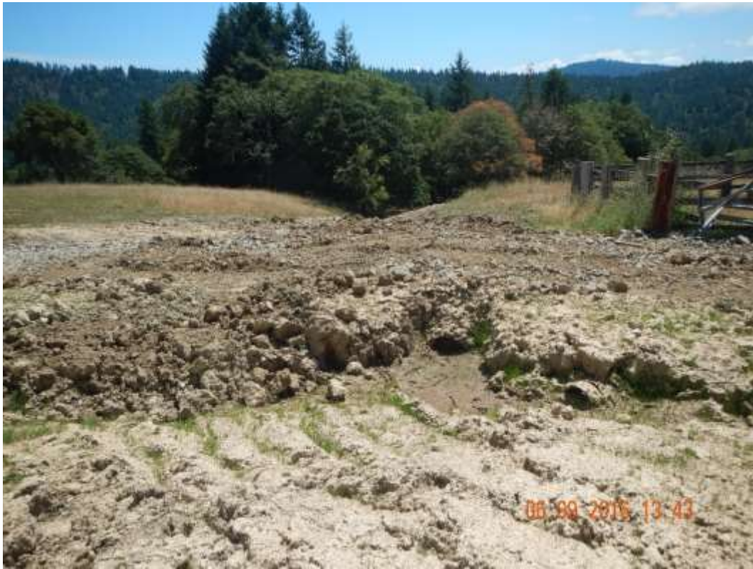
Plugged 24" CMP (center) draining the wet depression area, looking down channel. Pre-restoration.
