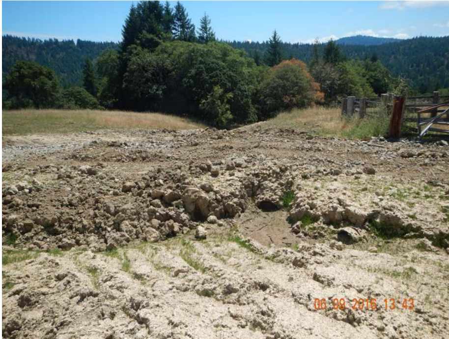
Plugged 24" CMP (center) draining the wet depression area, looking down channel. The culvert has been replaced with an armored rock crossing. See Interim Restoration Control Plan for photographs.
