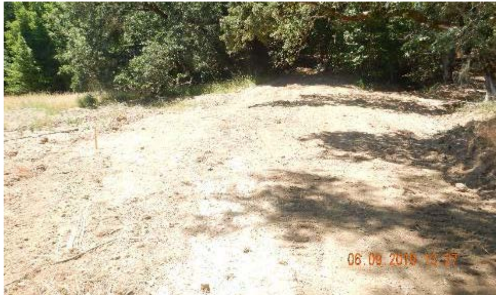
Road grading located east of the stream. The road will be hydrologically disconnected from the stream.
