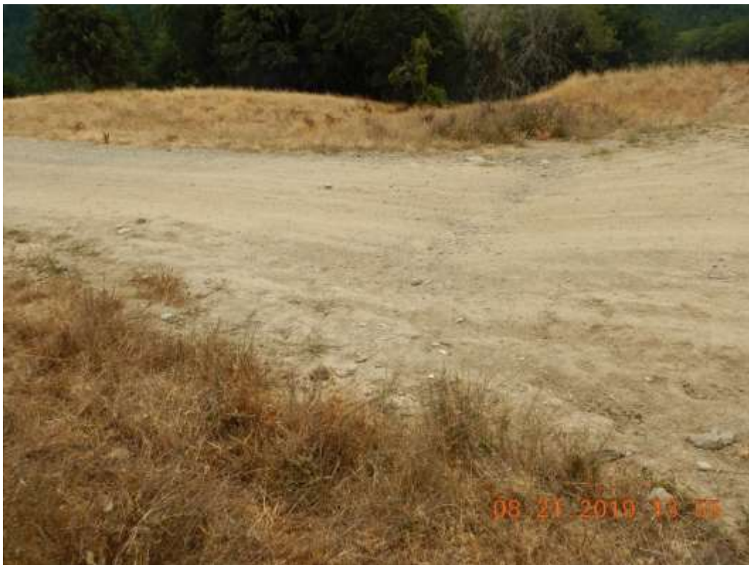
The culvert has been replaced with a rocky crossing. August 21, 2019 – Post restoration
