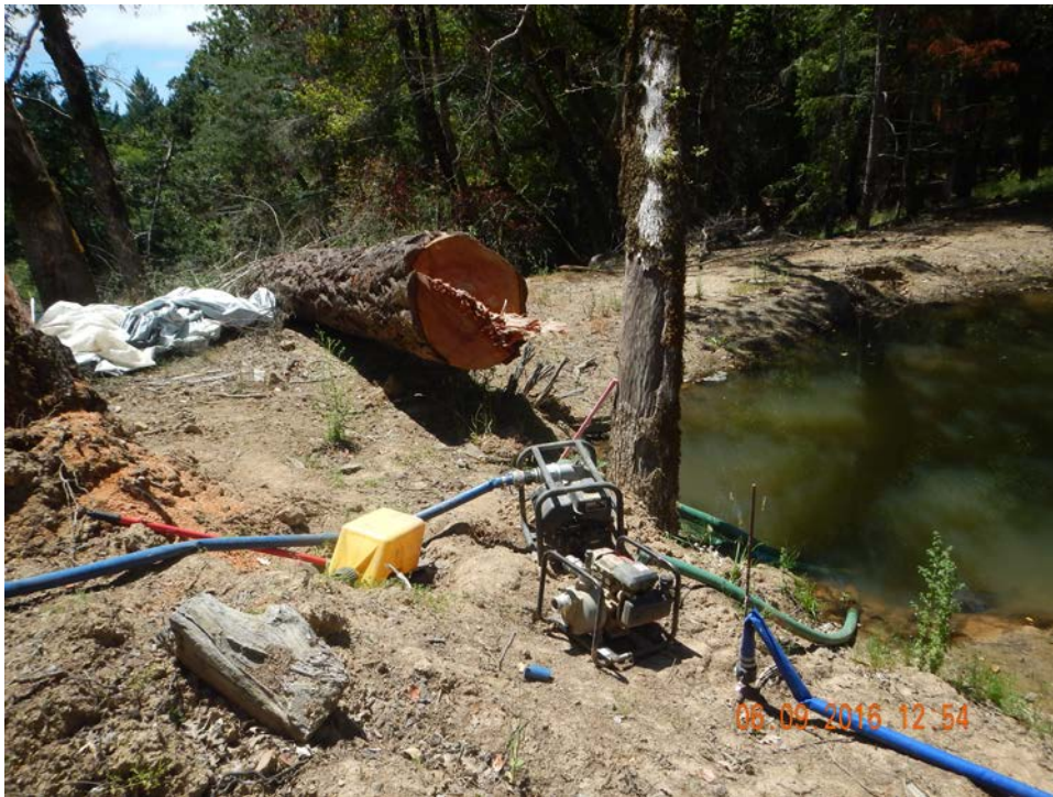
Dam fill in background has been removed. See Interim Restoration Control Plan for post-removal photographs.
