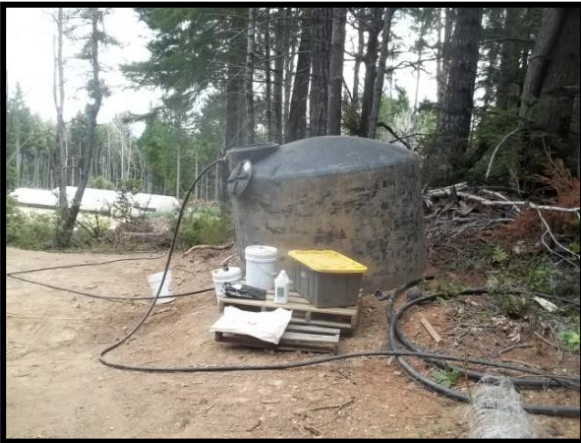
1500 gallon mixing tank
