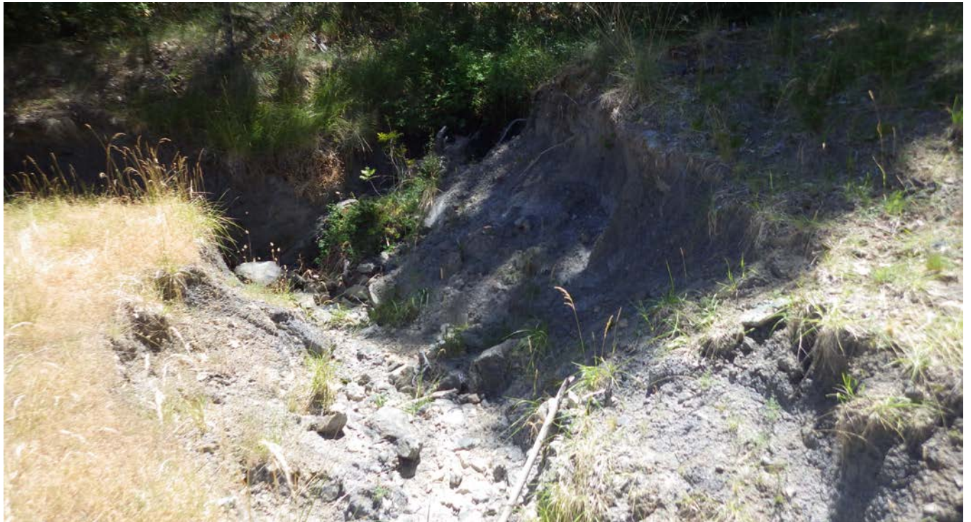
Photo 13 - Area 1 - Bank failure in ditch where conversion occurred for the pond entering a Class III watercourse.
