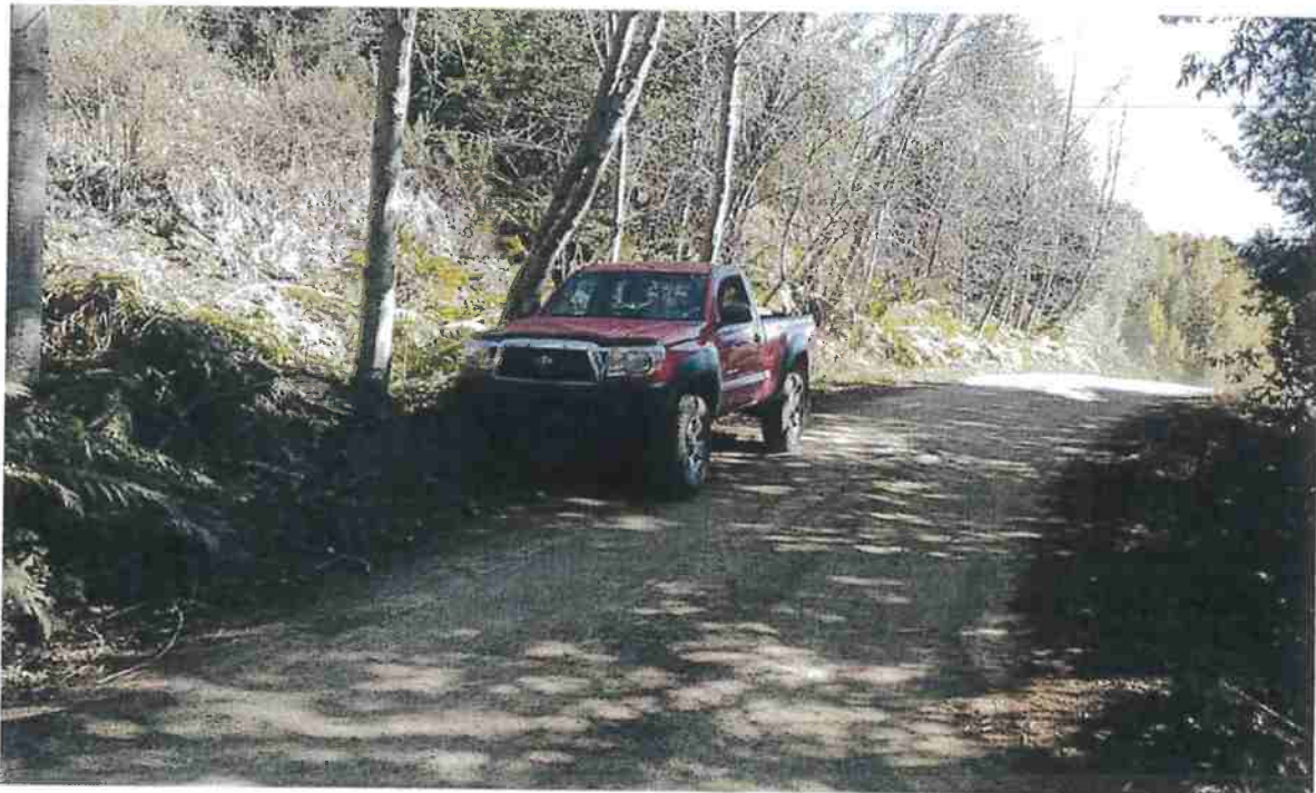
Map Point 6: Existing 18-inch diameter, ditch relief culvert (DRC). The culvert also drains a road side wet area. At Map Point 6 clean out debris and vegetation from the ends of the culvert and keep it open and maintained. The photos show the road surface in both directions is well maintained. Photo date 3-4-2020.
