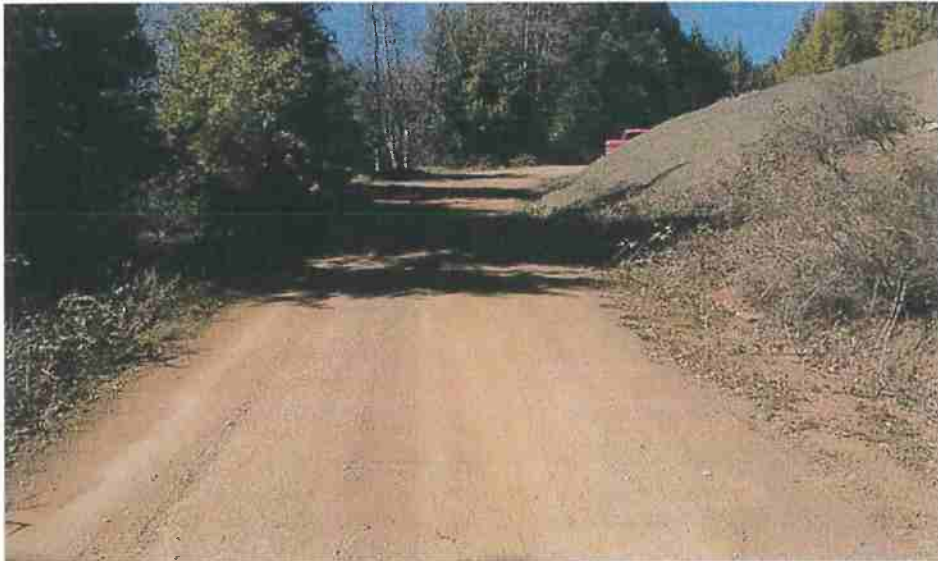
Map Point 3: The upper left shows the outlet, the upper right shows the inlet, and the bottom picture shows the road surface upslope of the culvert. Clean out both ends of the culvert. Above the culvert, grade the outer half of the road surface and outboard shoulder to allow for surface drainage. Photo date 3-4-2020.
