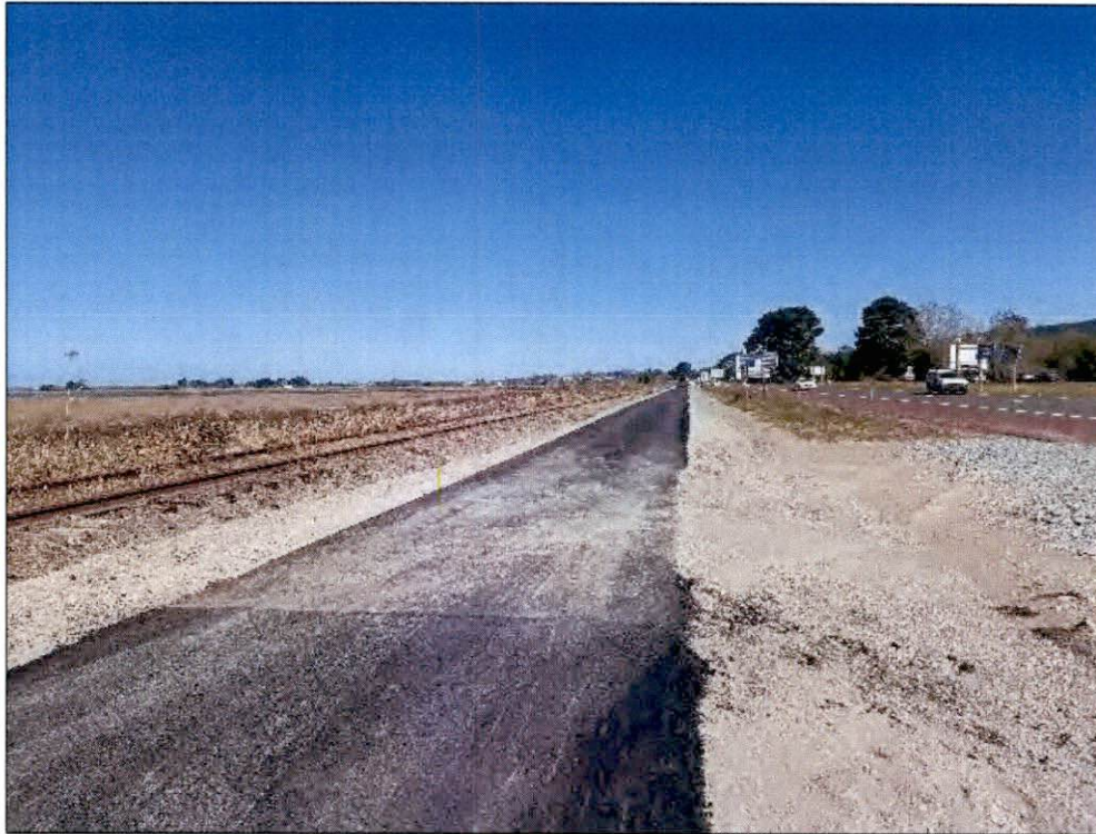
Image 12A. (VAU 10, KOP 12). Existing view of the Humboldt Bay Trail North, which is currently under construction. View facing north.
