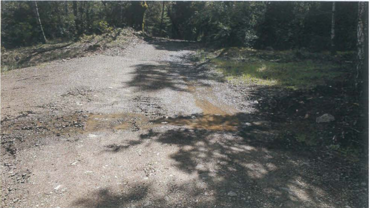
Site 55. Looking south at Site 55. Shows seep flows not being captured by a rocked rolling dip in the foreground.
