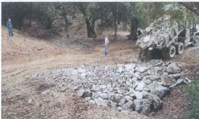
FIGURE 121D. Well graded rock armor is then backfilled into the structure and spread across the breadth of the U-shaped stream crossing, and about one-third the way up the roadbed, so that streamflow will only flow over or come in contact with resistant armor material. The armor must be spread and compacted across the design width of the expected flood flow channel width so peak flows will not flank the armored structure.
