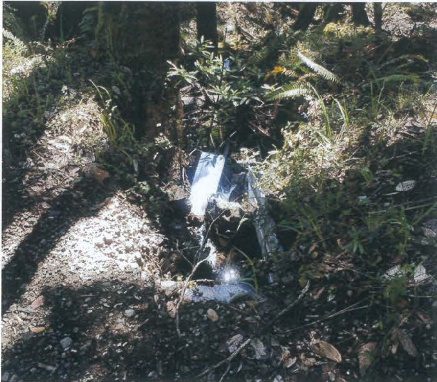
Site 47. Looking at the outlet of the crossing from the road. Note the short culvert and metal sheeting
