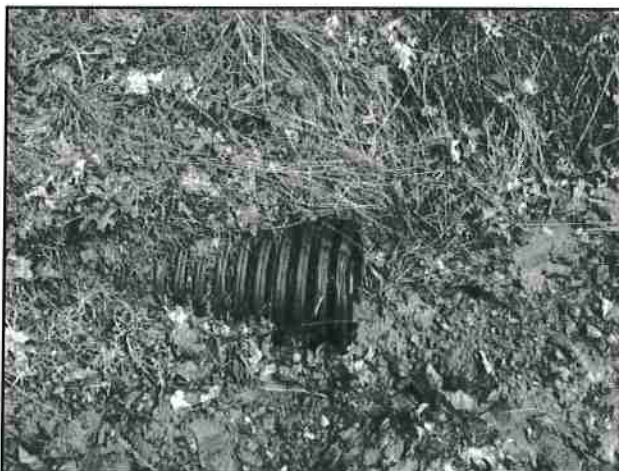
Photo #17 Cobb Rd Looking @ Exposed Culvert
