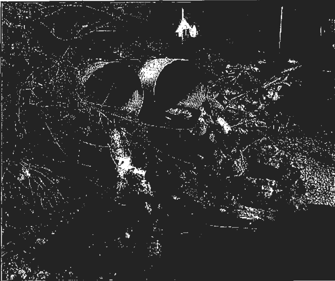
Figure 3. Rock armoring on shotgun culvert outlet. Photo Courtesy of California Department of Transportation (Caltrans).
