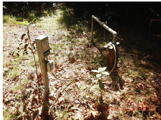
Figure 26. GPS location 461. Well without proper cap.
