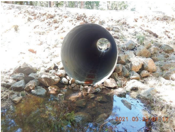
Figure 20. GPS location 455, LSA Crossing 3. Downstream of pond, the stream crossing Culvert was upgraded in ~2018, while enrolled in cannabis general order, without first obtaining authorization for instream work from the Regional Water Board. The inlet is a bit
