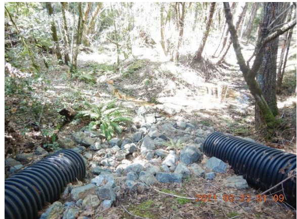
Figure 18. At base of pond berm, outlet pipes drain to watercourse. The LSA included the rock placement.
