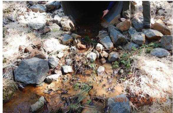
Figure 21. GPS location 455. Outlet of Crossing 3 with evidence of sediment deposits in downstream channel. According to CDFW, the erosion control measures weren't installed at the time of there inspection in December 2020.
