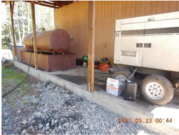
Figure 11. GPS location 447. A large generator powers the three large greenhouses. Indications of numerous small spills, as assessed by HumCo HazMat.
