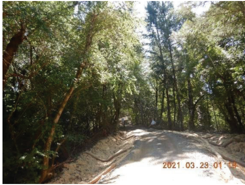
Figure 23. GPS location 455. The road approach to Crossing 3 lacks hydrologic disconnects.
