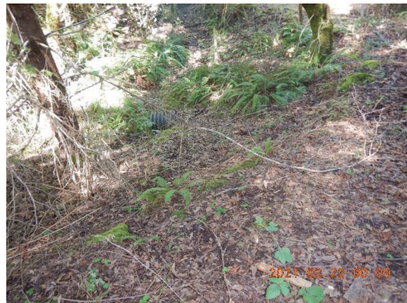
Figure 6. Outlet of culvert at GPS Point 445.
