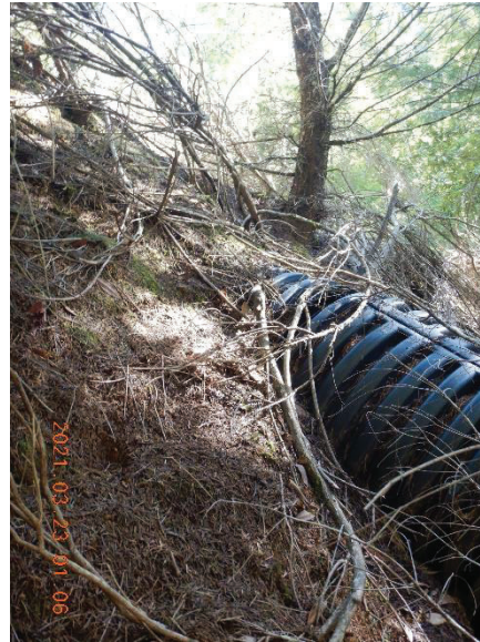
Figure 17. GPS point 454. One of the pond outlet pipes is separated at the 45, near the top of the berm
