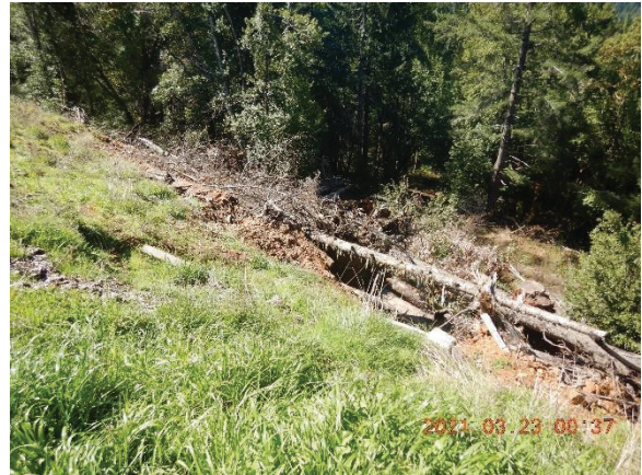
Figure 9. Upper graded flat, near GPS Point 447, slash at toe of fill slope.
