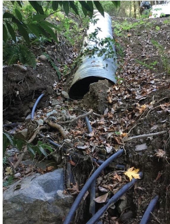
Figure 25. Photo of Crossing 1, by Ryan Bourque of CDFW taken on December 7, 2020 inspection. Photo shows lack of erosion control and erosion and sediment transport to the watercourse at the outlet of the downspout.
