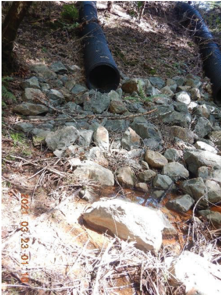
Figure 19. The separated pipe was not flowing water but I observed water between the rip rap at the outlet, indicating seepage at pipe separation or berm seepage.
