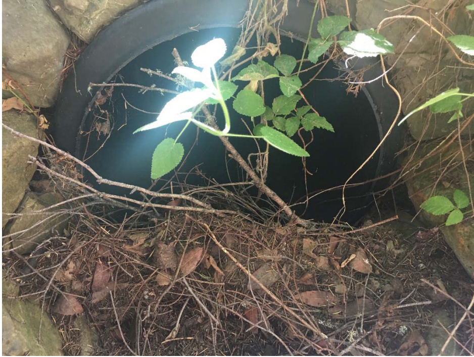
Figure 11. Culvert Inlet Debris 3/12/2020
