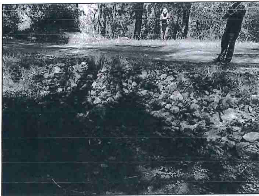
Photo 3 – Project #2, View looking downstream at the stream crossing culvert inlet and armored inboard fillslope.
