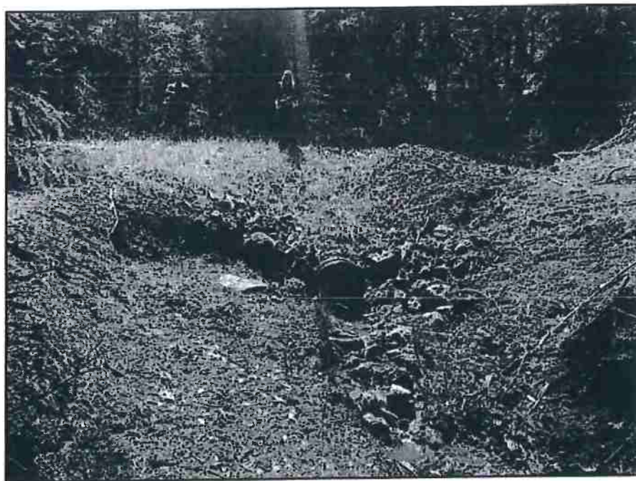
Photo 4 – Project #2, View looking upstream at the stream crossing culvert outlet and armored outboard fillslope:
