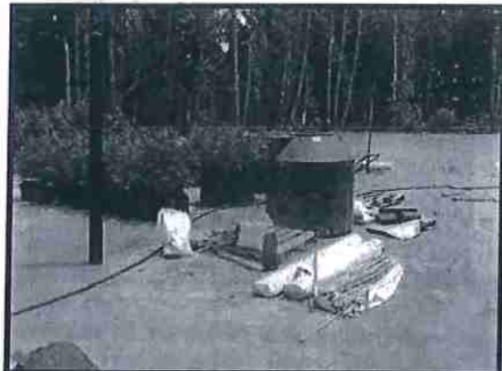
305 gallon mixing tank
