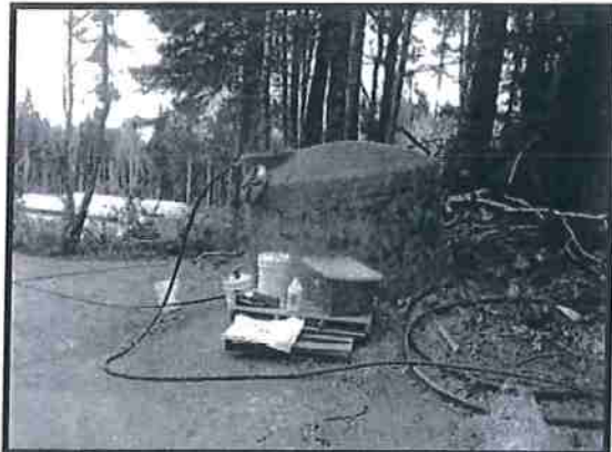
1500 gallon mixing tank
