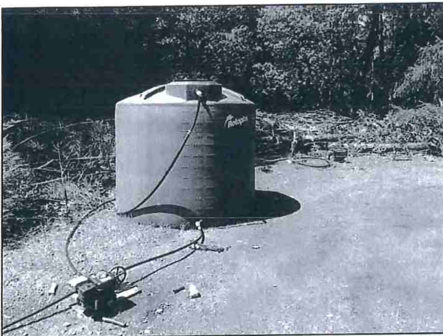
Photo 12 – View the 2,500 gallon water tank next to Well #2 that provides water storage for a neighboring parcel.
