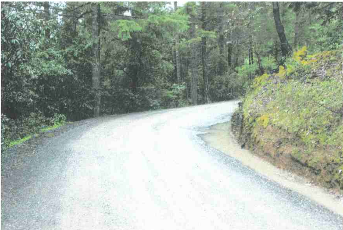
Photo 6. Mile 1.6: Pinch Point 3 (first pinch point on gravel segment), blind corner, 16-ft road surface + 1-ft shoulders.
