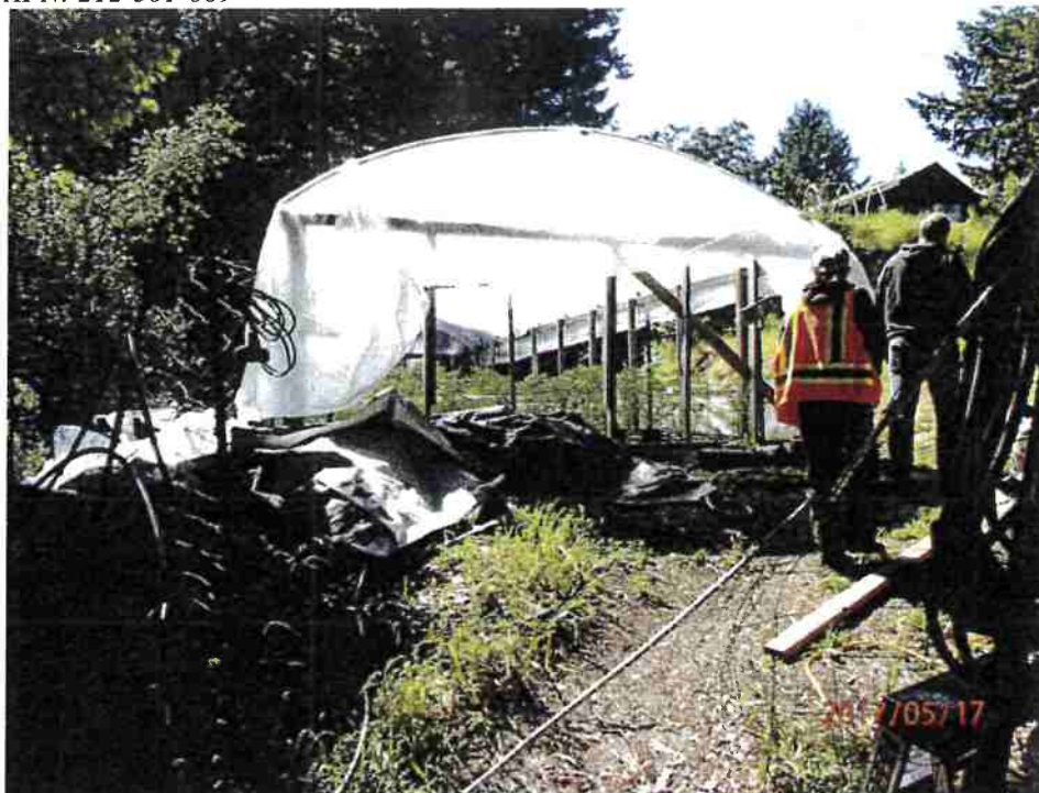
Photo 9- View of Greenhouse #1, which gets its water from the concrete cistern.
