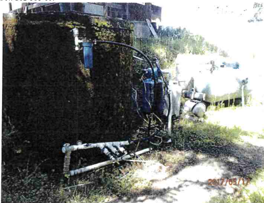
Photo 5- View of the concrete cistern that is used for domestic and cultivation purposes.
