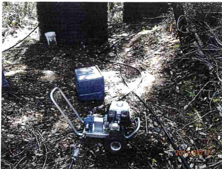
Photo 4- View of the water pump that directs the gravity fed water from tanks to cistern by house
