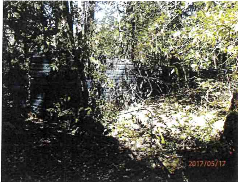
Photo 3- View of the five 2,825 gallon water storage tanks
