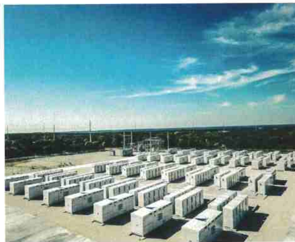
Photo 2: Aerial view of a typical BESS Project site.
