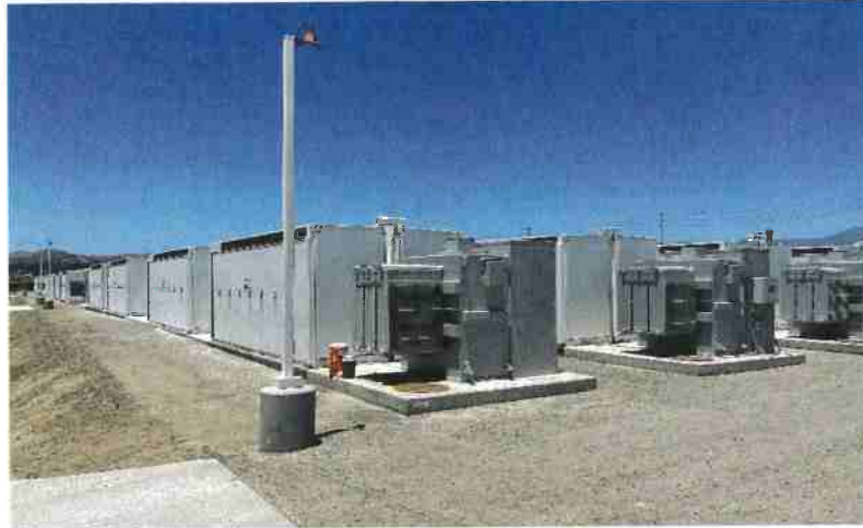
Photo 1: Overview of a typical Battery Energy Storage System (BESS) containers.
