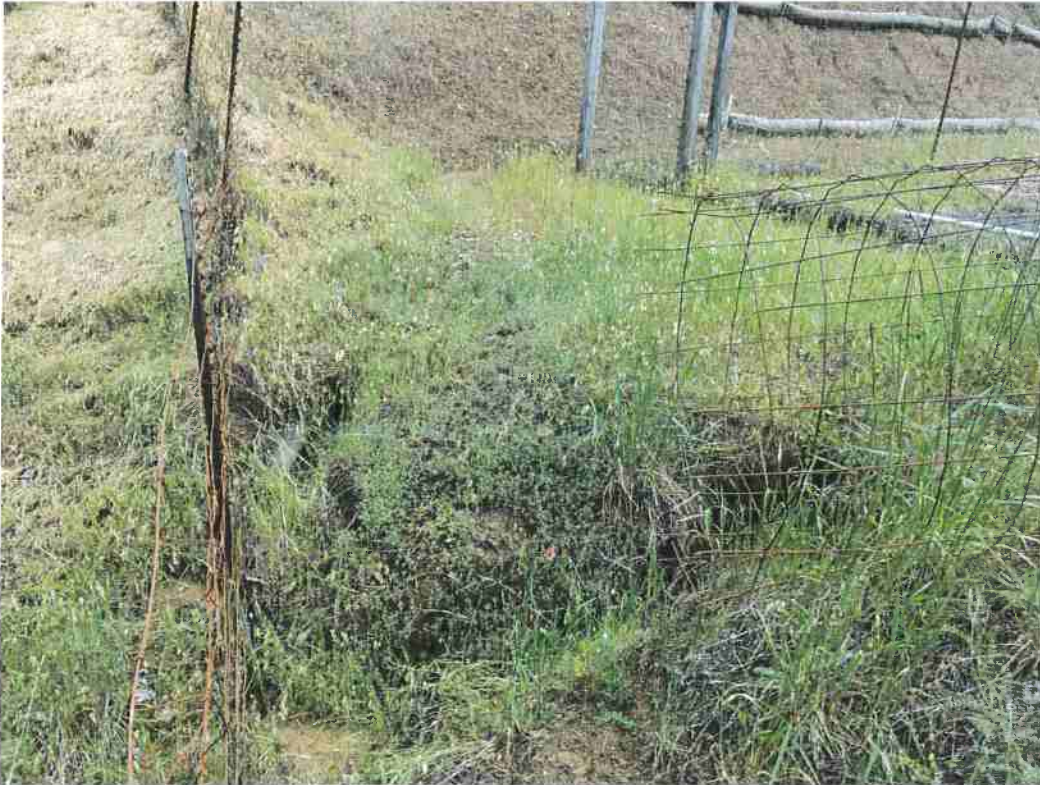
Photo 4. Site A; north edge looking at two small knick-point erosion features (Recommendation #1). Fill erosion features and armor edge of fill slope with 4" diameter rock.
