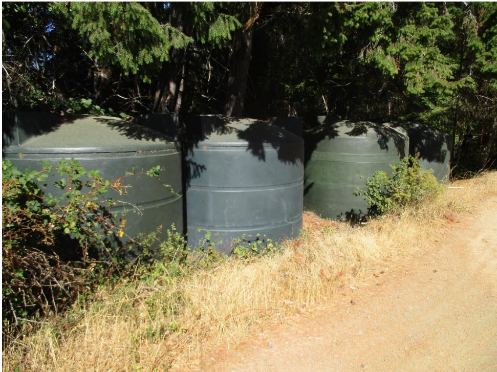
Water Storage Tanks (2016)
