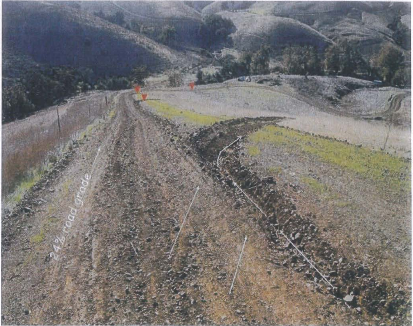
FIGURE 55. Steep roads that go straight up or down a hillside are very difficult to drain. This steep, fall line road developed a through cut cross section that was drained using lead out ditches to direct runoff off the road and onto the adjacent, vegetated hillside. The road was "outsloped" to drain runoff to the right side, and the lead out ditch was built slightly steeper than the road grade, to be self-cleaning. Four lead out ditches have been constructed at 100-foot intervals to the bottom of the hillside.
