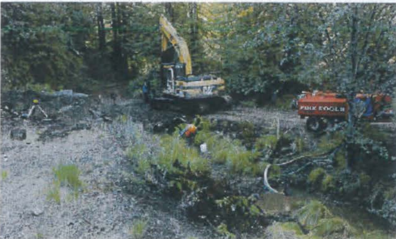
FIGURE 199. For larger streams, pump trucks, large pumps or multiple small pumps can be used to pump streamflow around project work sites. Here, a pump truck is used to temporarily divert flow in a fish bearing stream where dual culverts are being replaced with a raker bridge. Young fish were removed from this fish bearing stream before project work started.
