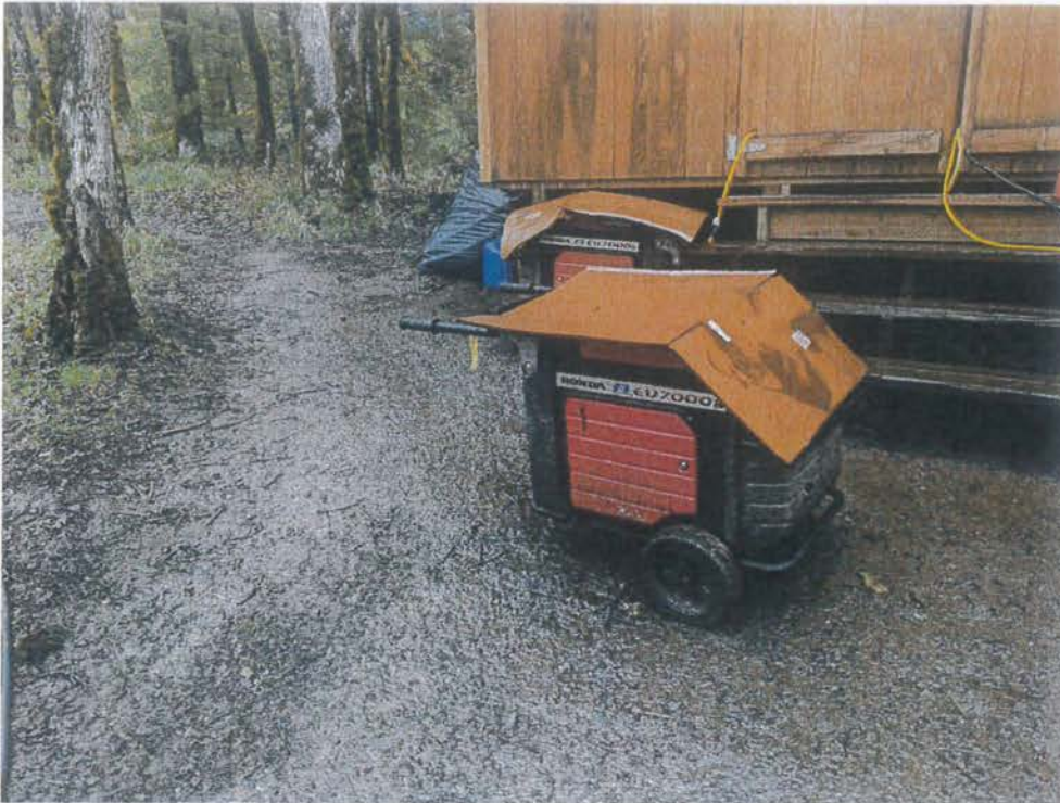
Improper storage of generators.
