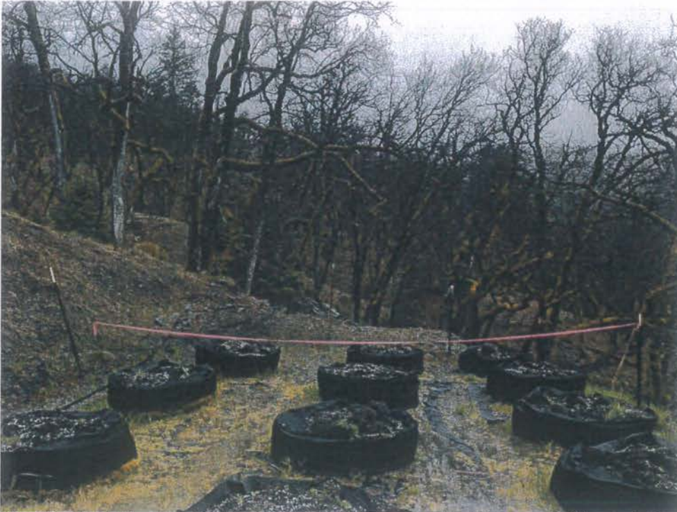
Site 20 at Cultivation Area D where five pots shall be removed and the area shall be seeded and straw mulched.
