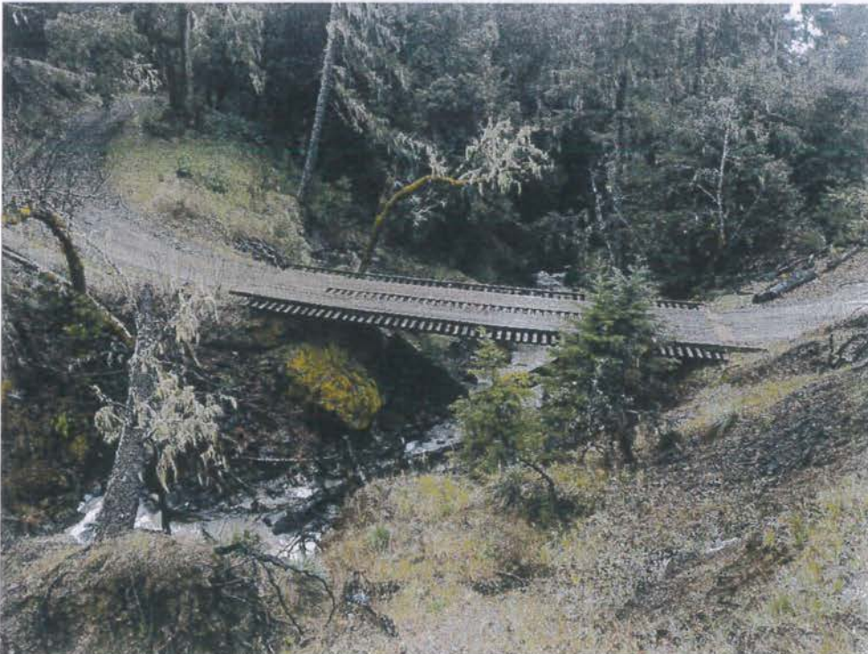
Looking down at Site 06 where both approaches to the bridge require additional rock surfacing.
