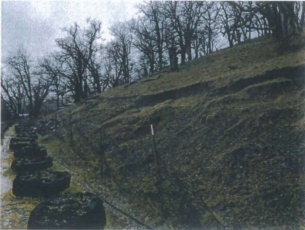
Site 19 with the cutbank failure.
