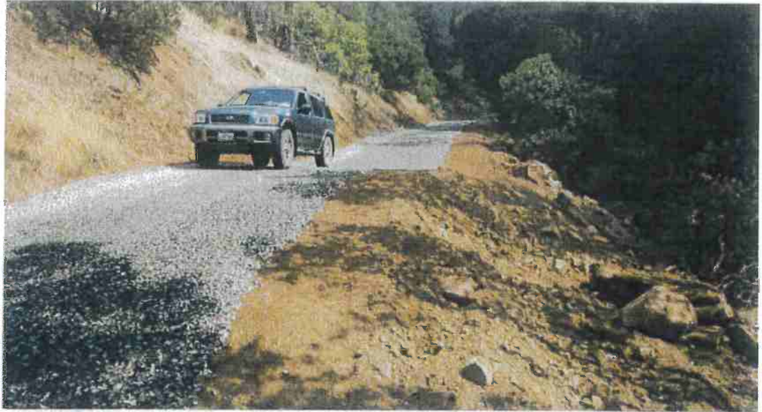
FIGURE 33A. Rolling dip constructed on a rock surfaced rural road. The rolling dip represents a change-in-grade along the road alignment and acts to discharge water that has collected on, or is flowing down, the road surface. This road was recently converted from a high maintenance, insloped, ditched road to a low maintenance, outsloped road with rolling dips.
