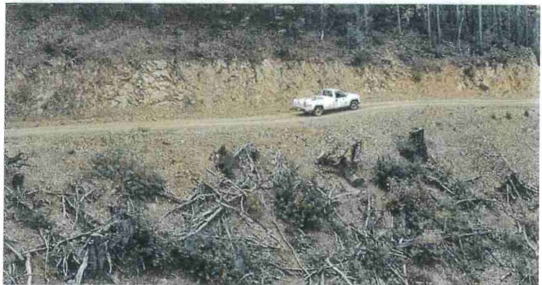
FIGURE 33B. This side view of an outsloped road shows that the rolling dip does not have to be deep or abrupt to reverse road grade and effectively drain the road surface. This outsloped forest road has rolling dips that allow all traffic types to travel the route without changing speed.
