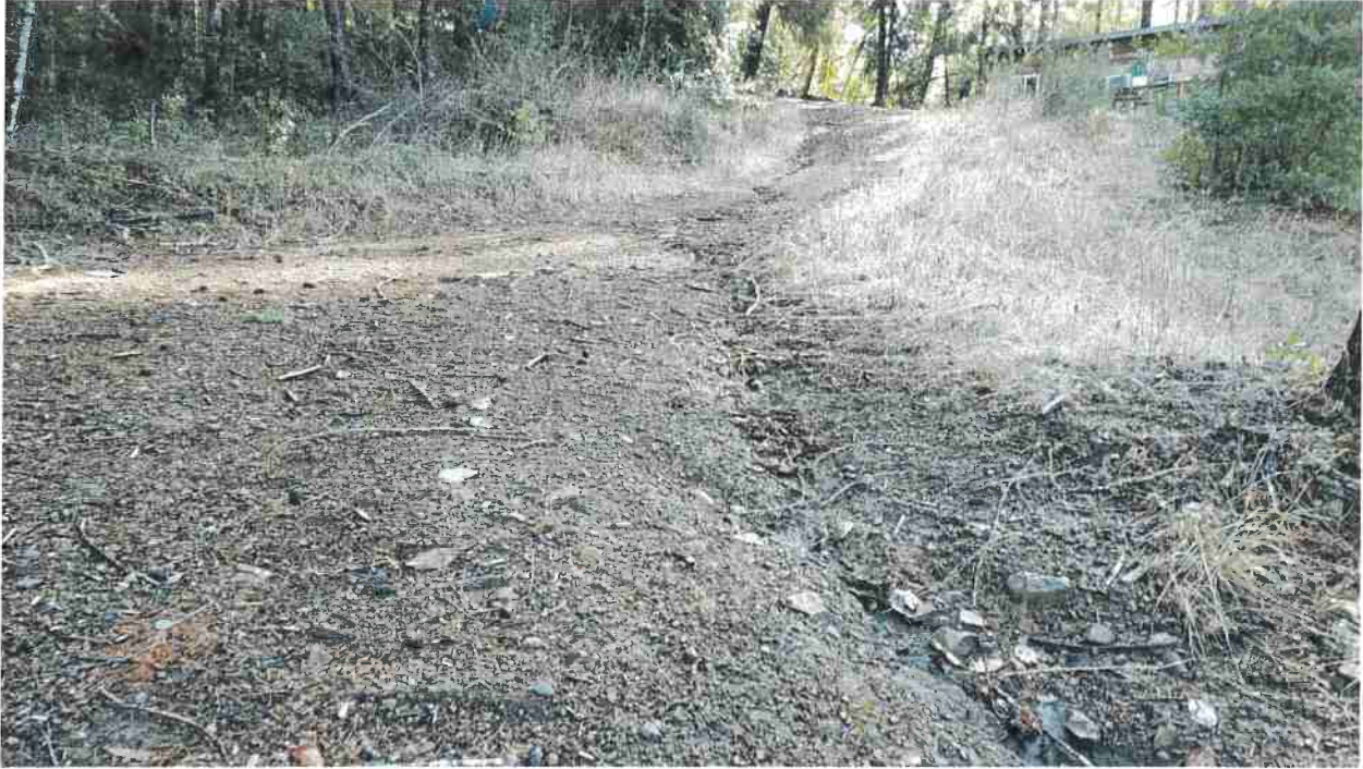
Photo looking up grade at concentrated road surface runoff that is coming from Site 04 and is draining into surface cracks at Site 06.
