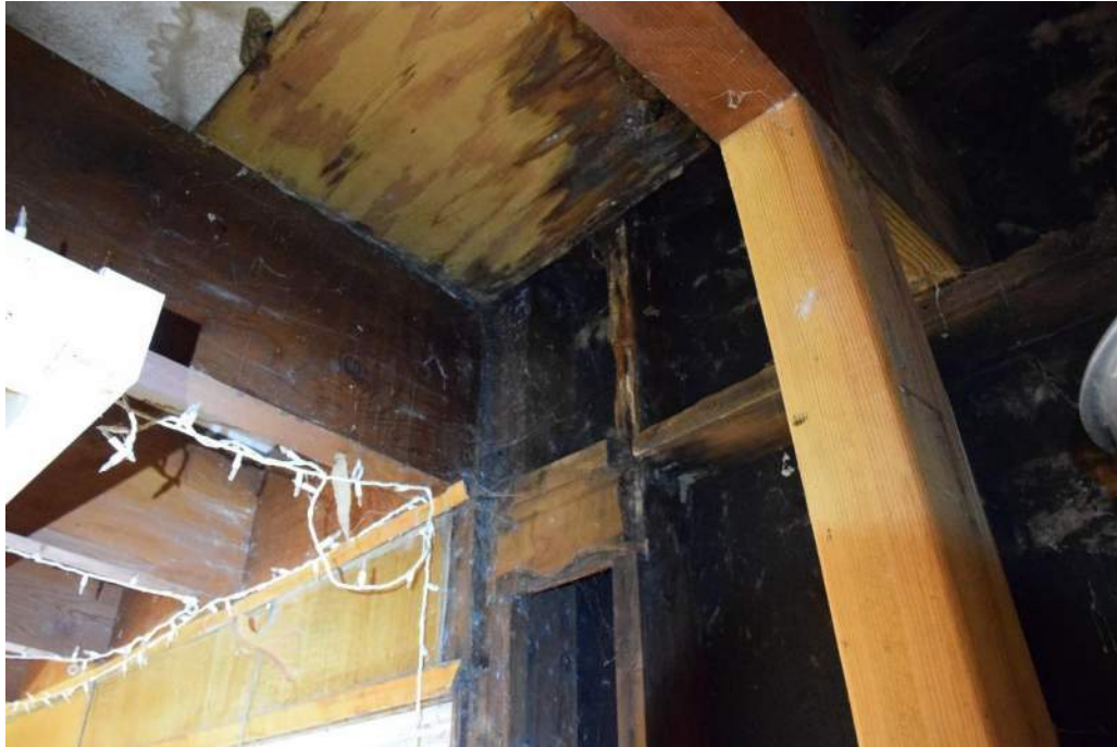
Figure 3 – Damaged beam, wall studs, and support ledger in the Auditorium
