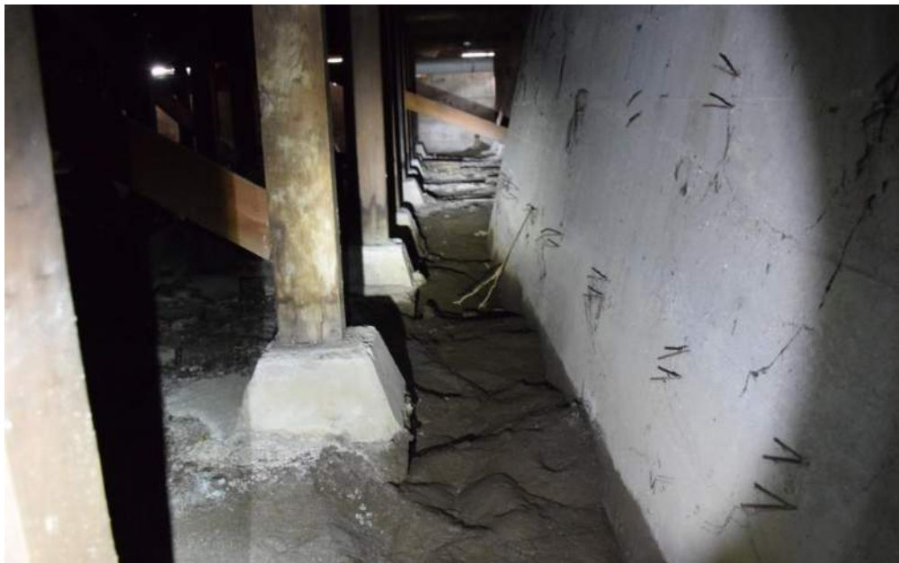
Figure 5A – Erosion of soil at isolated footings near west perimeter wall
