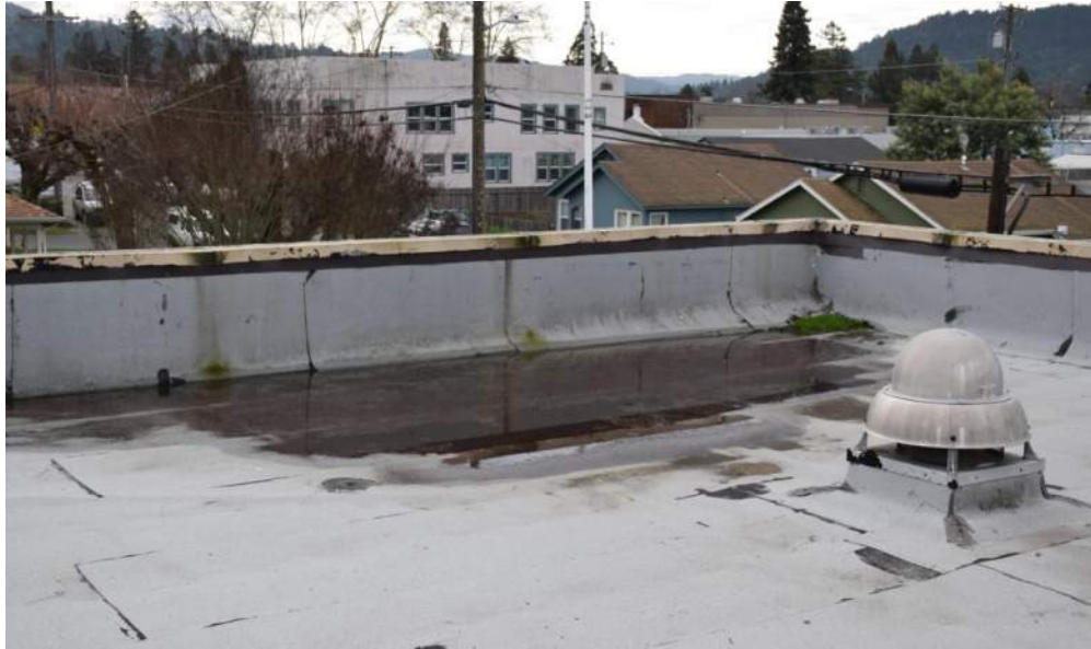
Figure 4 – Ponding at roof above spectator lounge
