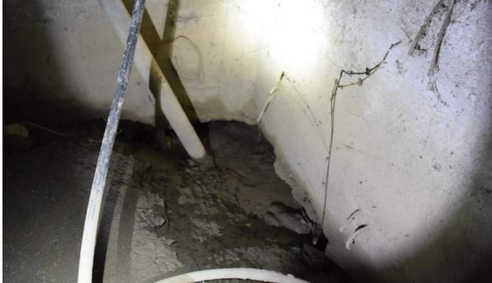
Figure 5B – Scour under northwest corner of perimeter foundation wall
