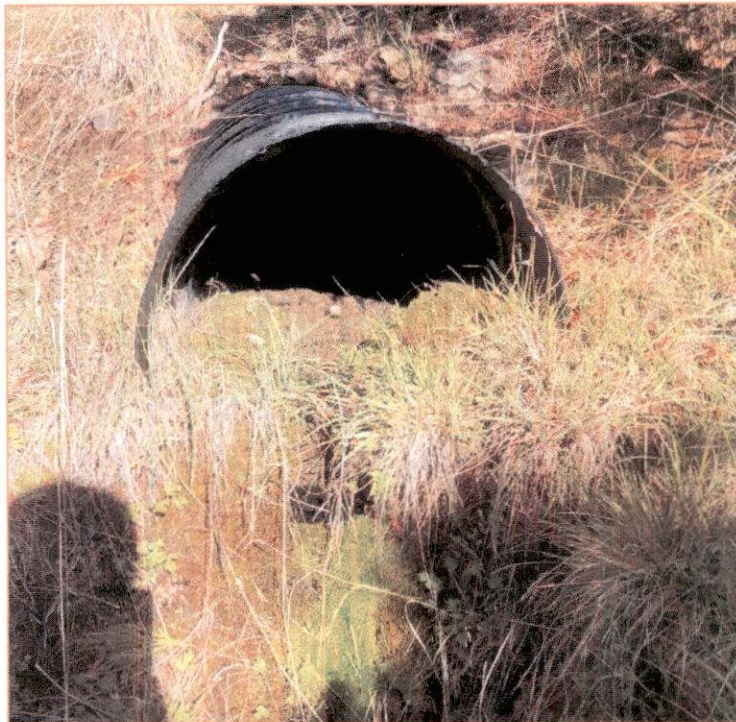
RP9) Clean and maintain DRC outlet.
