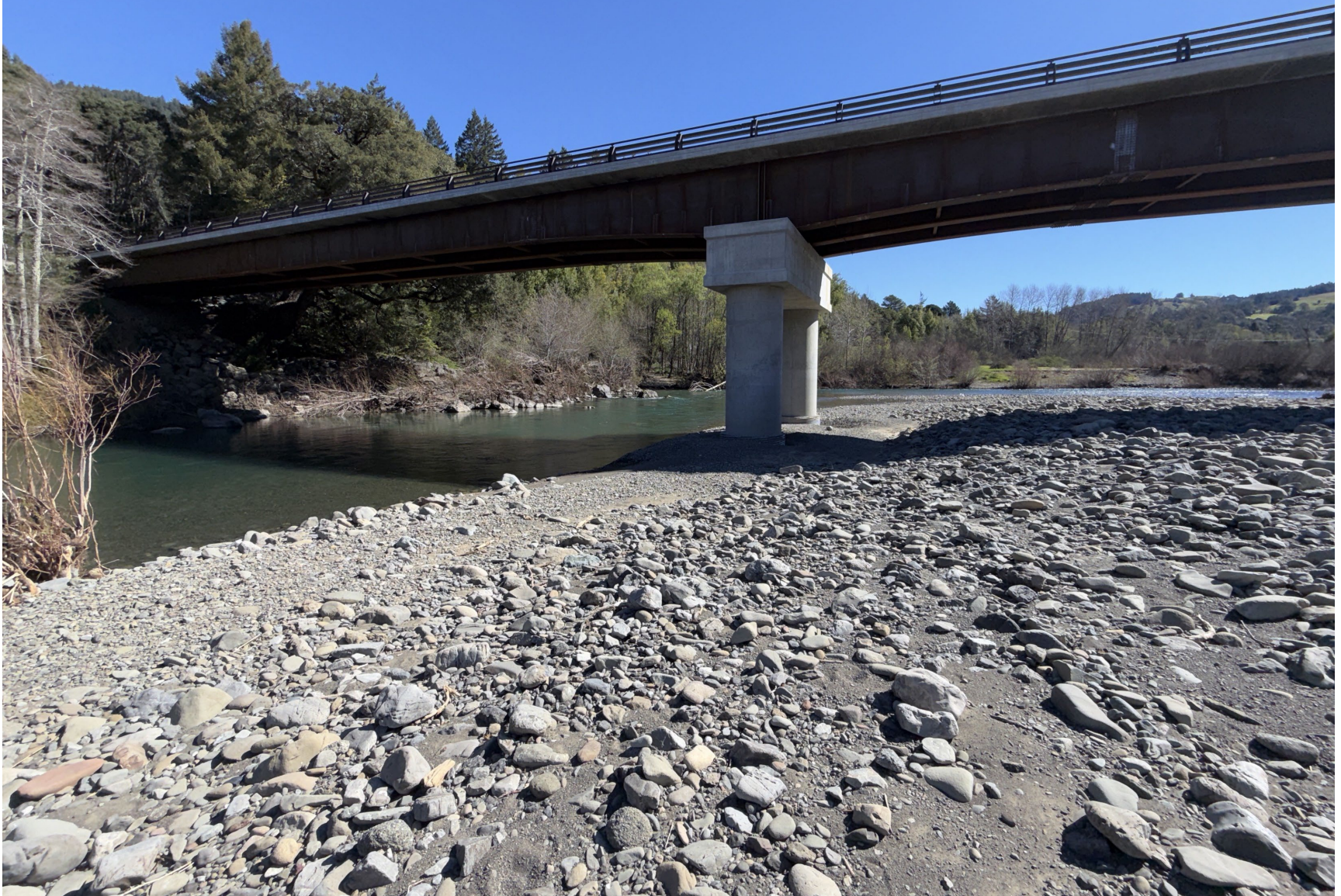
View facing northeast (upstream) of the new bridge over the Mattole River at Honeydew (March 2026)
