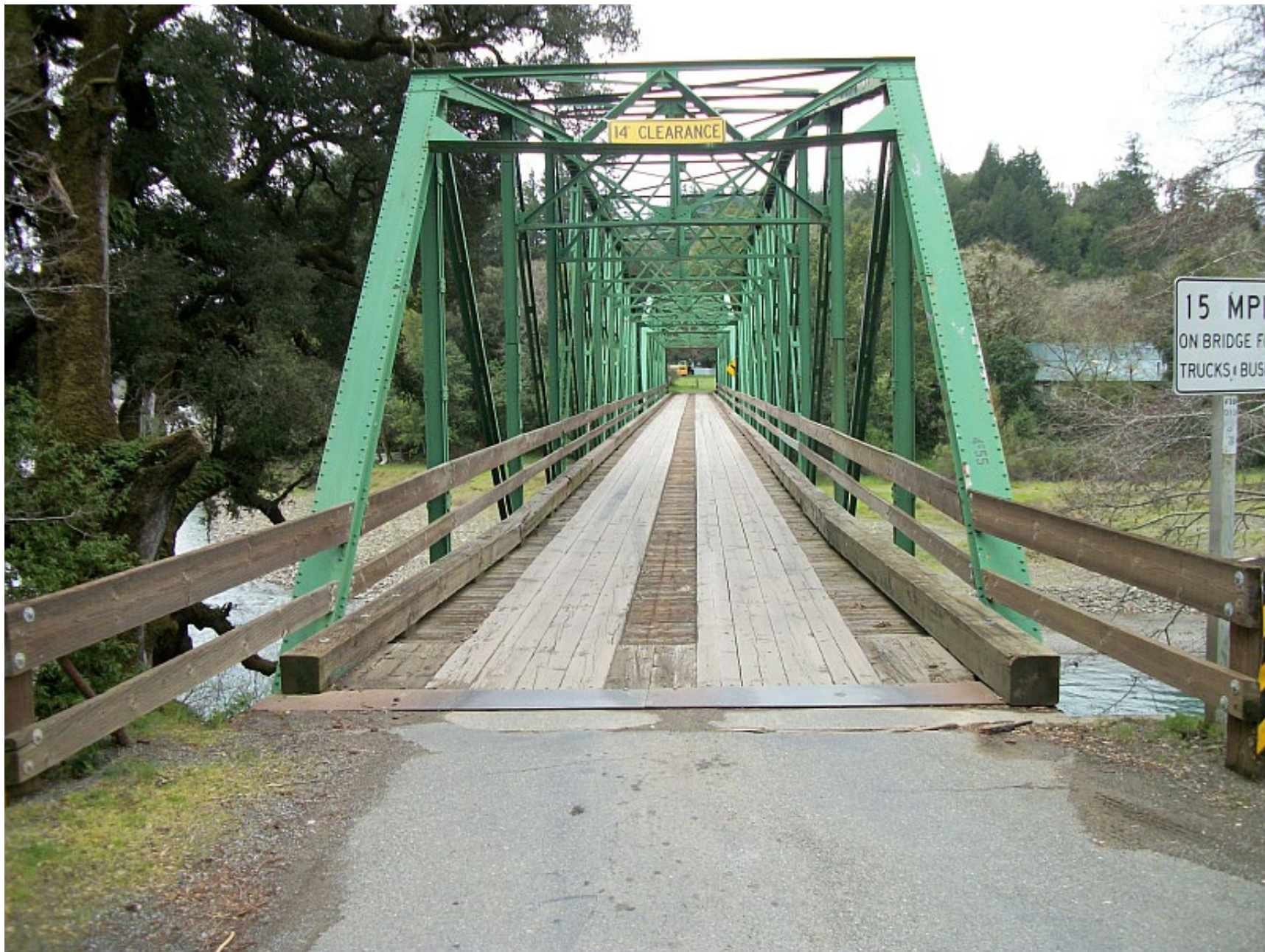
North side of the former bridge over the Mattole River at Honeydew (February 2012)
