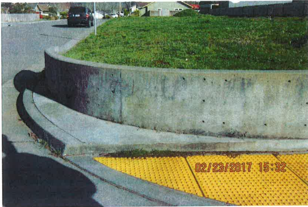
Above: Curb return requires retrofit to full intersection ramp.
