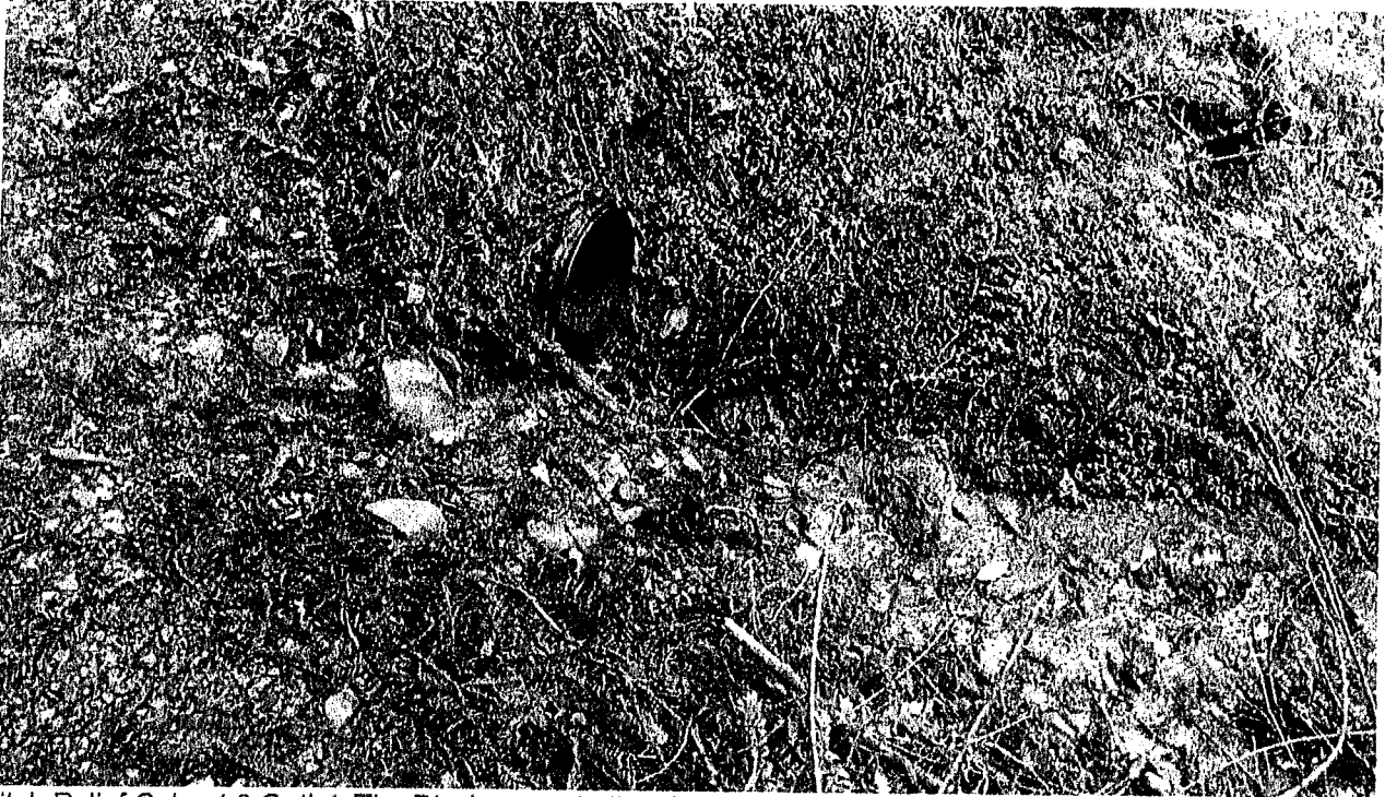
Ditch Relief Culvert 3 Outlet: The Discharger shall rock armor the outlet of this ditch relief culvert per attached specifications.
