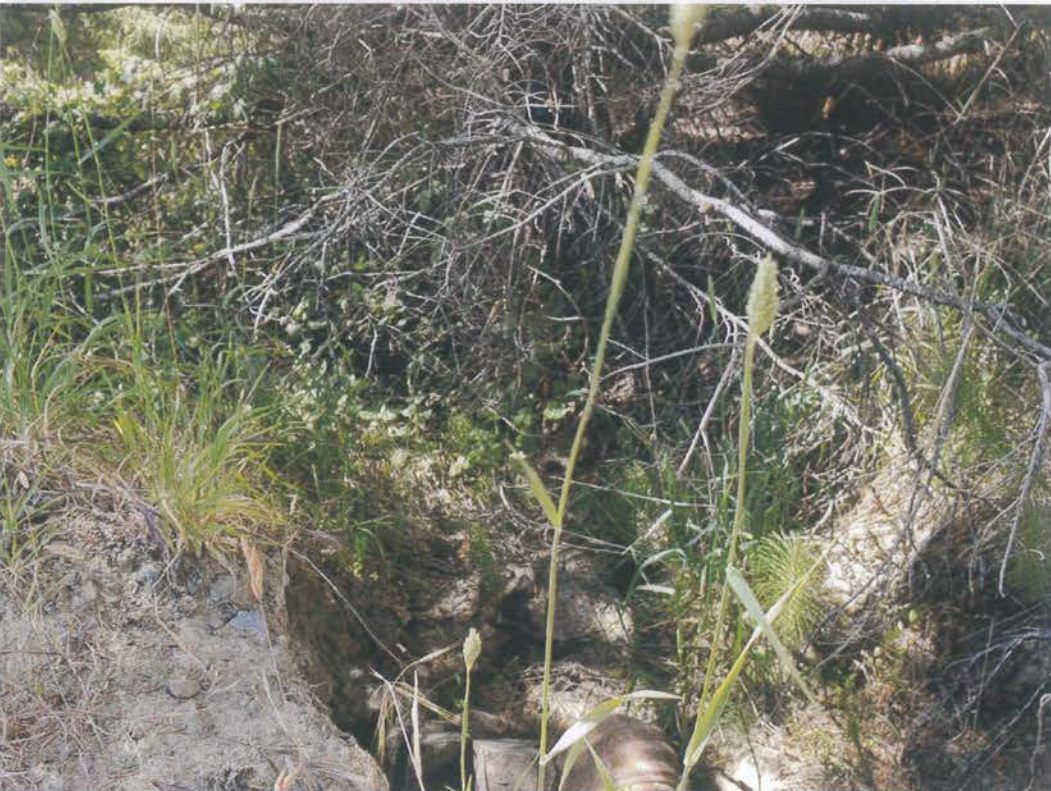
Site 07. Looking down-channel from the outlet. The upgraded culvert will outlet approximately in the brush to the upper center of the photo.
