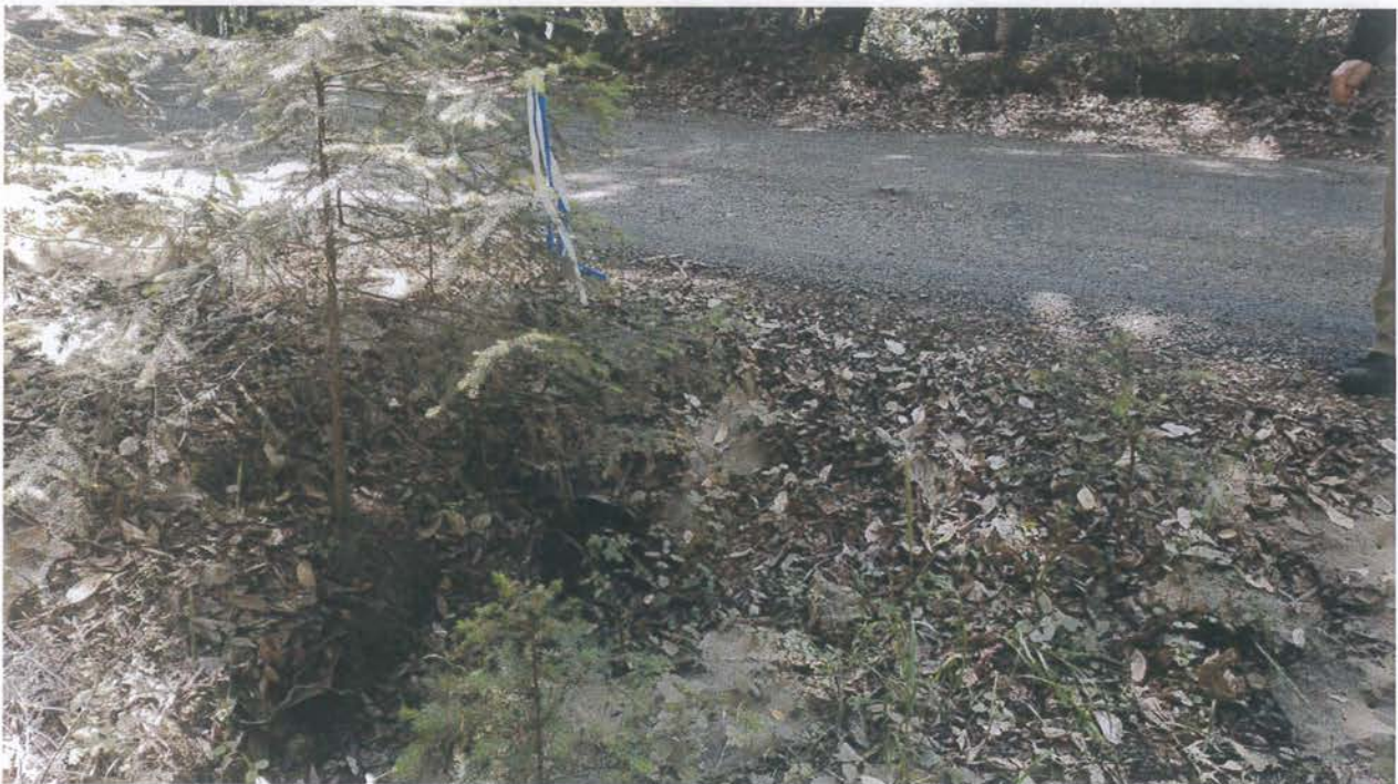
Site 24. Inlet of the watercourse crossing.
