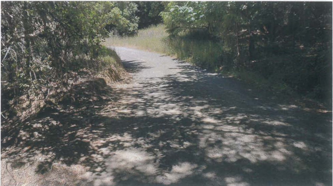
Site 13. Looking up grade at Site 13. A Class III watercourse is diverted down the inside ditch to the right. Re-alignment of this watercourse will consist of a culvert installed diagonally across the road from the grass patch in the upper center-right to the lower left of the photo.
