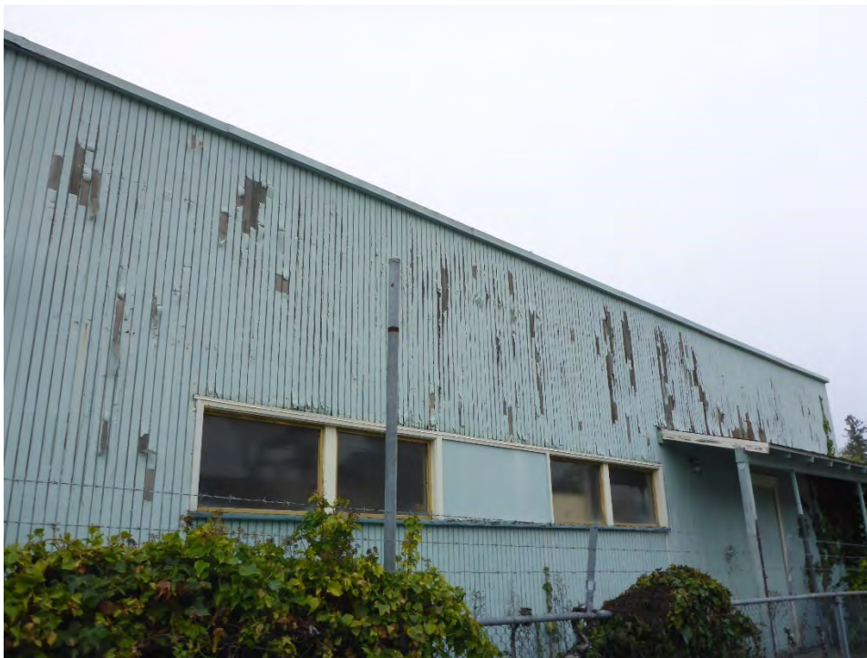
Photo #25: Exterior paint has reached the end of its useful life.
