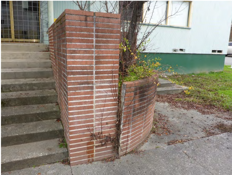
Photo #39: Planter Is Cracked and Is Failing.
