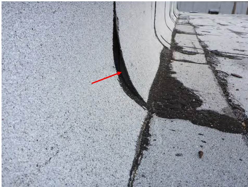
Photo #15: Roofing laps are not sealed.
