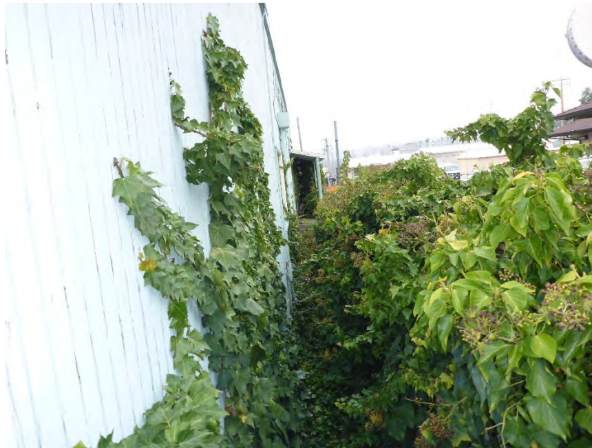
Photo #34: Ivey has grown onto exterior walls.
