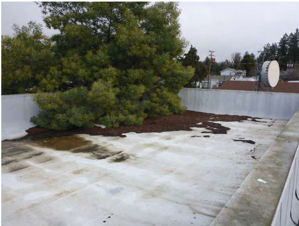
Photo #36: Adjacent tree is growing under foundation and is dispersing debris on to roof. This condition allows the drains to become clogged.
