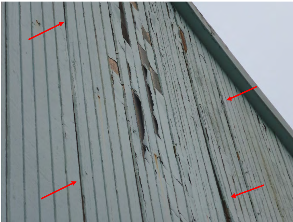
Photo #27: Exterior siding is warped.
