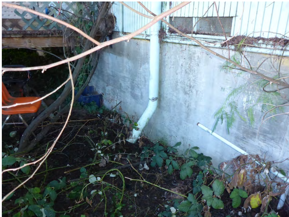
Photo #38: Roof downspout does not drain to street.
