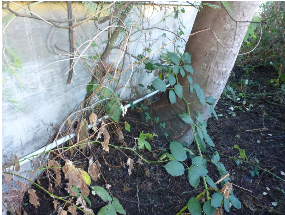
Photo #37: Adjacent tree is growing under foundation and is dispersing debris on to roof.
