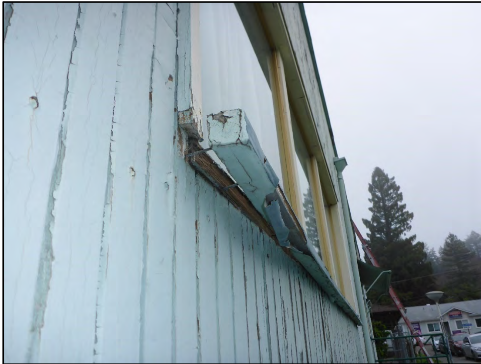
Photo #30: Exterior trim is decayed and is failing
