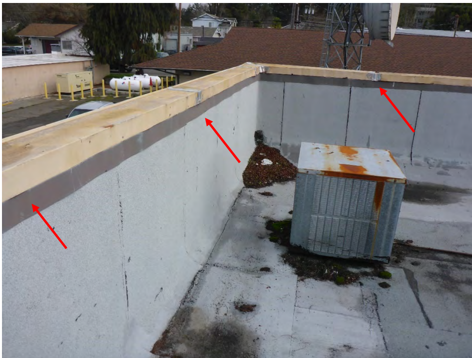
Photo #13: Roof coping caps have unsealed joints. Sheetmetal extension tucked up under coping cap in efforts to terminate re-roof. The termination is improper. It doesn't seal water infiltration through coping cap joints.
