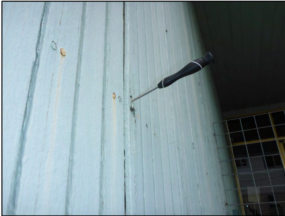
Photo #28: Exterior wall panels are decayed
