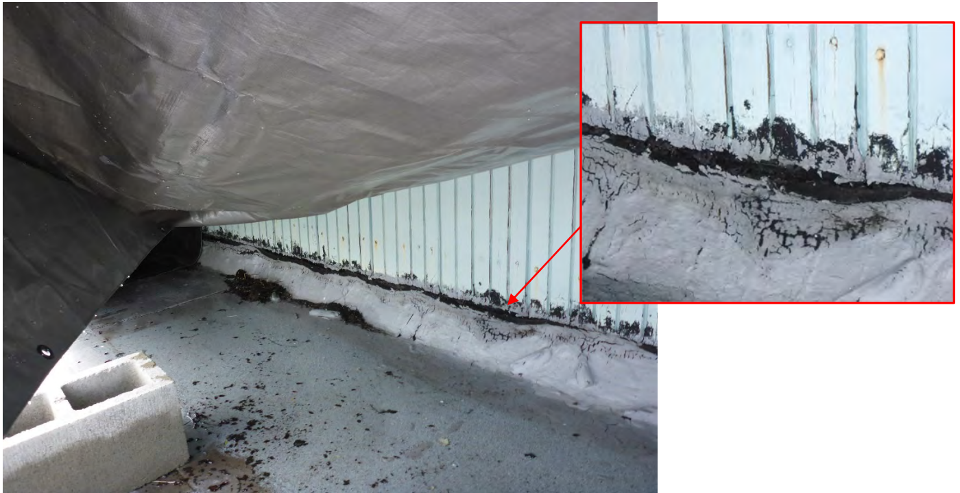
Photo #10: Roof base flashings are improper and or are missing. Roof is not flashed up under wall siding.
