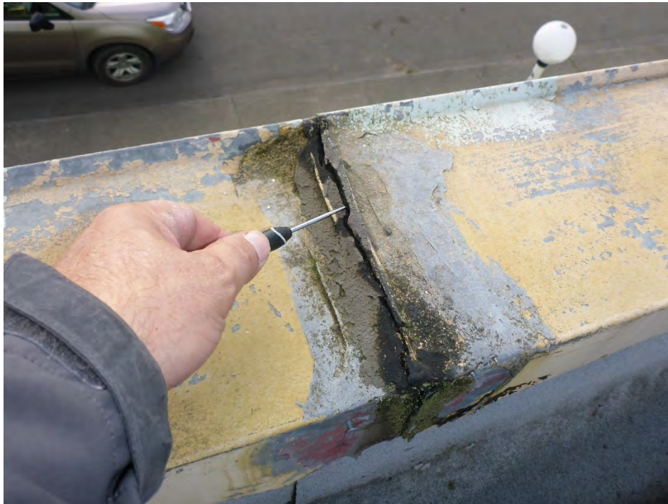
Photo #12: Roof coping caps have unsealed joints.
