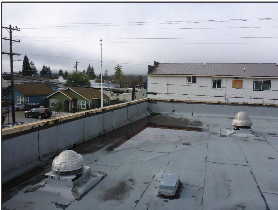
Photo #9: Roof lacks proper slope to drain. Standing water.
