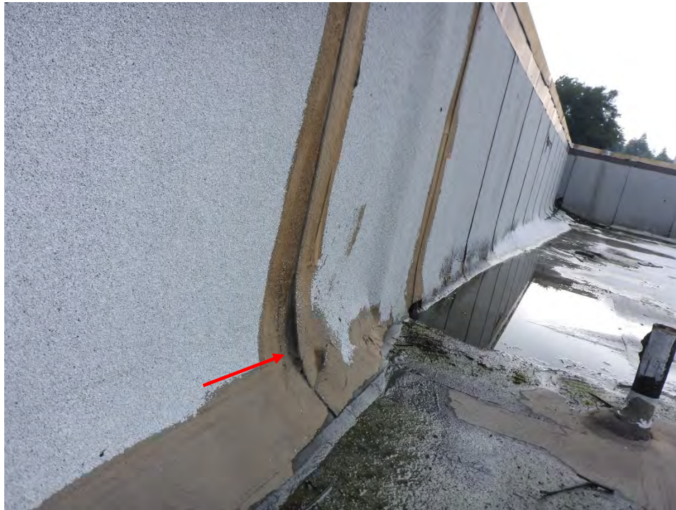
Photo #14: Roofing laps are not sealed. Open voids.
