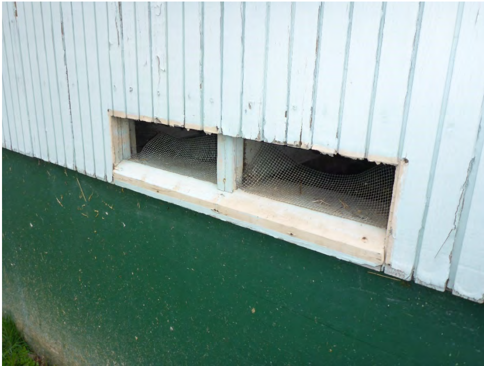
Photo #32: Foundation vents are damaged and are open
