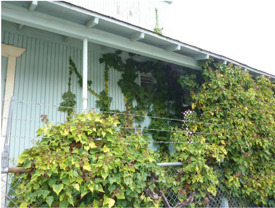
Photo #35: Ivey has grown onto exterior walls.
