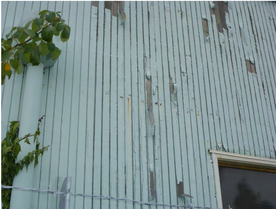
Photo #26: Exterior paint has reached the end of its useful life.
