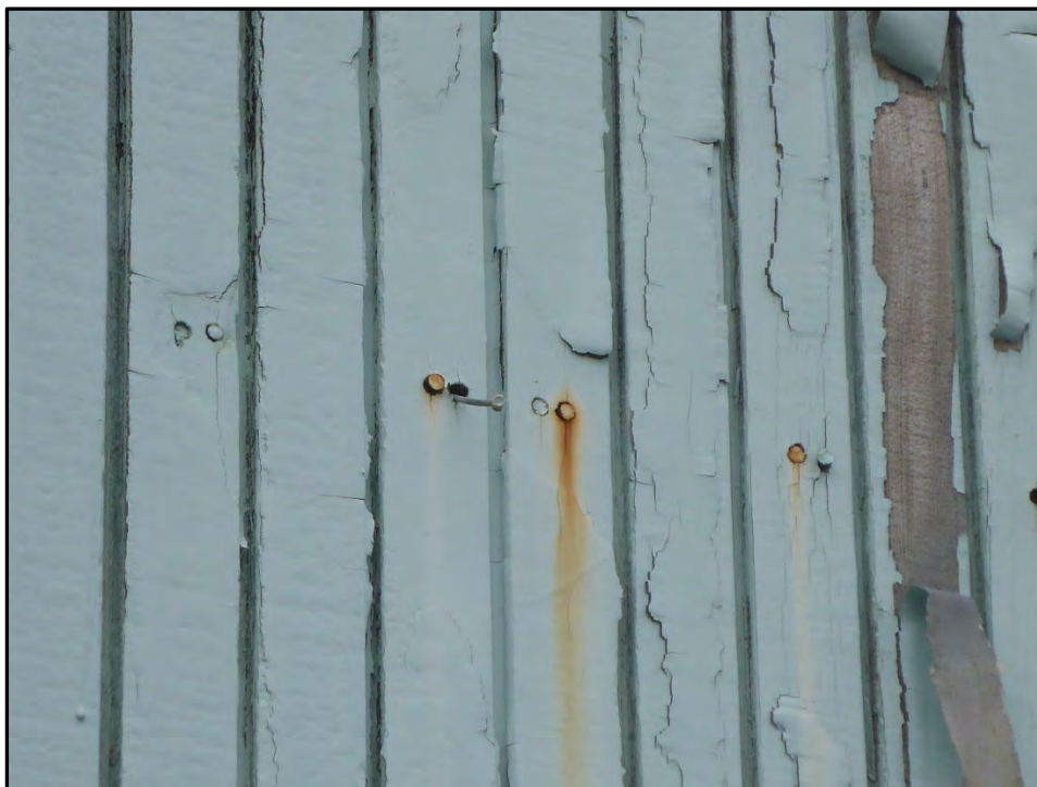
Photo #29: Exterior wall siding fasteners are rusting and are backing out
