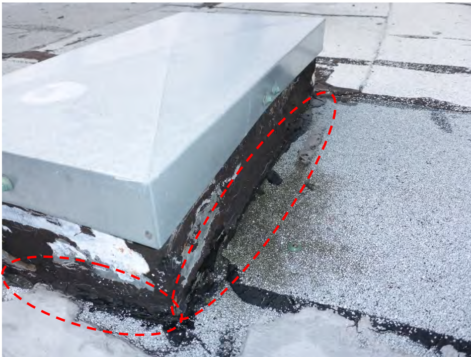
Photo #11: Roof base flashings are improper and or are missing. Roofing should also run down the curb and lap over membrane on the deck. Open voids are present.
