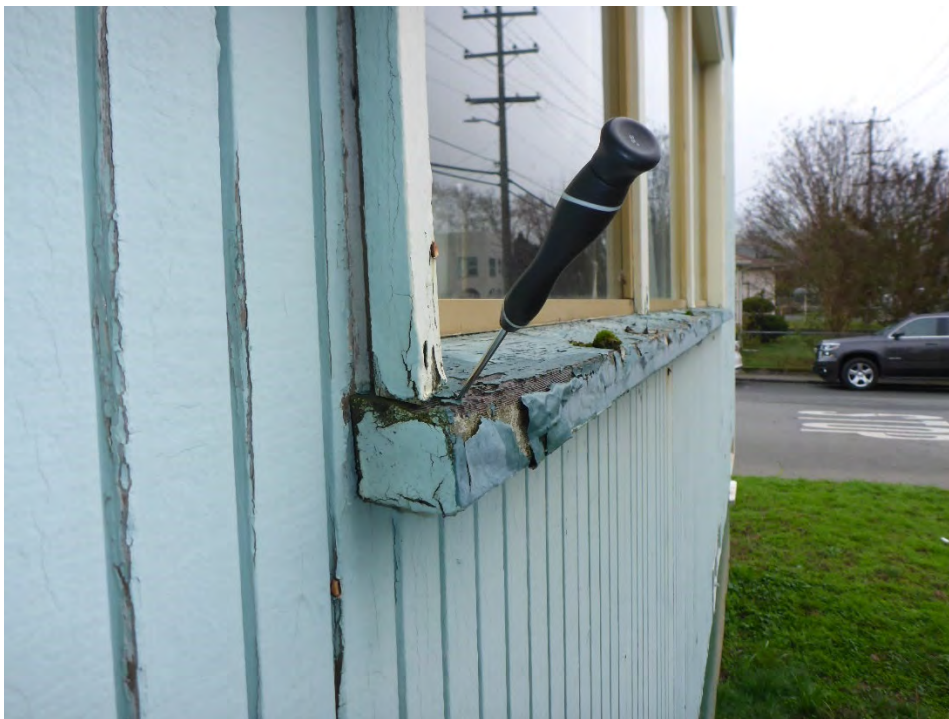
Photo #31: Exterior trim is decayed and is failing
