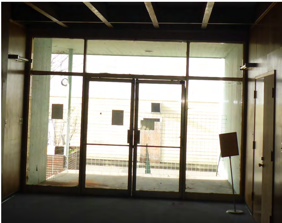
Photo #33: Exterior doors lack weather stripping.
