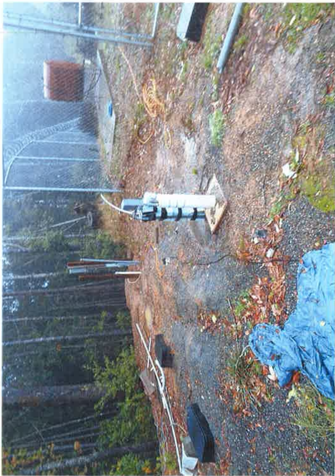
Well near Tanks
