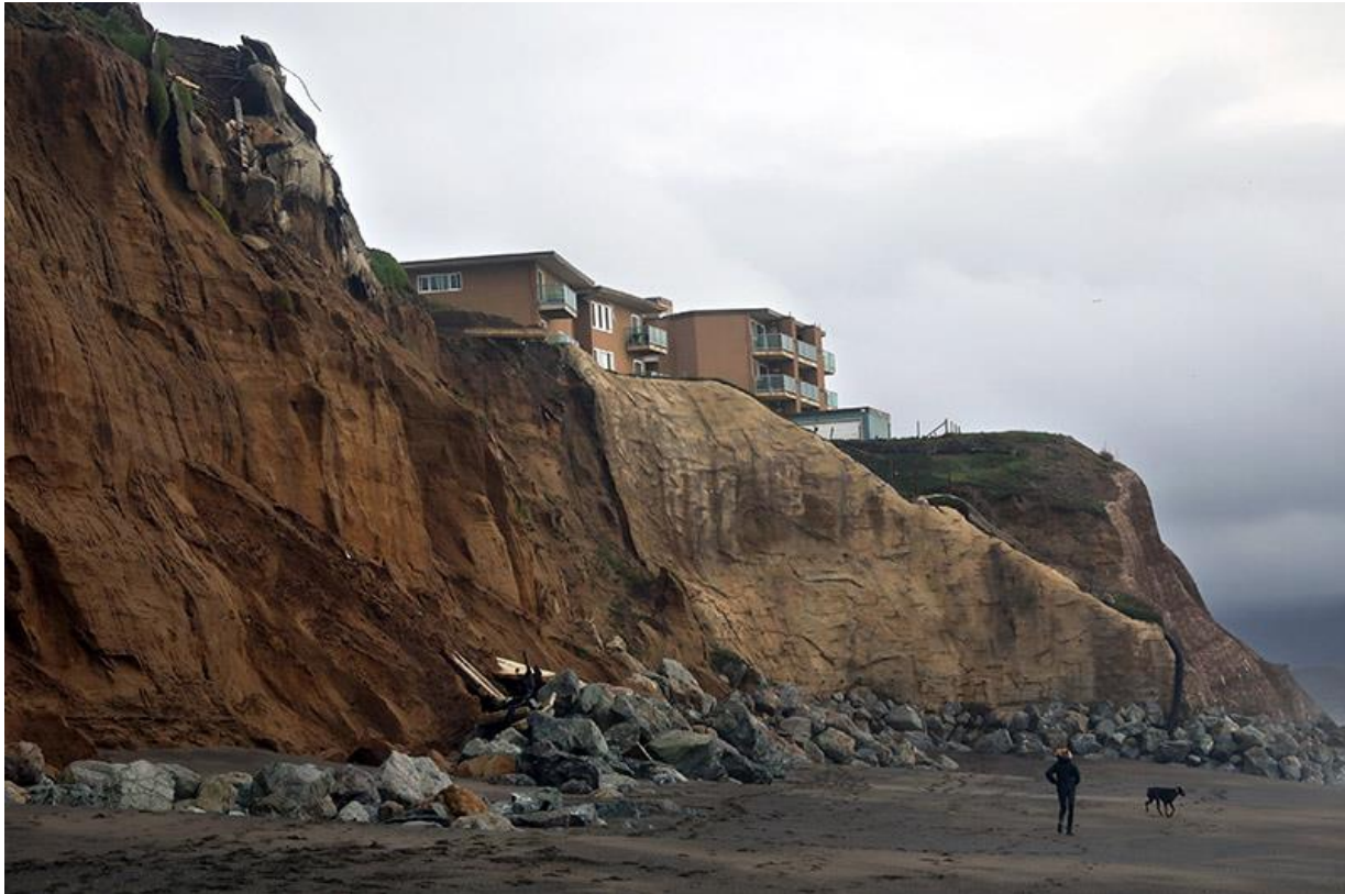
Remnants of a bluff-top apartment building in Pacifica fell down to the beach, where large rocks form a barrier against the rising sea. (Carolyn Cole / Los Angeles Times)
