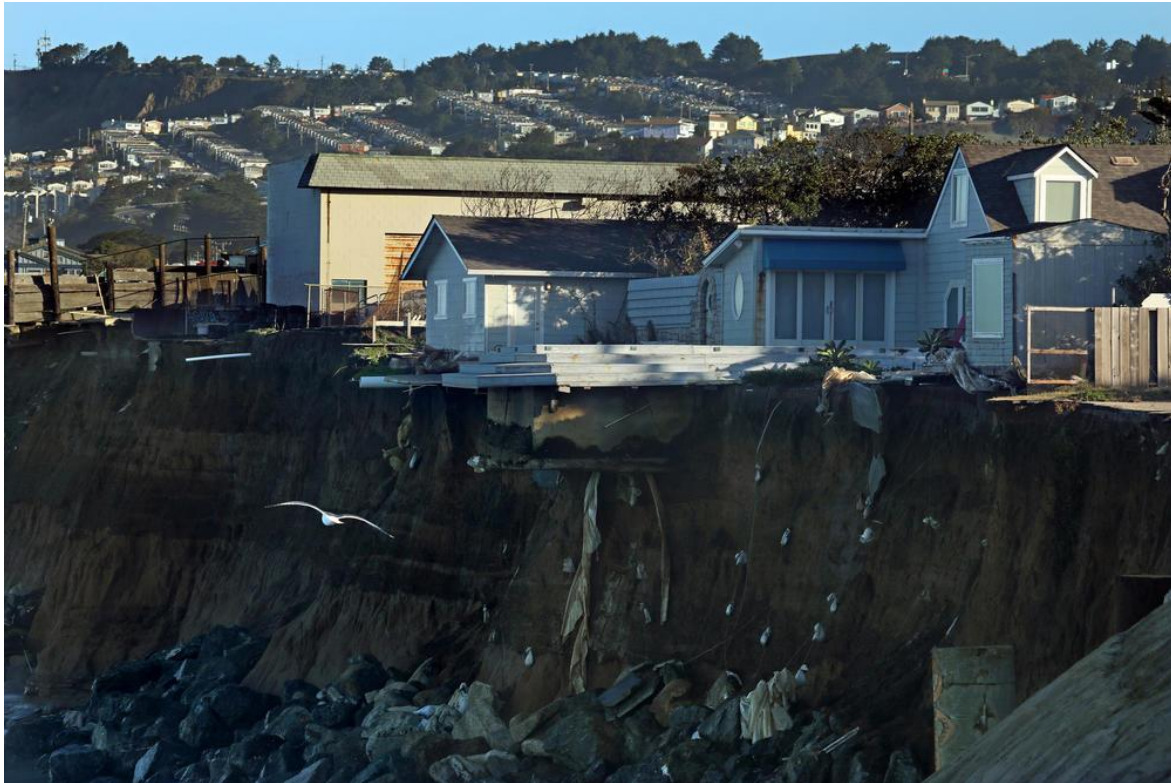
Homes along the cliffs of Pacifica are hanging on to time. Some have already been condemned or removed. (Carolyn Cole / Los Angeles Times)
