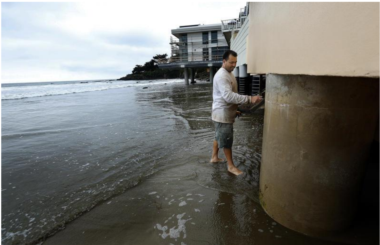
A number of homes at Broad Beach are supported by concrete columns. Rock walls and sandbags have also been deployed as protection from the sea. (Mel Melcon / Los Angeles Times)
