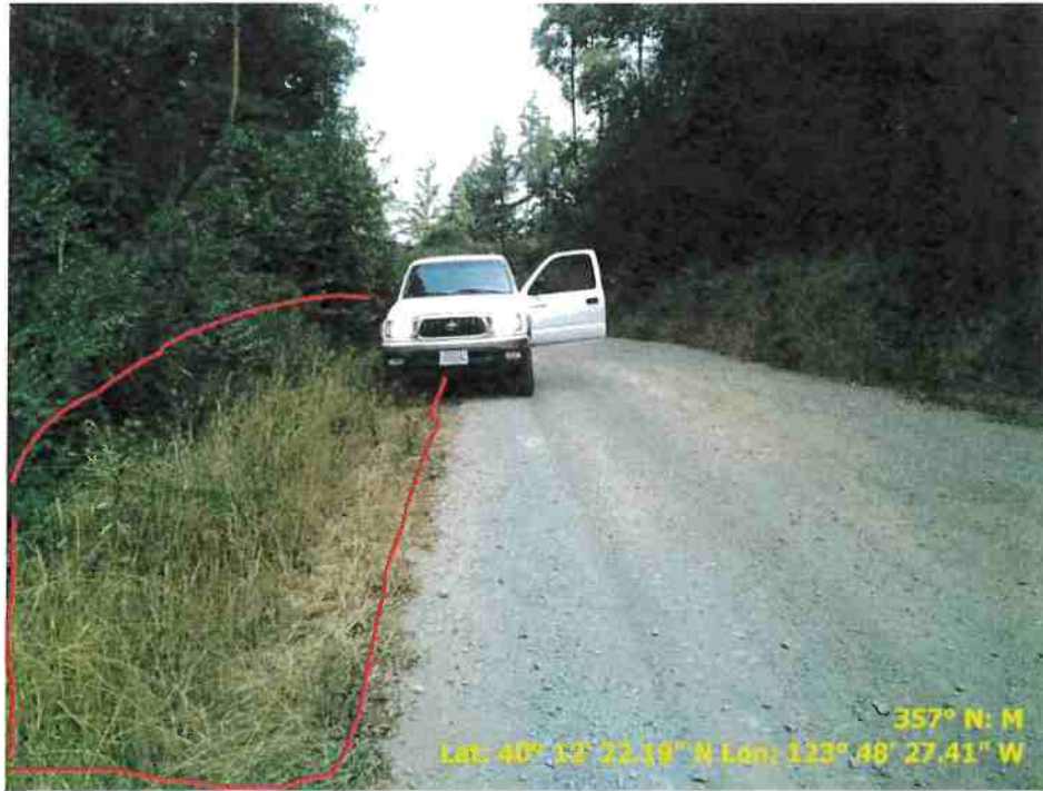
Figure 17. Photo of Road Point 76 showing a pullout that needs to be regraded...
