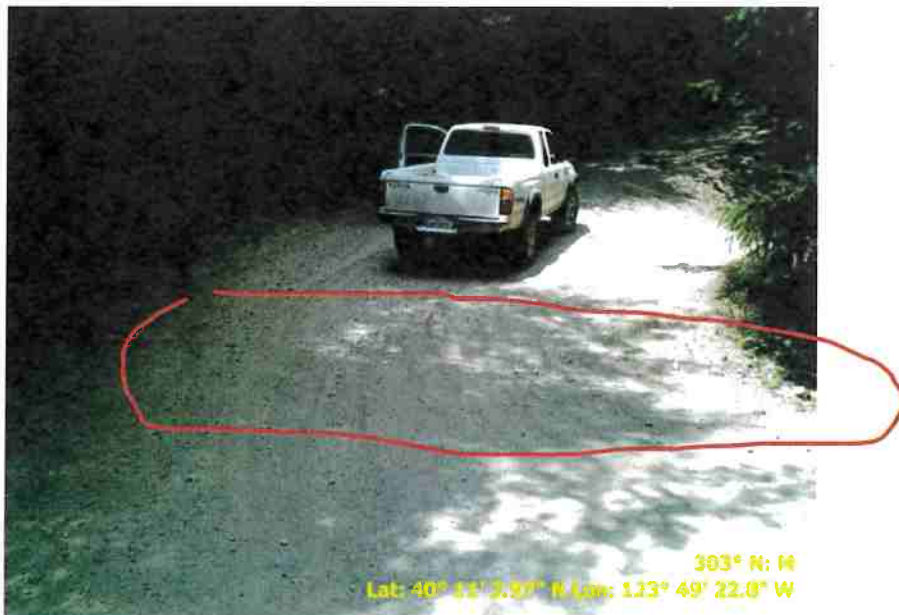
Figure 48. Photo of Road Point 159 showing a class three stream crossing that need a culvert or rock ford.
