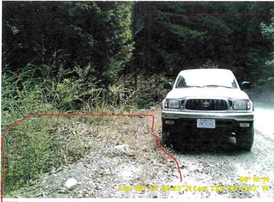
Figure 9. Photograph showing Road Point 27 which is a pullout that need to be regraded.
