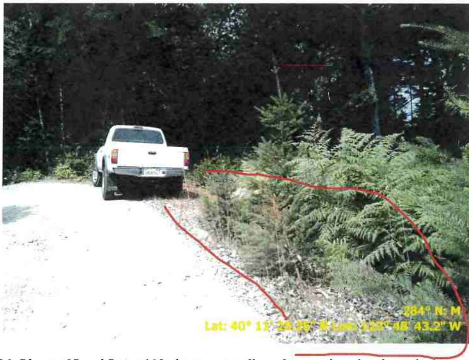
Figure 36. Photo of Road Point 118 showing a pullout that needs to be cleared of vegetation and regrading.
