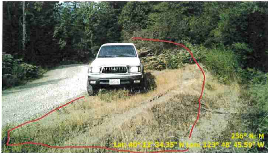
Figure 13. Photograph showing Road Point 64 which is a pullout that needs to be regraded to make room for larger vehicles.
