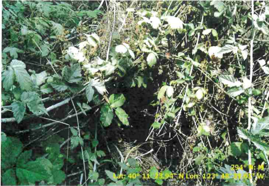
Figure 35. Photo of Road Point 115 showing the inlet of a 36" onstream culvert that needs the inlet cleared.
