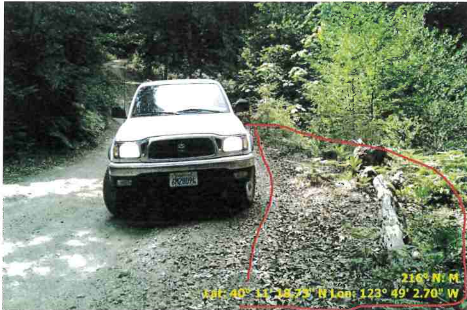
Figure 49. Photo of Road Point 162 showing a pullout that needs to be cleared of vegetation and regraded.
