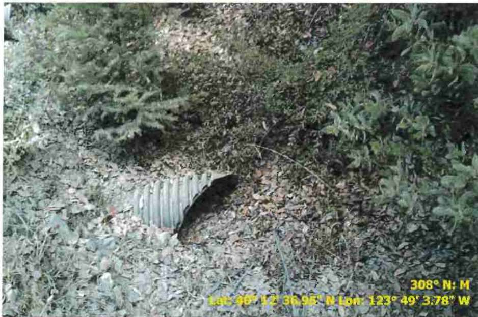
Figure 12. Photograph showing Road Point 42 which is 18" drainage relief culvert with debris in the inlet that needs to be cleared.
