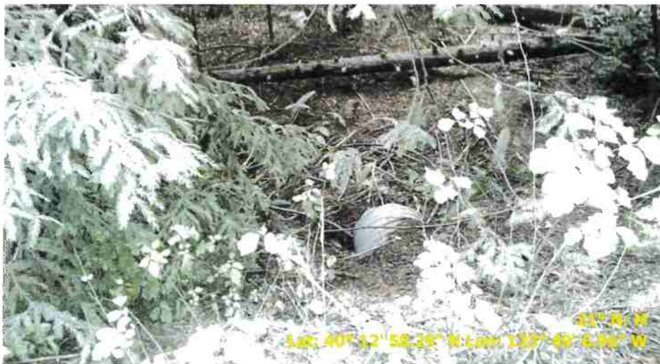
Figure 4. Road point 58 showing an 18-inch drainage relief culvert that is in good condition.
