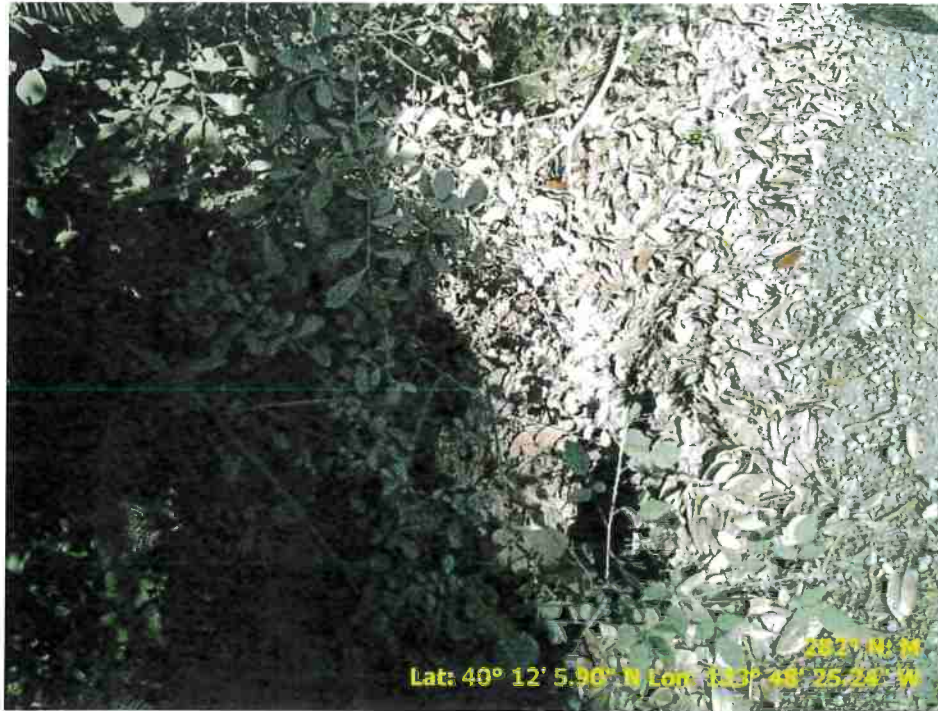
Figure 21. Photograph of Road Point 82 showing an a partially plugged inlet to an 18 inch drainage relief culvert. The fix is to clear the inlet with a shovel.
