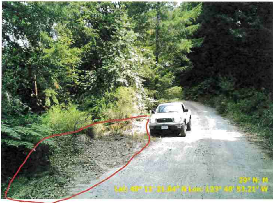
Figure 38. Photo of Road Point 123 showing a pullout that needs to be cleared of vegetation and regrading.
