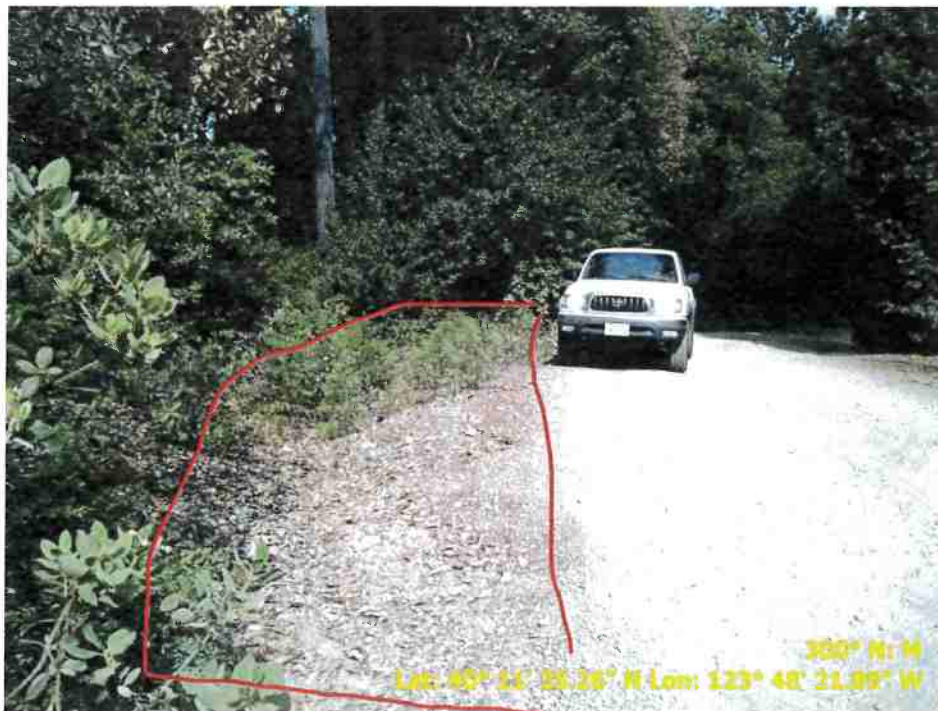
Figure 28. Photo showing a pullout that needs to be regraded and vegetation cleared.
