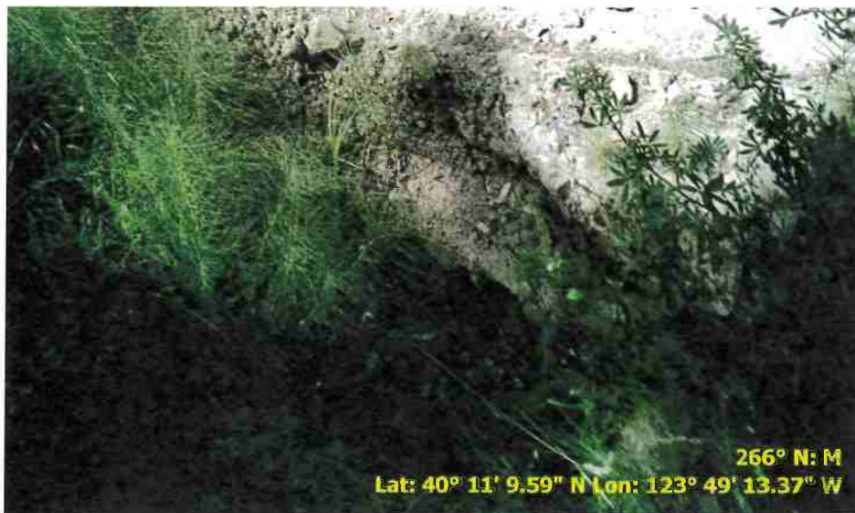
Figure 46. Photo of Road Point 148 showing the inlet of an 18" onstream culvert that needs the inlet cleared and the inlet needs rock slope protection above and around the inlet.
