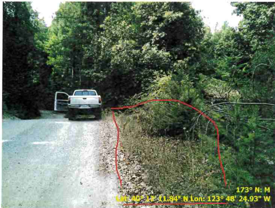
Figure 20. Photo of Road Point 80 showing a pullout that needs to be regraded and vegetation cleared.
