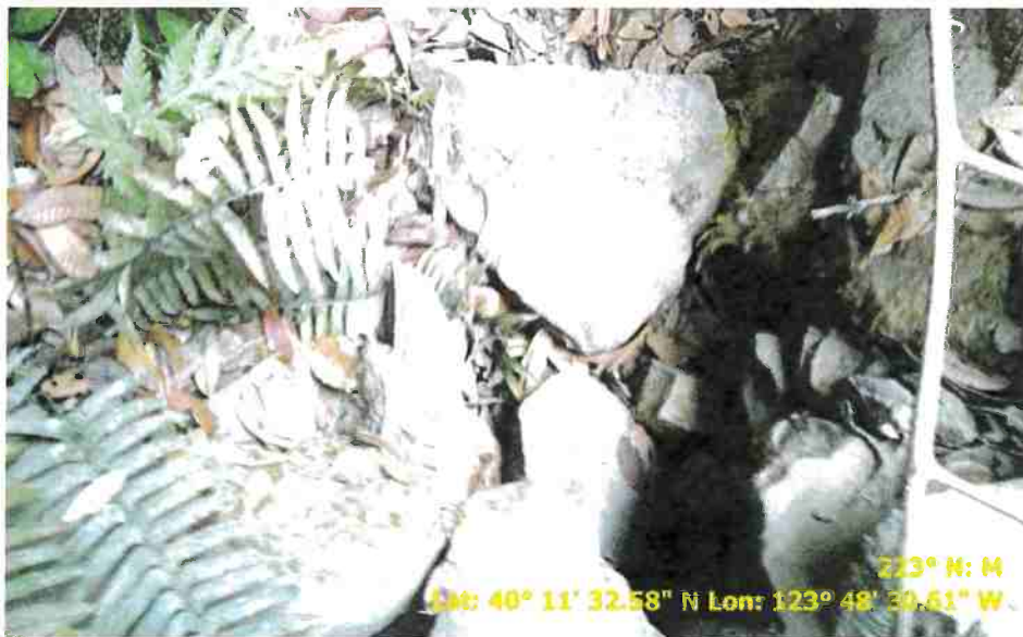
Figure 32. Photo of Road Point 190 showing the inlet of an 18" drainage relief culvert that needs to be cleared.
