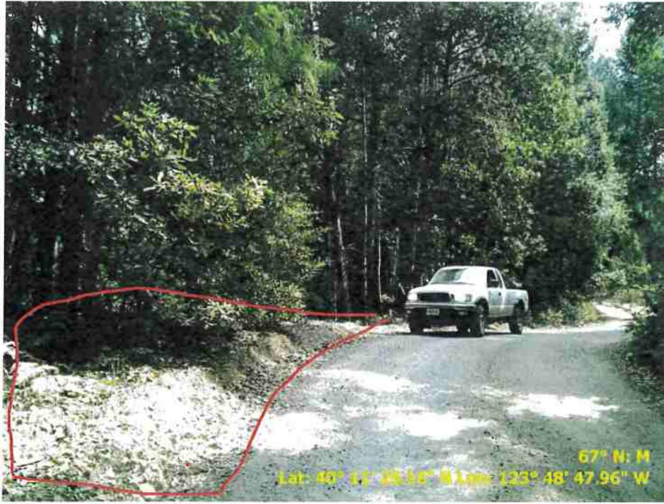
Figure 37. Photo of Road Point 119 showing a pullout that needs to be cleared of vegetation and regrading.
