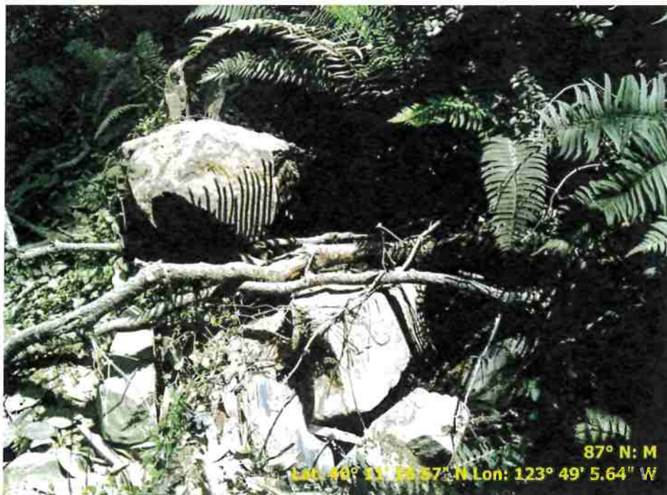
Figure 40. Photo of Road Point 132 showing the inlet of a 18" onstream culvert that needs the inlet cleared.
