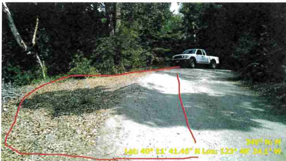
Figure 30. Photo of Road Point 103 showing a pullout that needs to be regraded.
