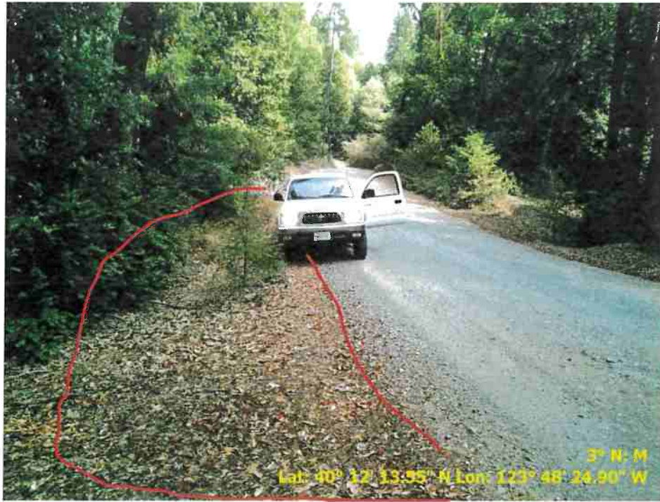
Figure 19. Photo of Road Point 79 showing a pullout that needs to be regraded and vegetation cleared.
