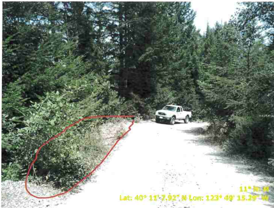
Figure 47.. Photo of Road Point 150 showing a pullout that needs to be cleared of vegetation and regraded.
