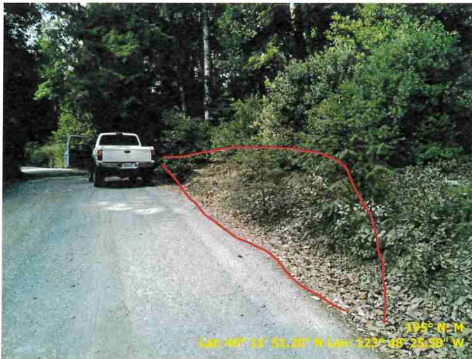
Figure 24. Photo of Road Point 89 showing a pullout that needs to be regraded and vegetation cleared.
