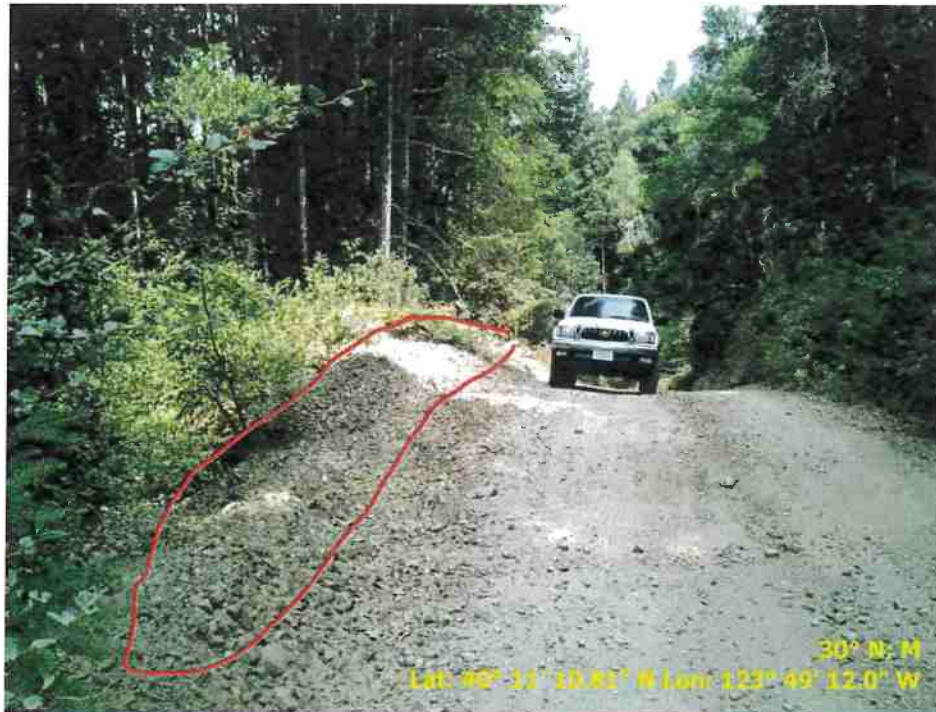
Figure 45. Photo of Road Point 145 showing a pullout that needs to be cleared of vegetation and regraded.
