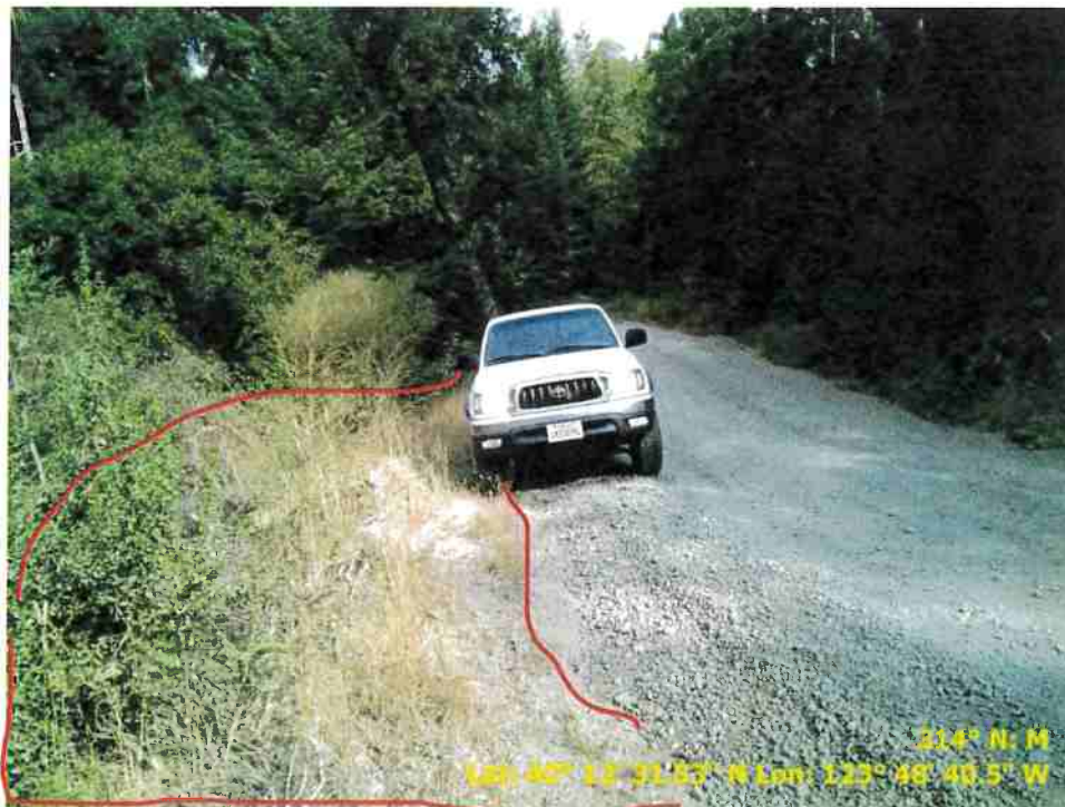
Figure 14. Photo of Road Point 67 showing a pullout that needs to be regraded and vegetation cleared.
