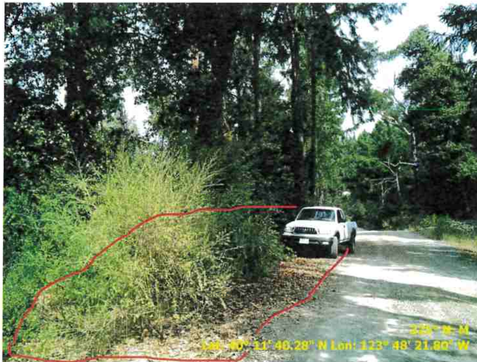
Figure 26.. Photo of Road Point 94 showing a pullout that needs to be regraded and vegetation cleared.
