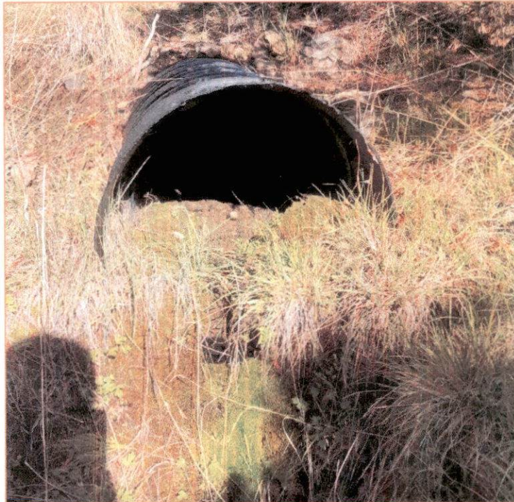
RP9) Clean and maintain DRC outlet.
