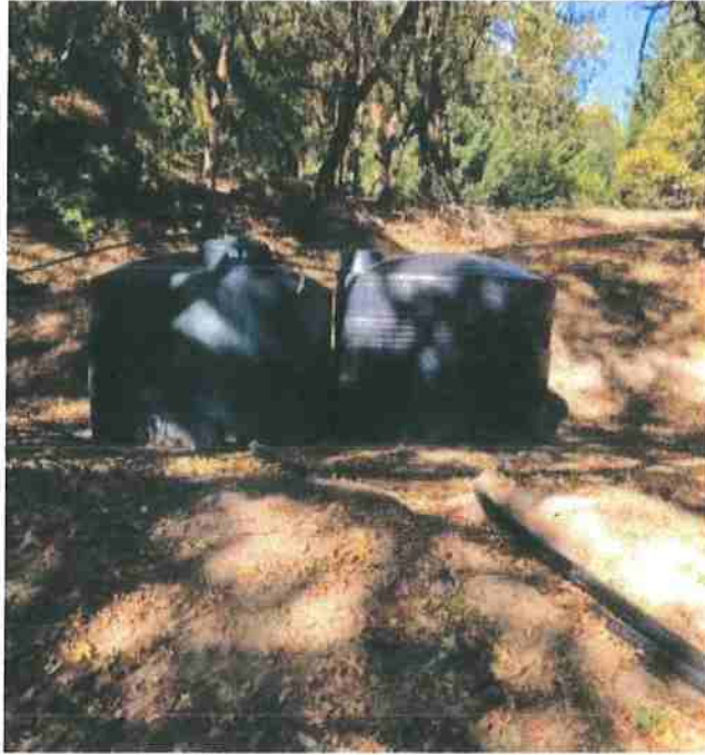
2500 Gallon Holding Tanks by Well 1
