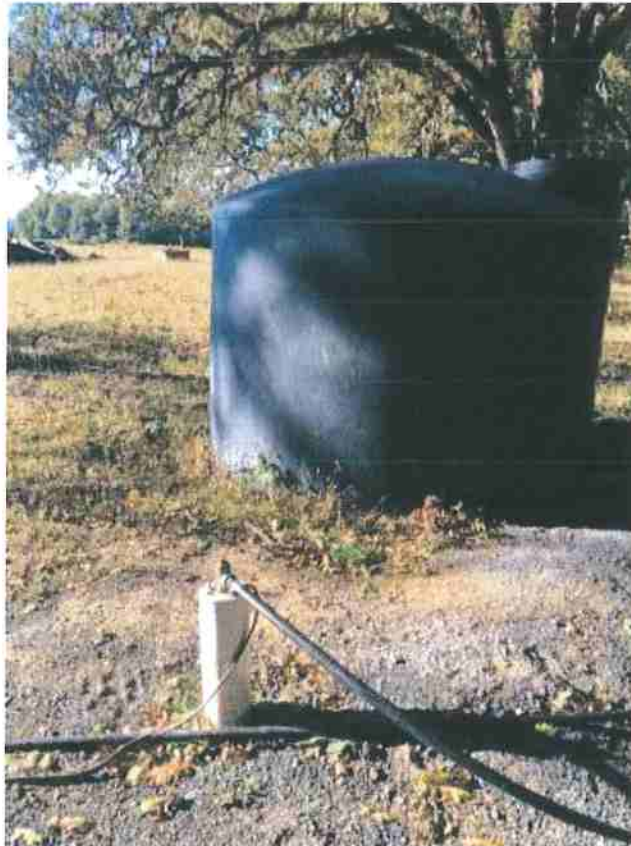
Well 2 and 2500 Gallon Holding tank
