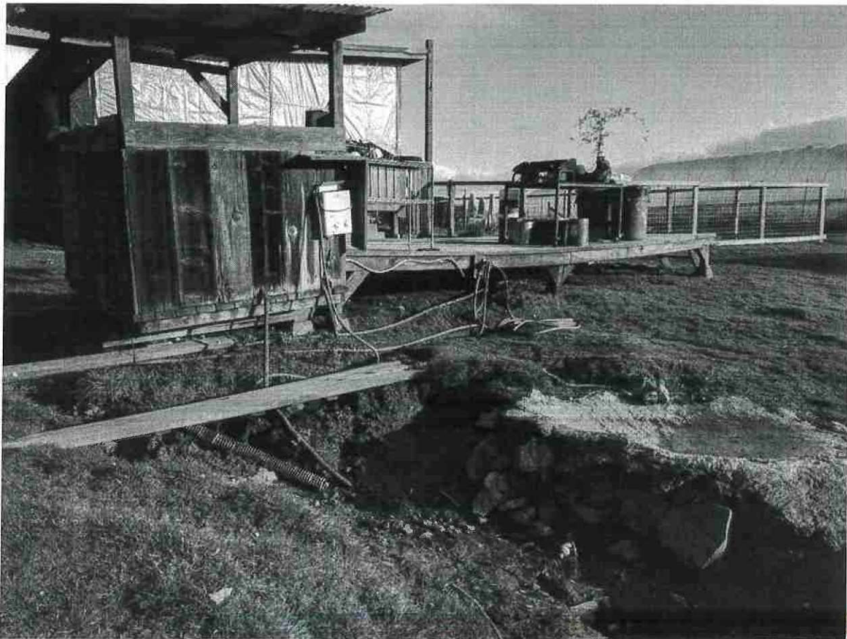
Photograph #45– Structure within Class III watercourse riparian area; Upstream of SC8; Further consultation with county and state agencies to determine variance options
