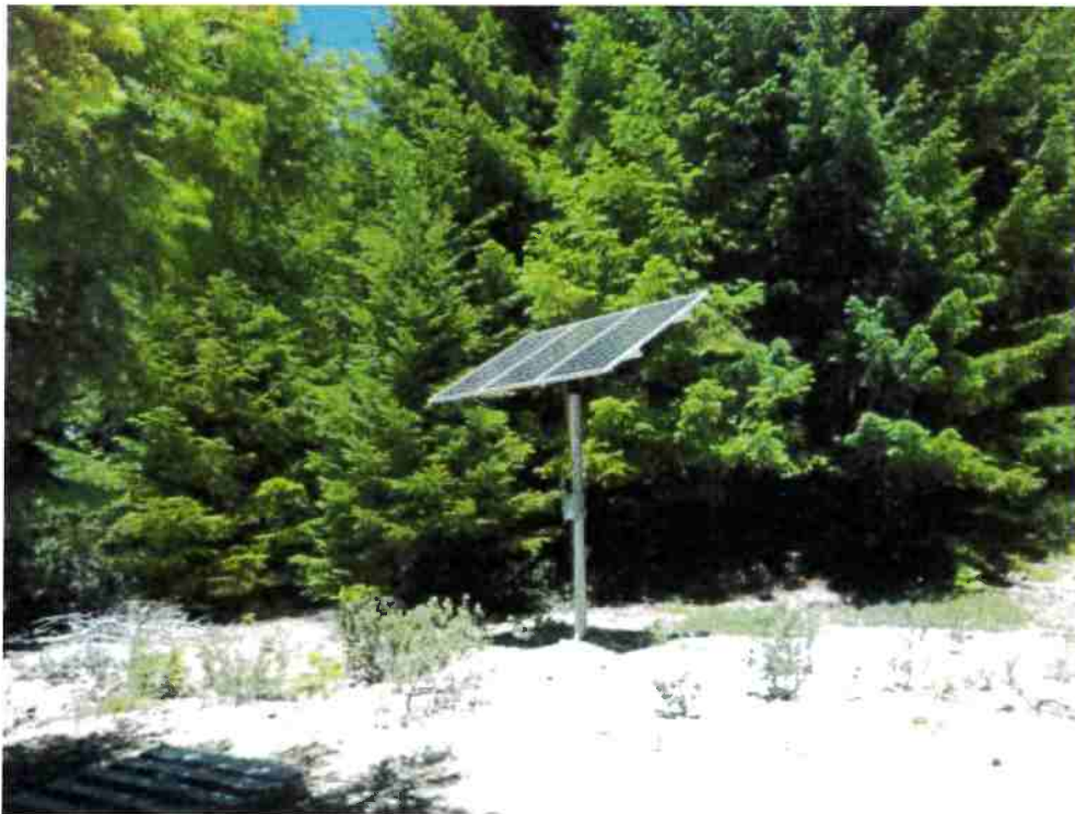
Photo 11. Solar panel for well
