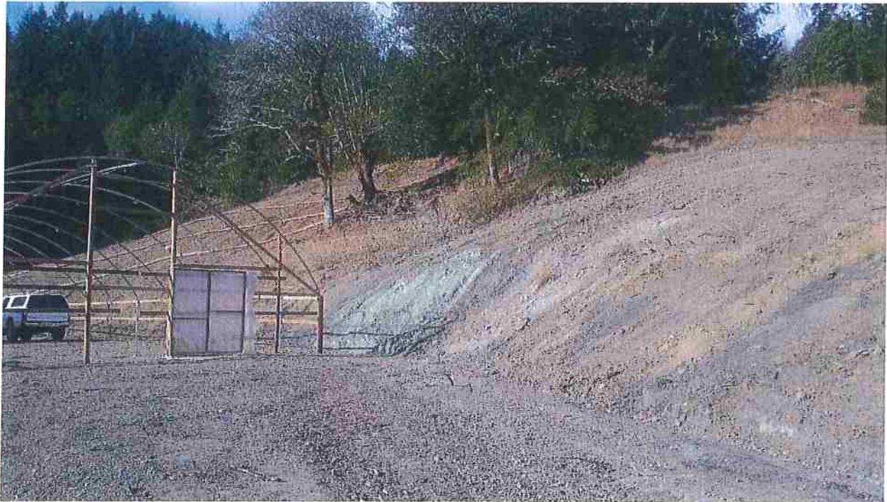
Figure 19: Straw wattles placed on the disturbed area of the hillslope above the greenhouse.
