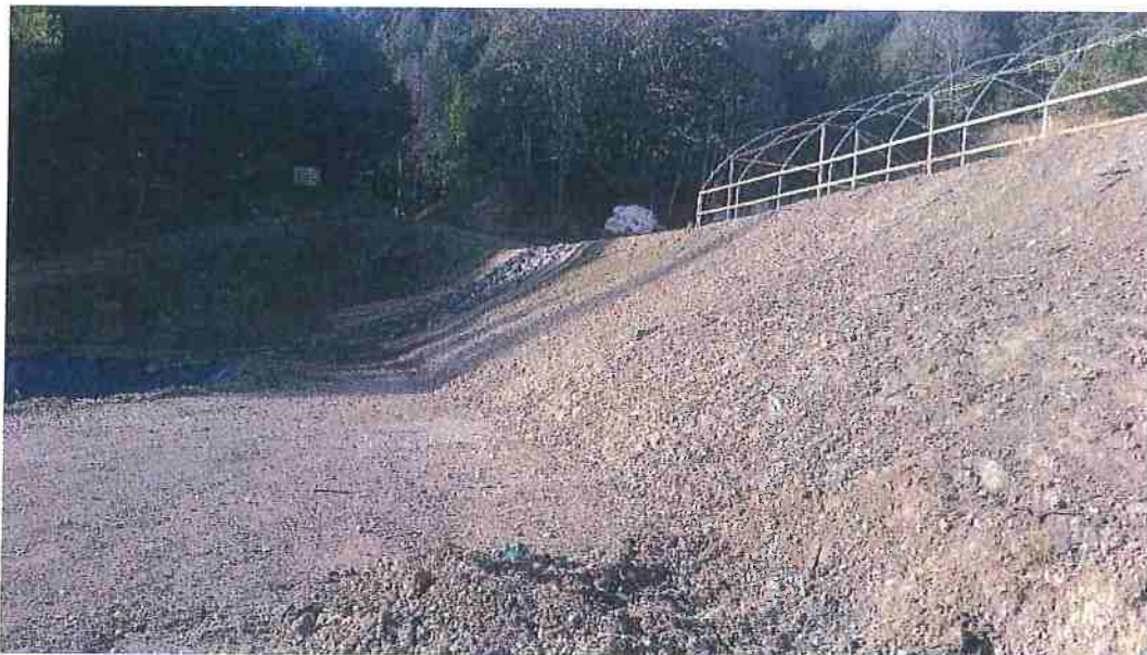
Figure 18: Jute netting, rip rap and grass seed starting to take near the inlet apron. Other disturbed areas require similar measures.
