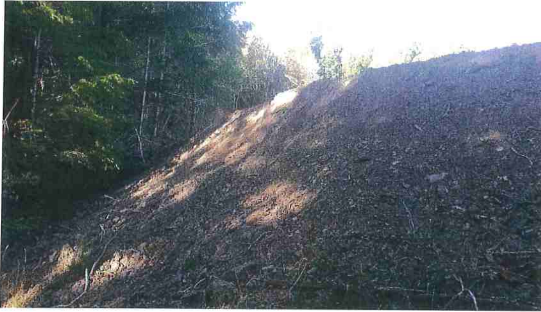
Figure 6: Southeast corner of pond, looking approximately West, near the top of the legacy pond overflow scour area.
