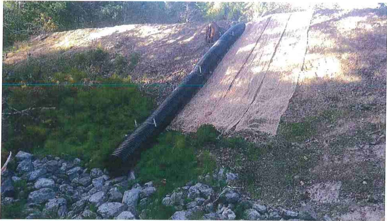
Figure 11: South Pond overflow consisting of an 18" culvert which outlets onto a rock apron where water is directed into a swale.
