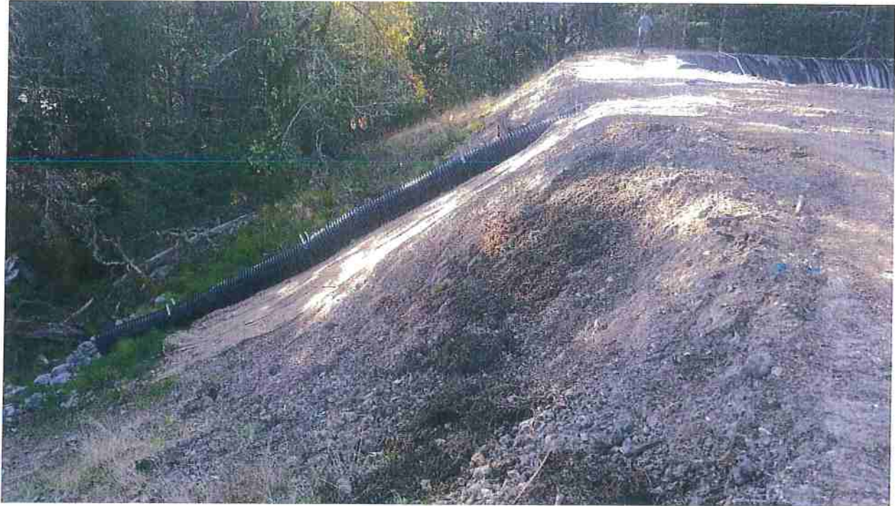
Figure 10: East dam wall of the South Pond as it appears looking South. Note the ~8-ft minimum crest width and 2:1 exterior fill slopes to native near the overflow.
