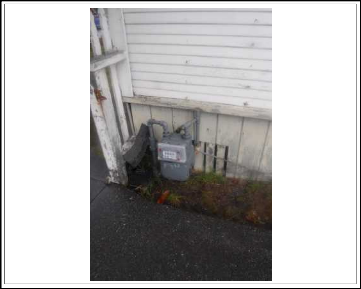
Gas Meter Utility
