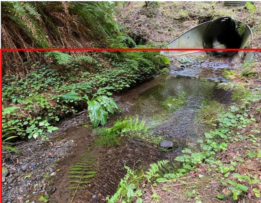
Figure 9. Temporary impact area (red box): Savage Creek existing intake facility (zoomed in) to be replaced
