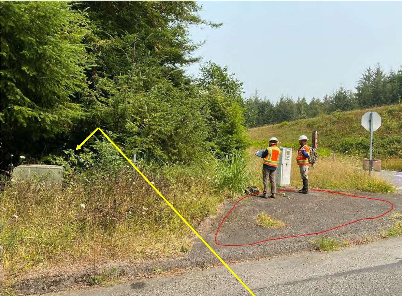
Figure 3. Location for backwash system (looking northeast)
