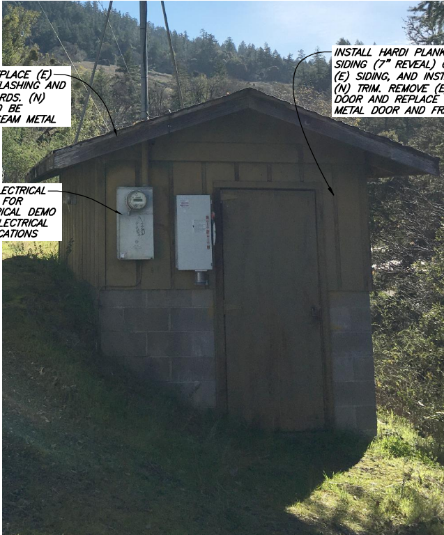
PUMP STATION EXTERIOR
