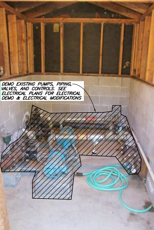
PUMP STATION INTERIOR
