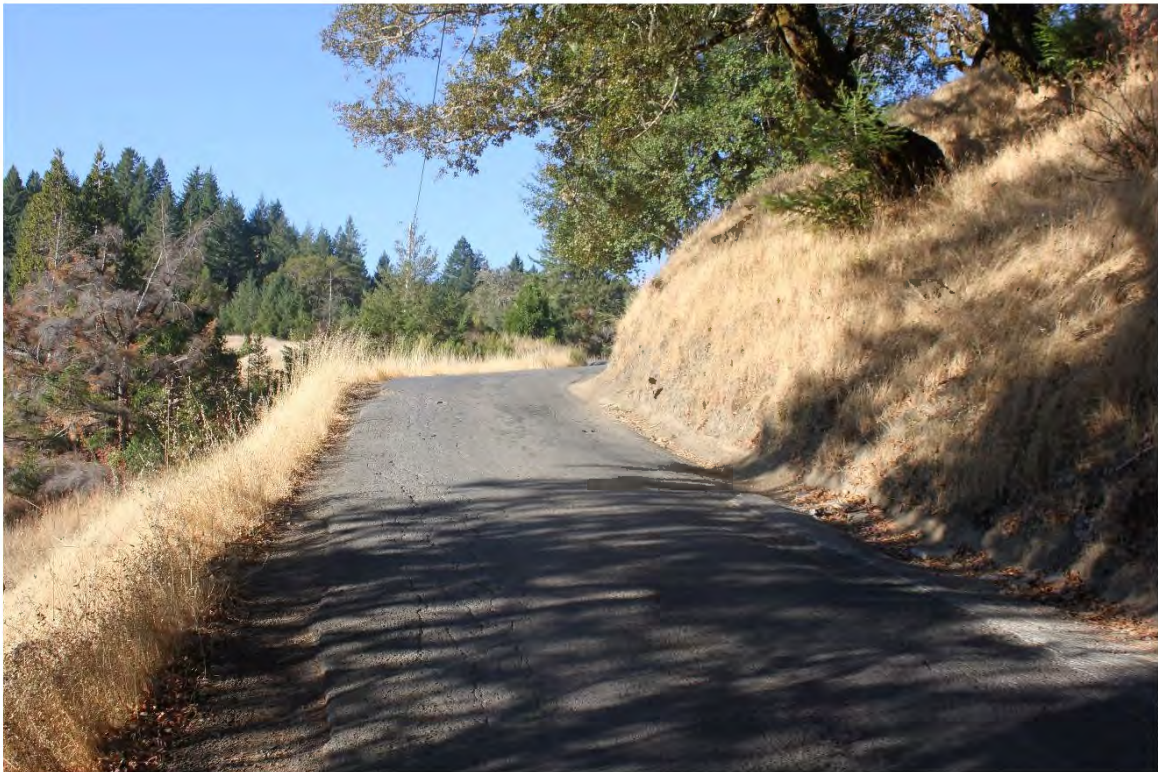
Photo 42. Mile 3.65: Blind corner - 12-ft road width with 1-ft shoulders. Potential location to widen corner on inside to improve width and visibility.
