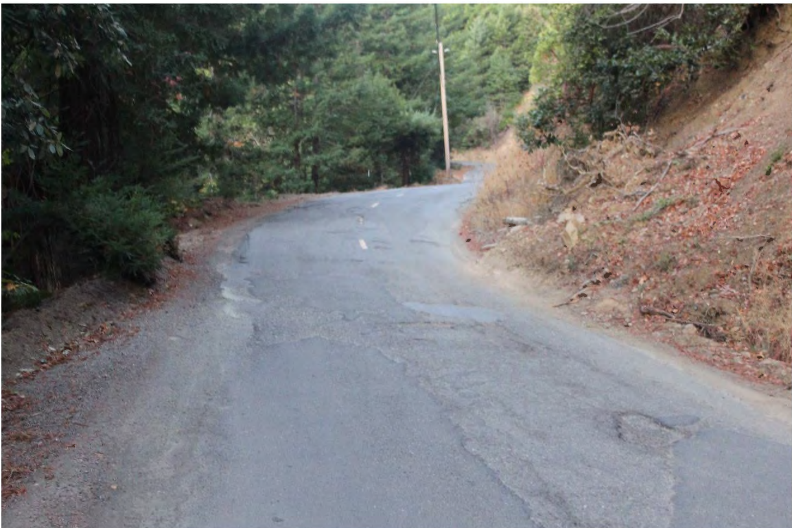
Photo 2. Mile 0.3: Pinch point at recent debris slide and tree; 14' width, no shoulder, blind corner, dangerous spot.
