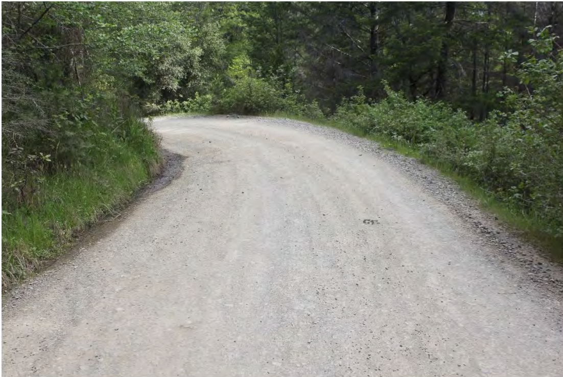
Photo 10. Mile 0.7: 16' width, 1' shoulders at blind corner, road is traversing steep area so difficult to widen.
