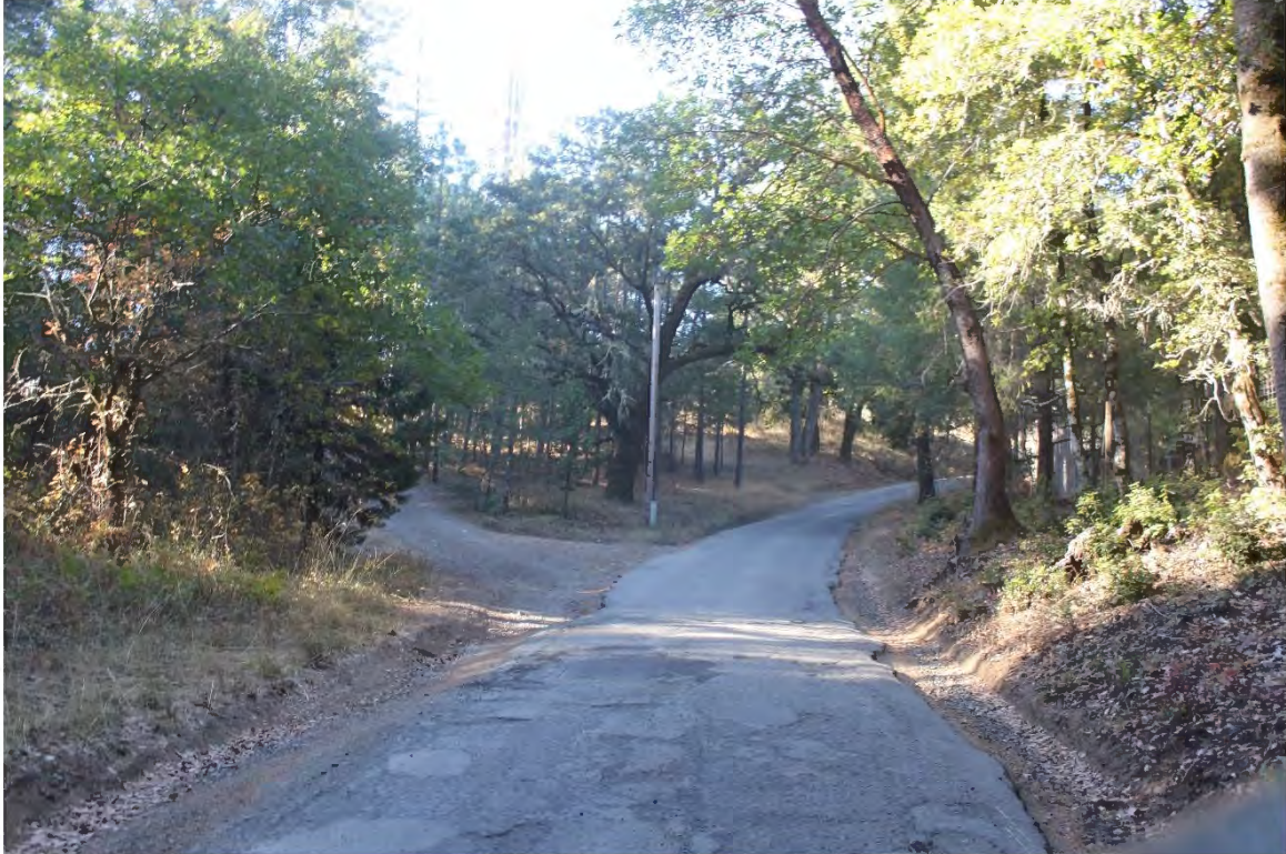
Photo 47. Mile 4.0: 15-ft road width with 2-ft shoulders. Broken pavement edges make segment more treacherous.
