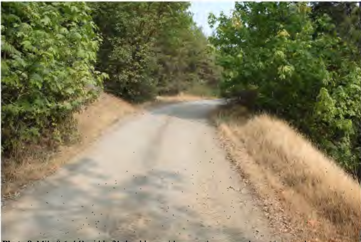
Photo 8. Mile 0.6: 14' width, 2' shoulders, with vegetation encroachment into roadway.
