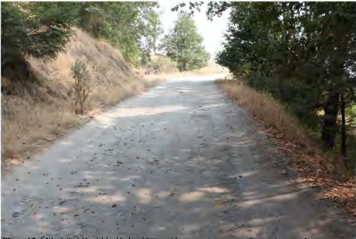
Photo 12. Mile 1.0: 14' width, 1' shoulders, with vegetation encroachment into roadway.
