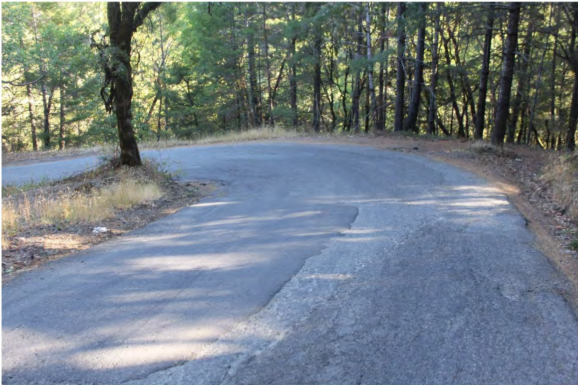
Photo 40. Mile 3.5: 18-ft road width with 1-ft shoulder. Very steep, sharp corner where trucks often get stuck. Consider re-engineering grade and curve radius.
