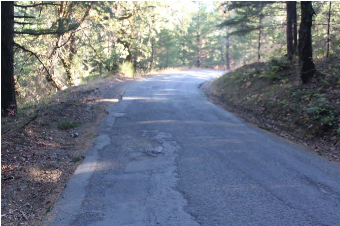
Photo 46. Mile 3.9: 15-ft road width with 2-ft shoulders. Broken pavement edges make segment more treacherous.
