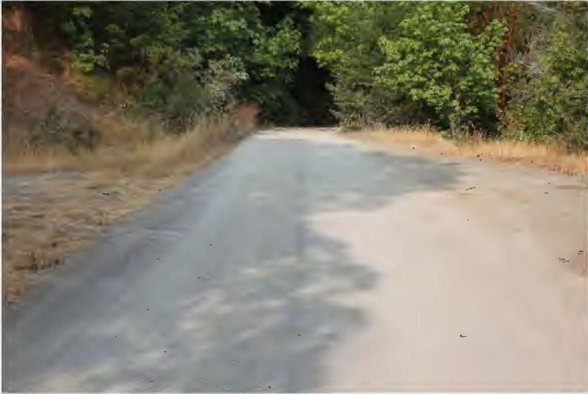
Photo 5. Mile 0.3: 18' width, 2' shoulders; blind corner to west with vegetation encroachment into roadway.
