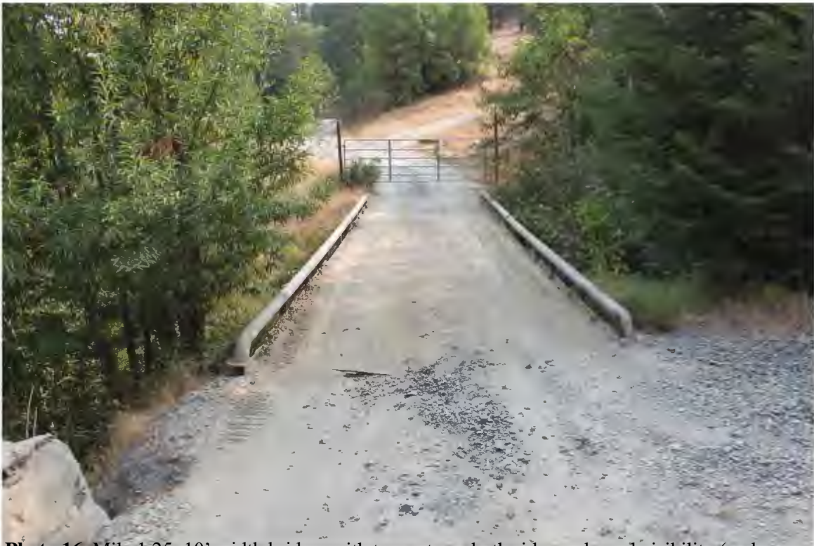
Photo 16. Mile 1.25: 10' width bridge, with turnouts on both sides and good visibility (end Segment 5).
