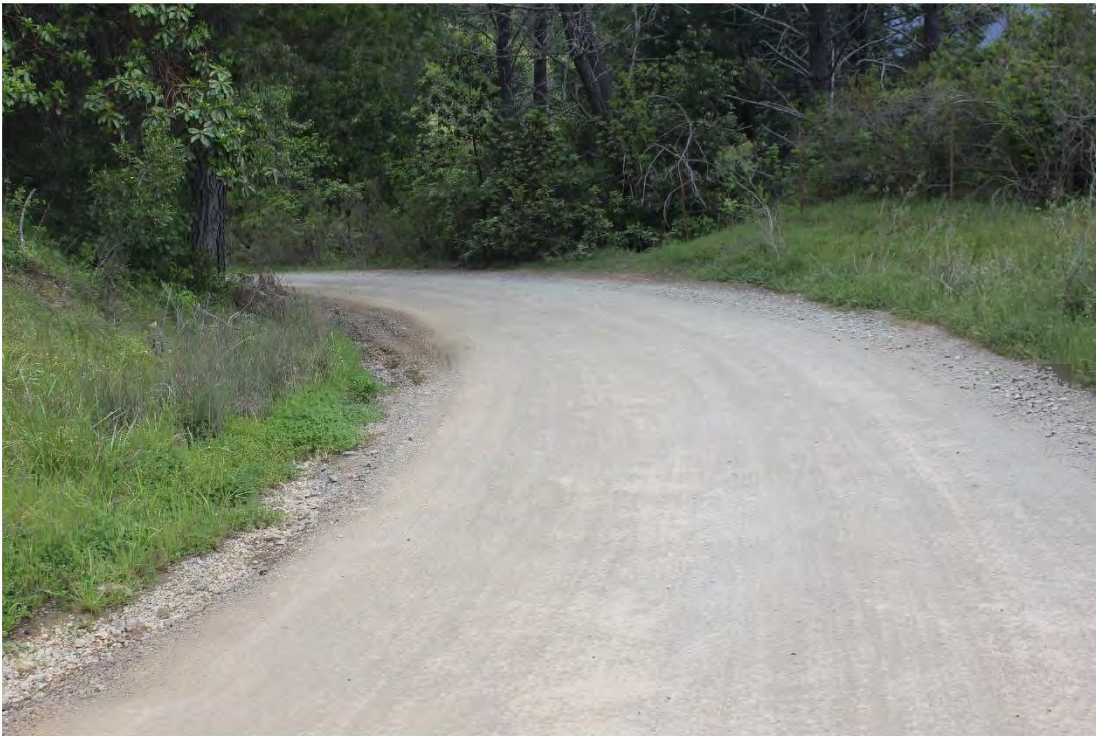
Photo 2. Mile 0.15: 14' width, 1' shoulders at blind corner with deep ditch. improve inside of turn.
