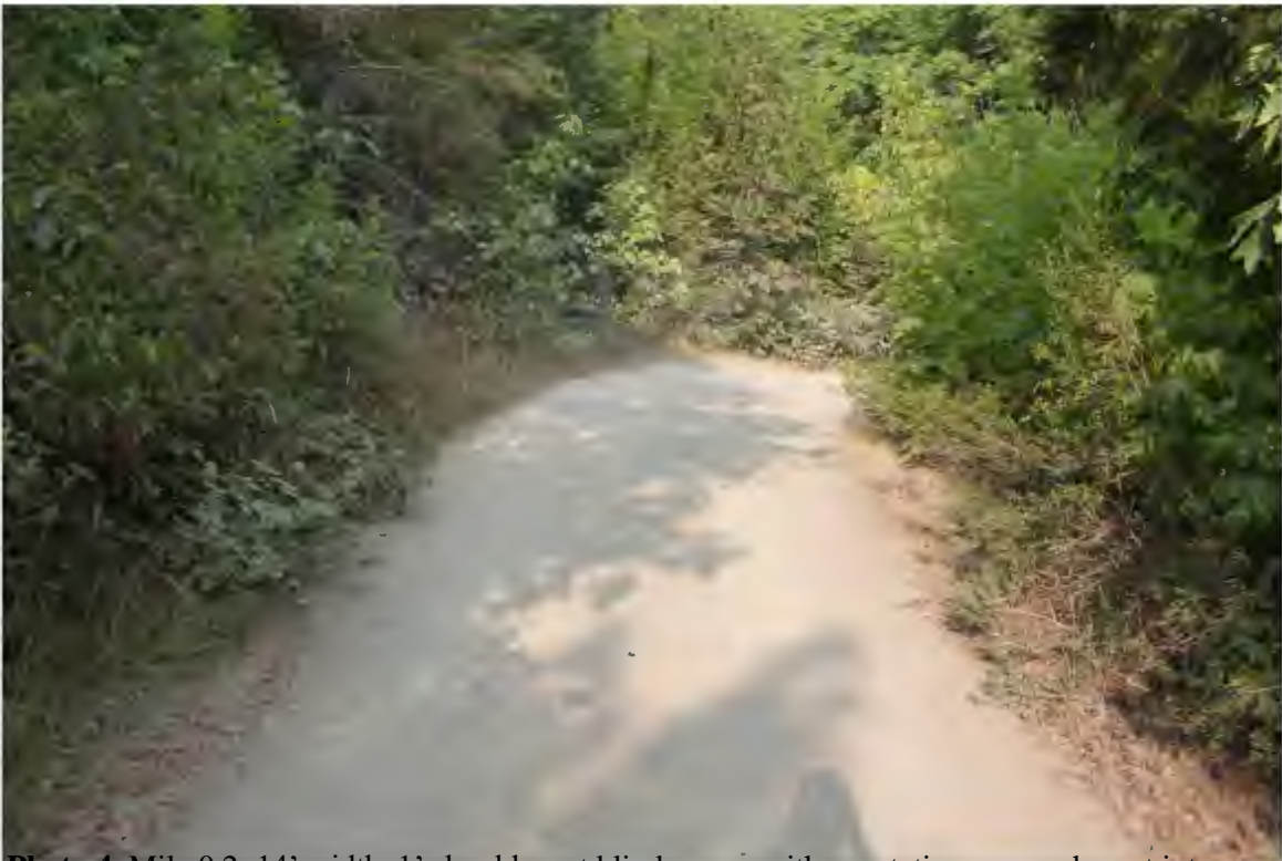
Photo 4. Mile 0.2: 14' width, 1' shoulders at blind corner with vegetation encroachment into roadway.
