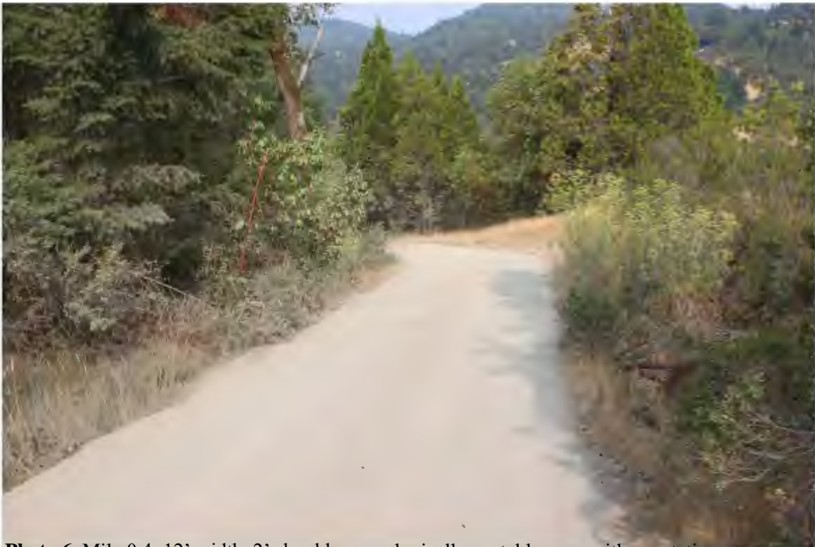
Photo 6. Mile 0.4: 12' width, 2' shoulders, geologically unstable area, with vegetation encroachment into roadway.
