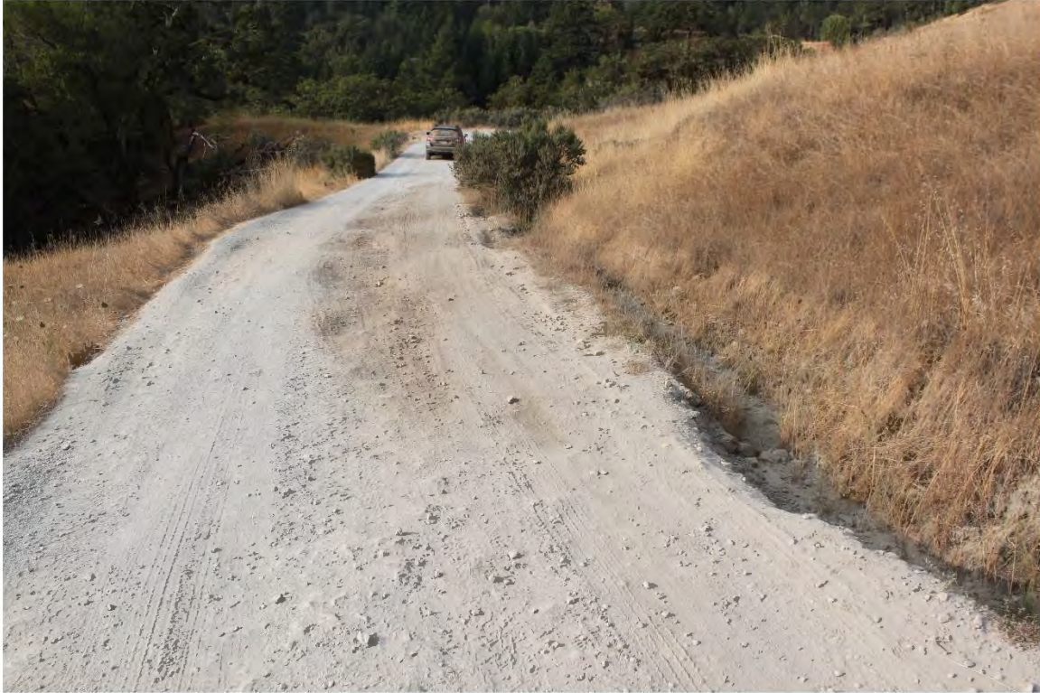
Photo 9. Mile 0.75: Eroding inboard ditch.
