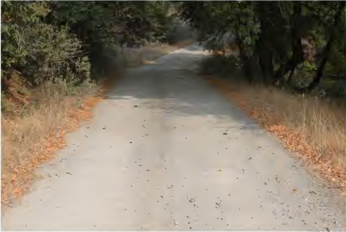
Photo 11. Mile 0.9: 14' width, 2' shoulders, with vegetation encroachment into roadway.
