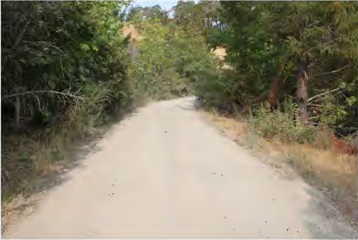
Photo 7. Mile 0.5: 12' width, 2' shoulders, with vegetation encroachment into roadway.
