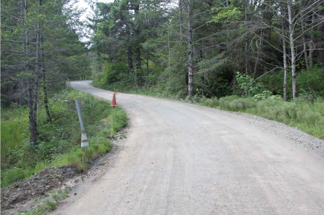
Photo 5. Mile 0.32: 16' width, no shoulders at pinch point at culvert crossing; good visibility and turnouts on both sides of crossing.
