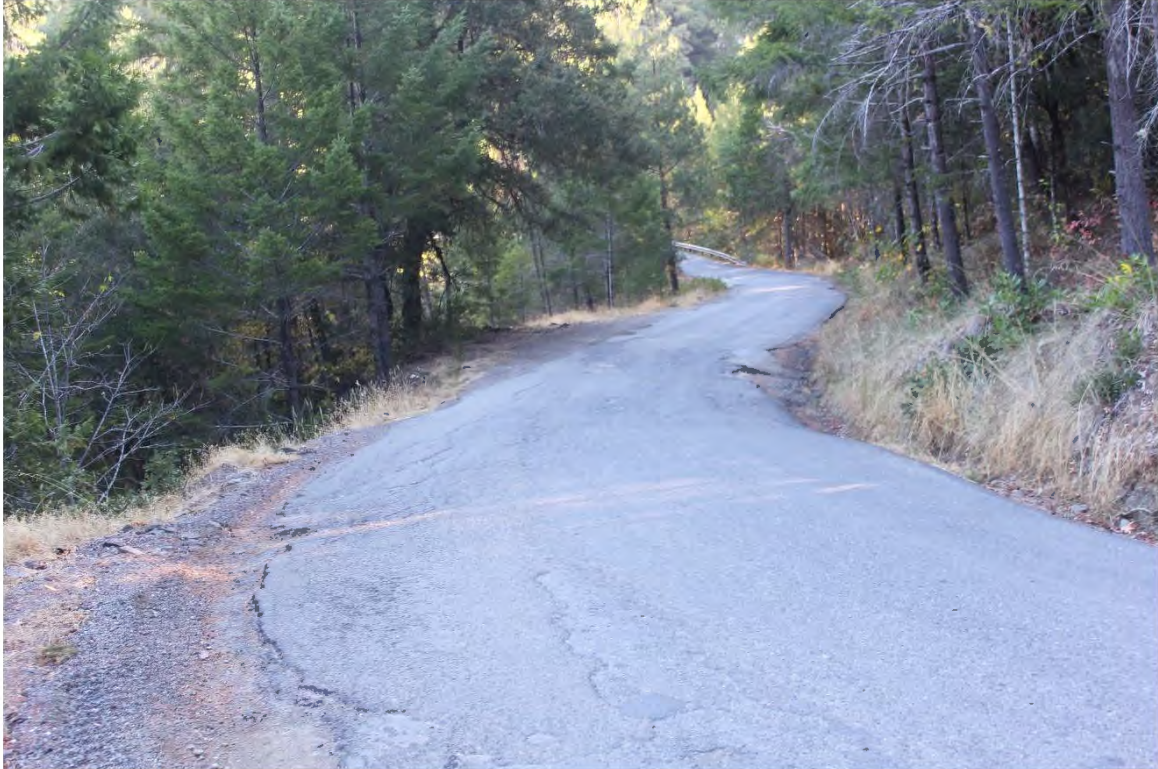
Photo 39. Mile 3.4: 16-ft road width with 1-ft shoulder. Pinch point at downgradient extent of blind corner. Potential spot to widen corner on inside to improve width and visibility.
