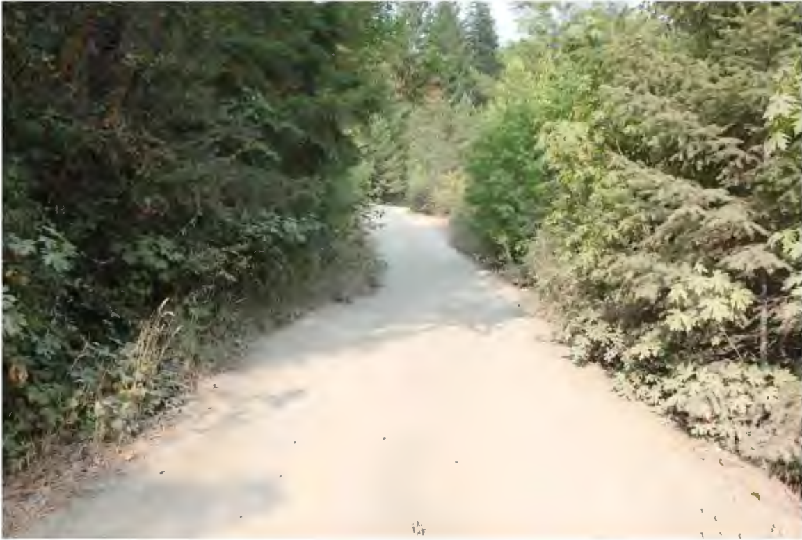
Photo 1. Mile 0.05: 12' width, no shoulders at location where road has slumped.
