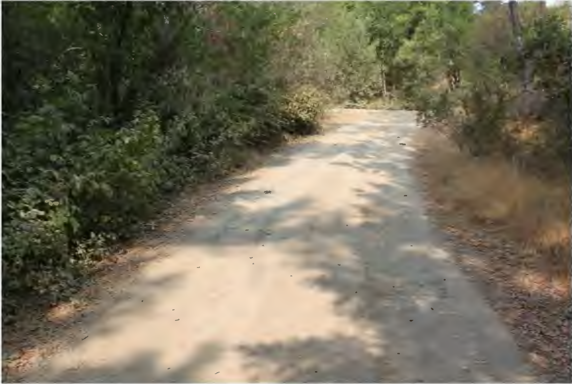
Photo 13. Mile 1.1: 14' width, 1' shoulders, with vegetation encroachment into roadway.
