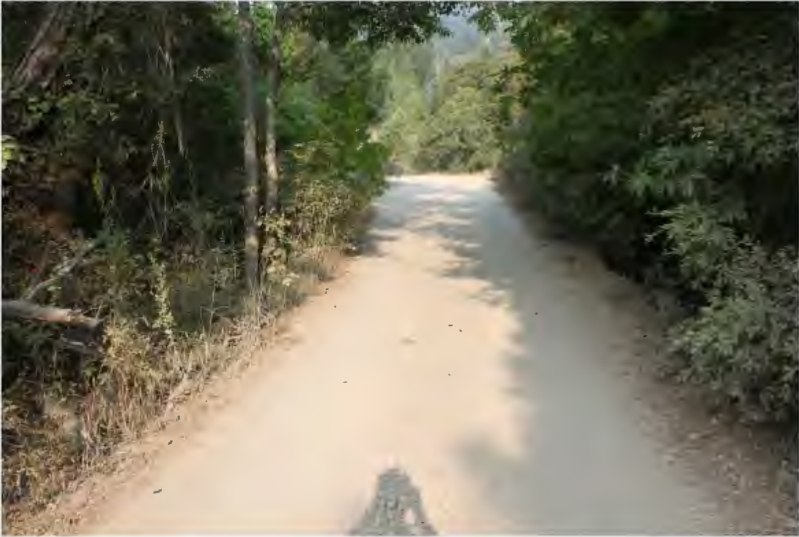
Photo 3. Mile 0.15: 12' width, no shoulders, pinch point at culvert crossing, good turnouts on both sides, but vegetation impedes visibility.
