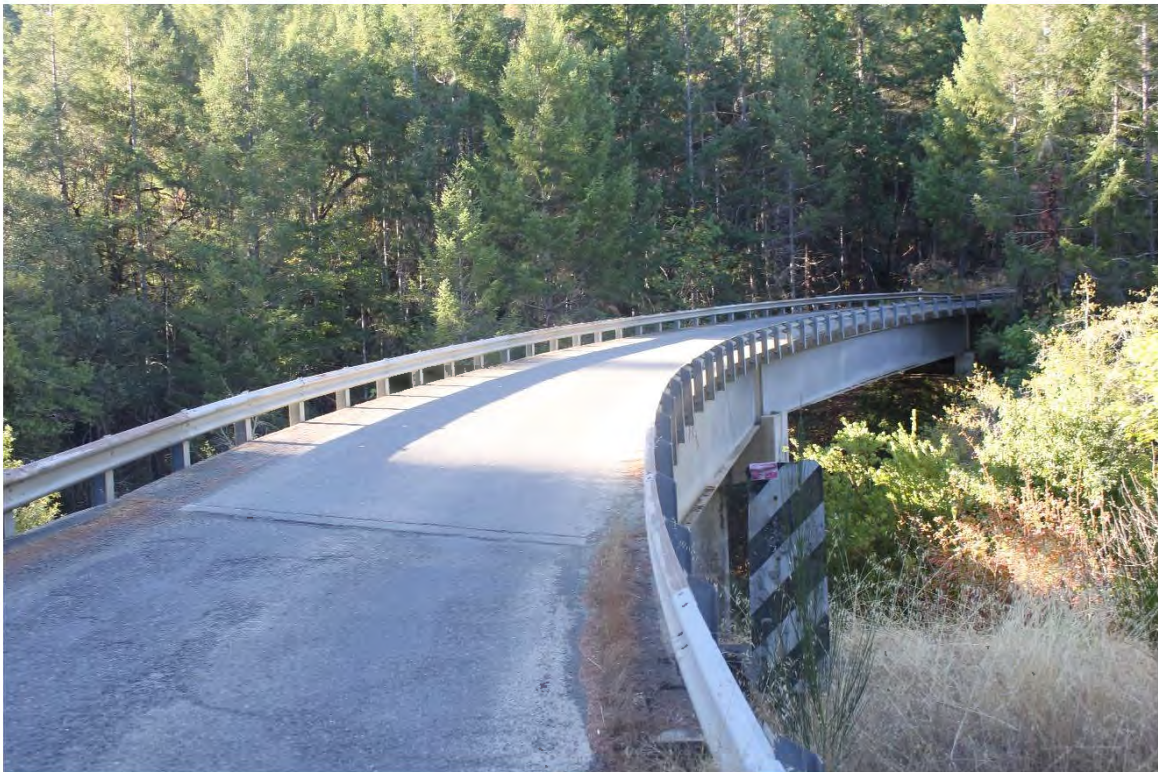
Photo 38. Mile 3.3: 16-ft wide bridge, no shoulders. Recommend removing vegetation on west extent of bridge to improve visibility.
