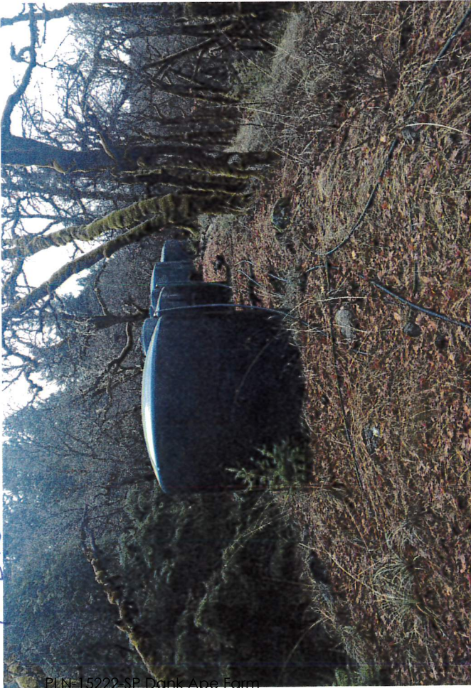
WATER STORAGE AREA 7-1550 7-2500 > GALLON TANKS
