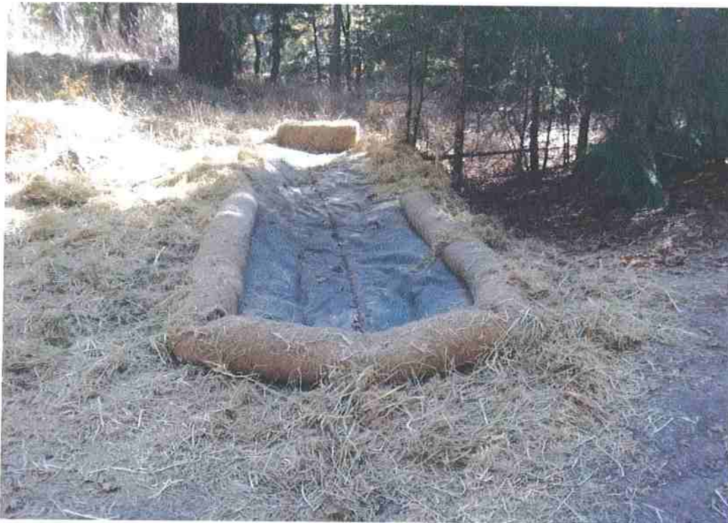
Figure 8. Interim Measure C – View of eastern culvert downstream from outlet. The objective is to return the culverted flow to sheet flow over area where there was no natural channel prior to construction.
