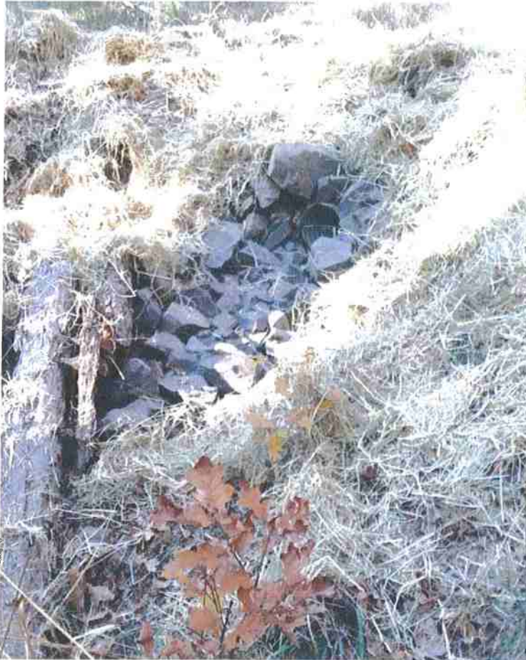
Figure 10. Interim Measure D – Western culvert, view of culvert and channel protection at outlet (left) and inlet (below).
