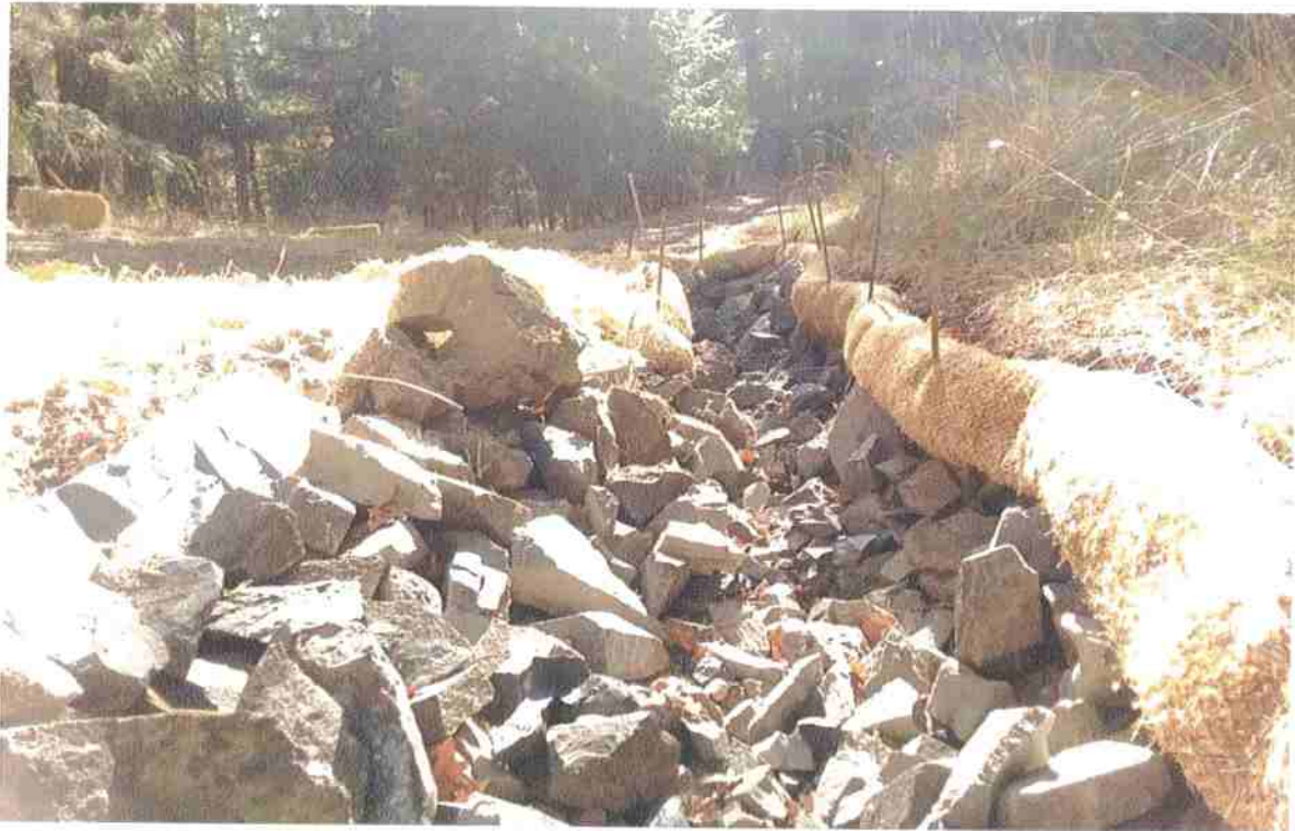
Figure 6. Interim Measure C – View of protected channel looking downstream towards culvert inlet.
