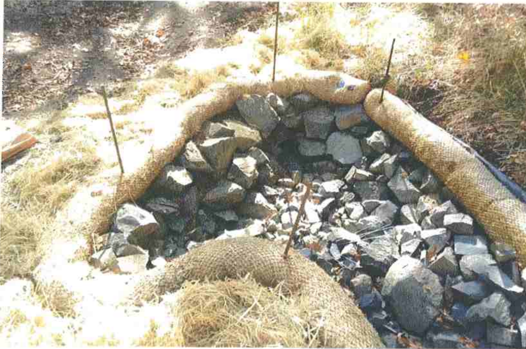
Figure 7. Interim Measure C – View of eastern culvert inlet after installation of erosion protection and flow control.
