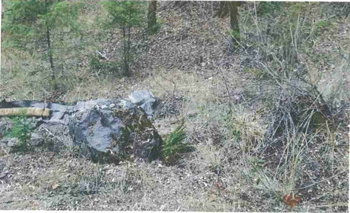
Figure 5. Interim Measure C – View of connection of natural drainage to excavated channel upstream of eastern culvert. Interim measure includes installing erosion control fabric to protect channel from further erosion and installing rock and straw wattles.
