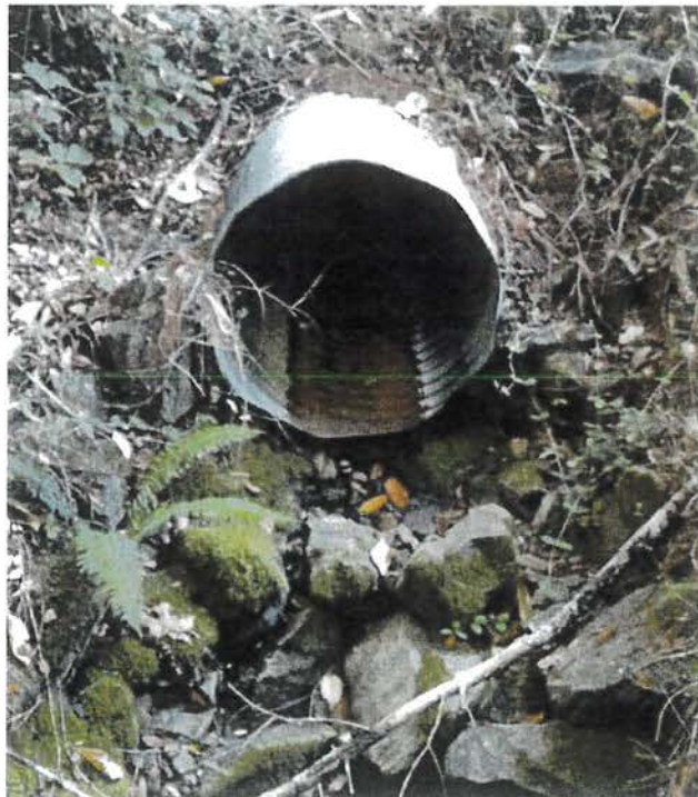
Photo looking at the outlet of the watercourse crossing at Site 21. Photo date 6-11-2016
