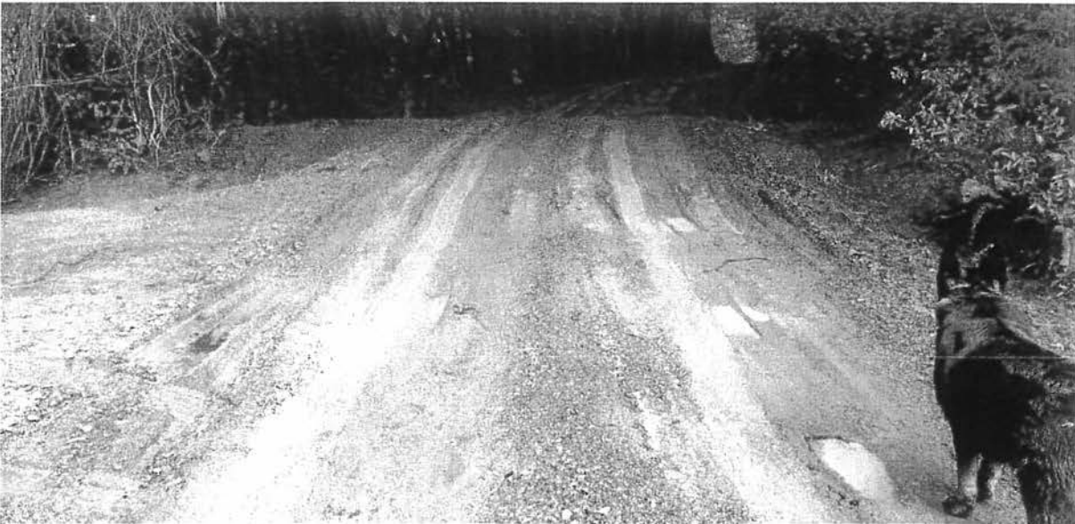
Photo looking northeast at Site 02. Additional competent rock surfacing is being prescribed here, and at other locations on the property where similar conditions exist. The majority of permanent roads on the property have adequate rock surfacing and a stable road surface. Certain locations require additional rock surfacing to create a stable road surface.
