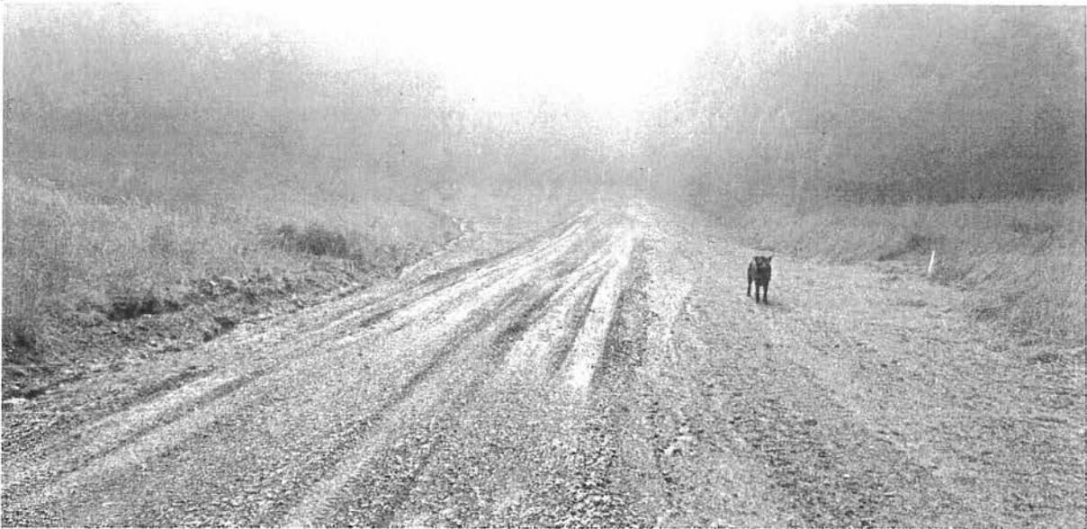
Photo looking downgrade at Site 10. Note road rutting and rock surfacing. Additional competent rock surfacing (4" – 6" crushed angular) will be required here.
