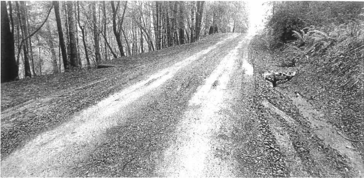
Photo looking west at Site 01. All ditch relief culverts have been recently installed during the fall of 2019 along with the grading, shaping, and rock surfacing of all permanently used roads. The ditch relief culverts were install correctly, only requiring the hand placement of additioan rock energy dissipaters at the outlets.
