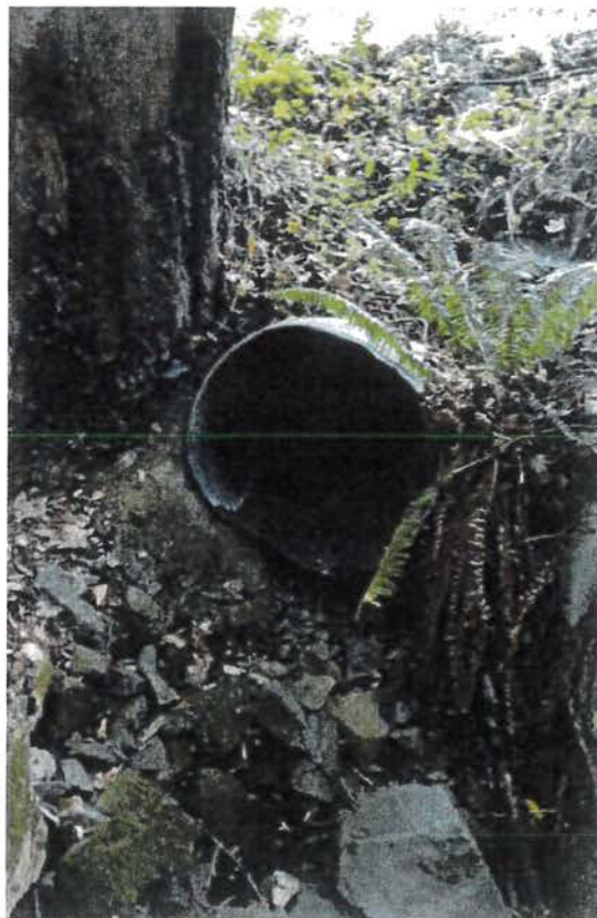
Photo looking at the outlet of the watercourser crossing at Site 22. Photo date 6-11-2016
