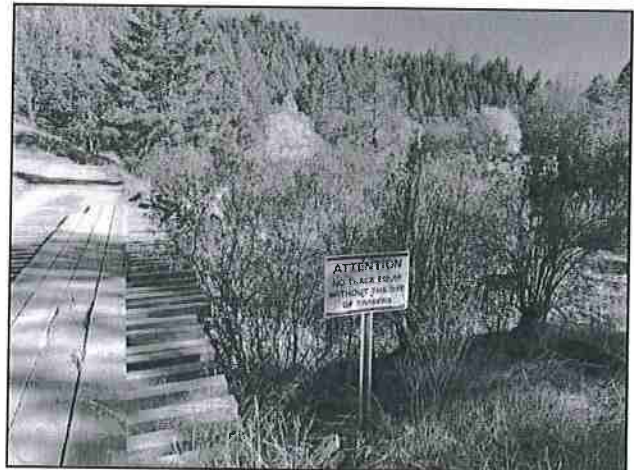
Photo #4 River Rd Warning sign @ RR Car Bridge
