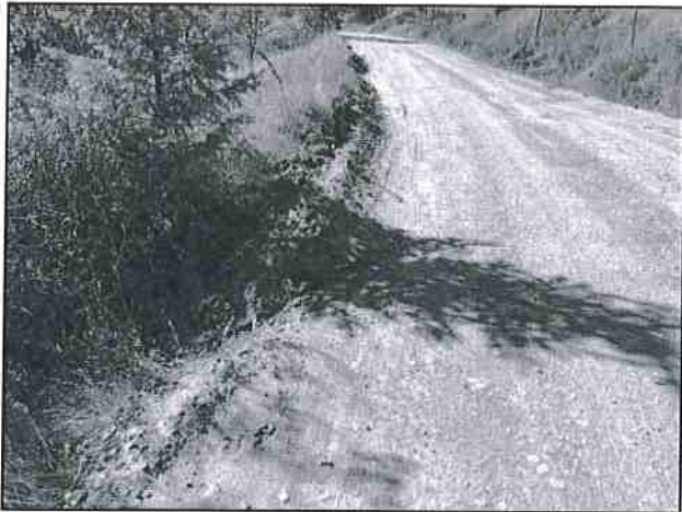
Photo #27 River Rd Looking NW @ Erosion & Tire Tracks Over Eroded Area
