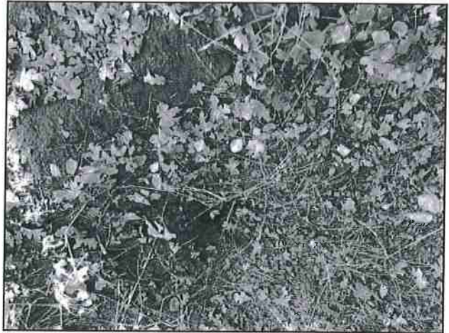
Photo #26 River Rd Looking @ Clogged 12" Culvert Out
