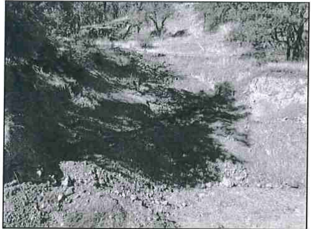
Photo #56 River Rd Looking @ Slide
