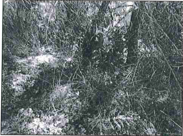
Photo #61 River Rd Looking @ Clogged Culvert In
