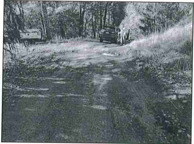
Photo #8 APN 208-241-019 Private Access Rd Looking @ Curve w/ Turnout & Drainage Issue
