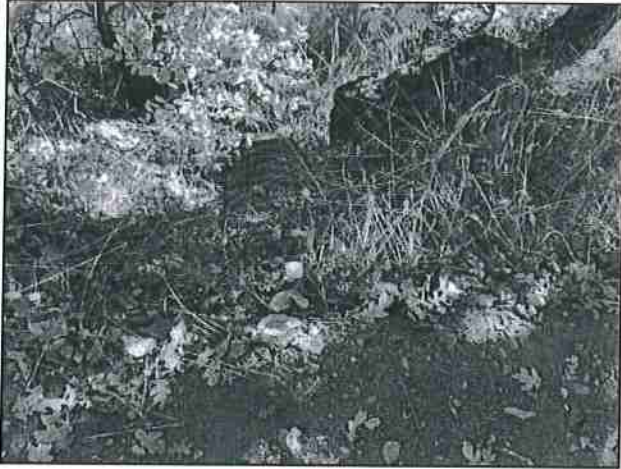
Photo #49 River Rd 12" Culvert Out
