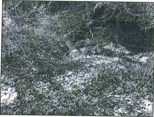
Photo #25 APN 208-241-019 Private Access Rd 18" Culvert Out
