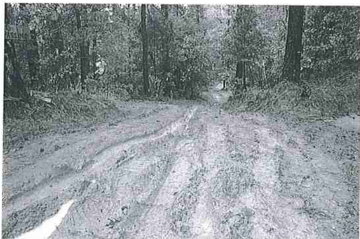
Figure 10. These ruts were created by wet-weather use of an unsurfaced, poorly drained road. Photo: Angela Wilson, Central Valley Regional Water Quality Control Board.
