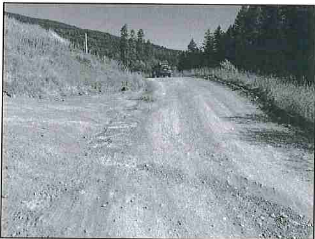
Photo #41 River Rd Looking East @ Curve w/ Pullout & Approach w/ Erosion from Drainage
