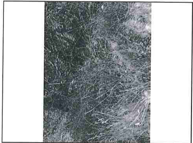
Photo #28 River Rd 12" Clogged 12" Culvert Out
