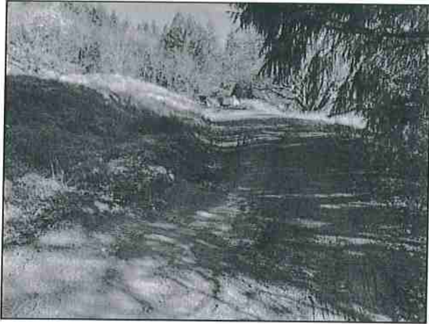
Photo #7 APN 208-241-019 Private Access Rd Looking NE @ Drainage Issue
