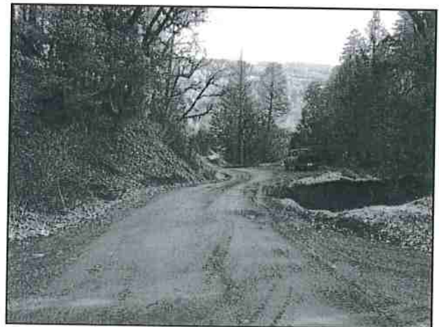
Photo #30 Intersection of River Rd & 208-241-019 Private Access Rd Looking SW @ Erosion Issue
