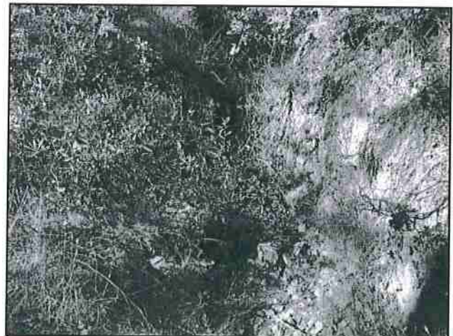
Photo #90 River Rd Looking @ Clogged 24" Culvert In
