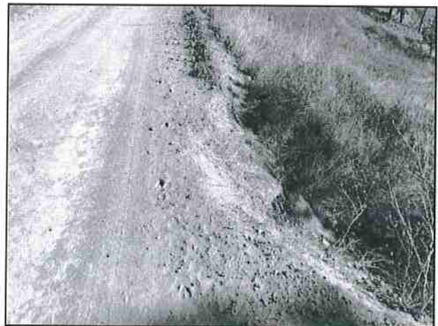
Photo #30 River Rd Looking SE @ Erosion
