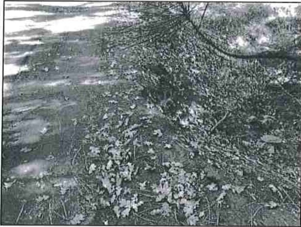
Photo #25 River Rd Looking @ Clogged 12" Culvert In
