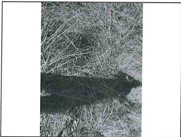
Photo #29 River Rd Looking @ Clogged 12" Culvert In
