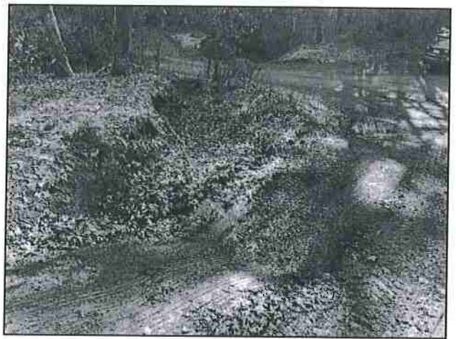
Photo #32 Intersection of River Rd & 208-241-019 Private Access Rd Looking SE @ Eros.- River RD
