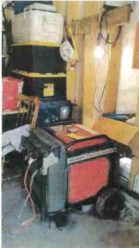
Photo 15. Generator currently used to run residence, to be replaced by solar
