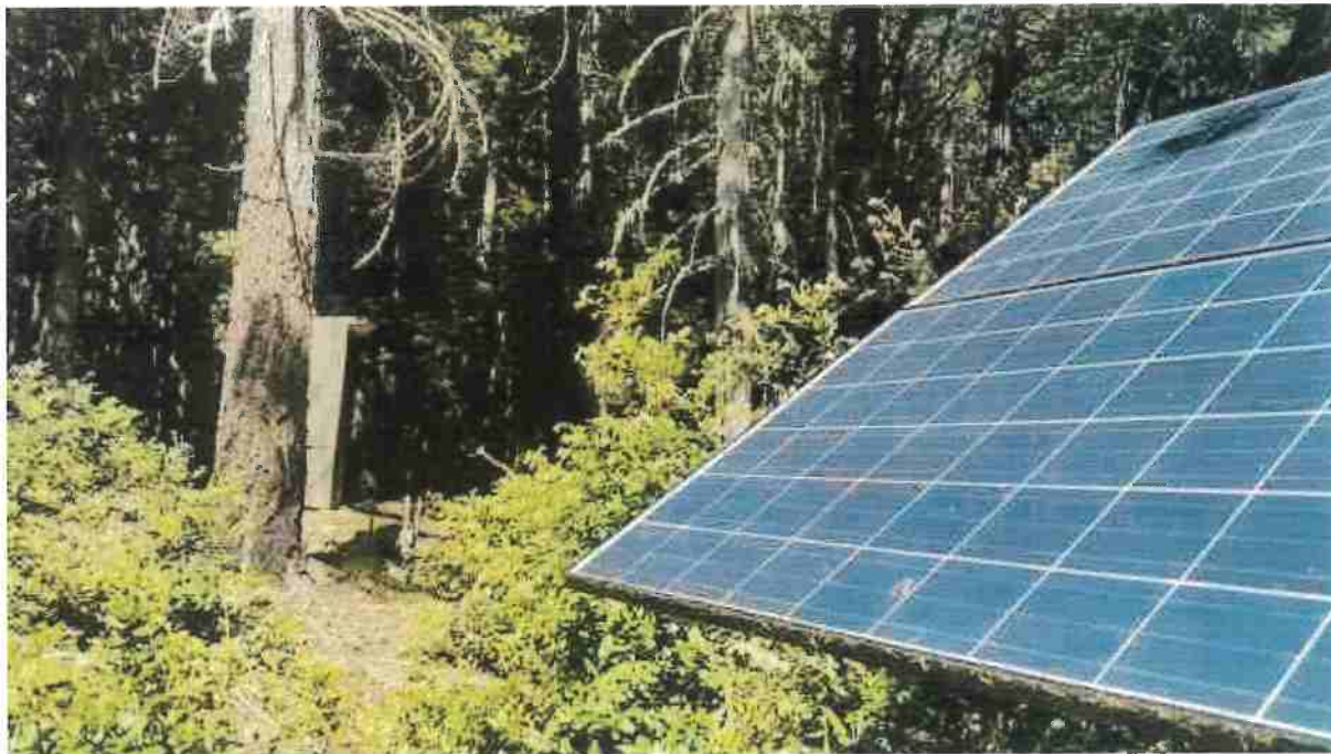
Photo 6. View of well shed and solar panel to run well pump
