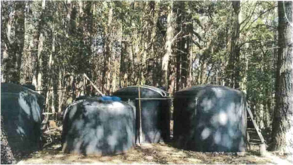
Photo 7. Water storage located just above Site C and adjacent to well and infrastructure
