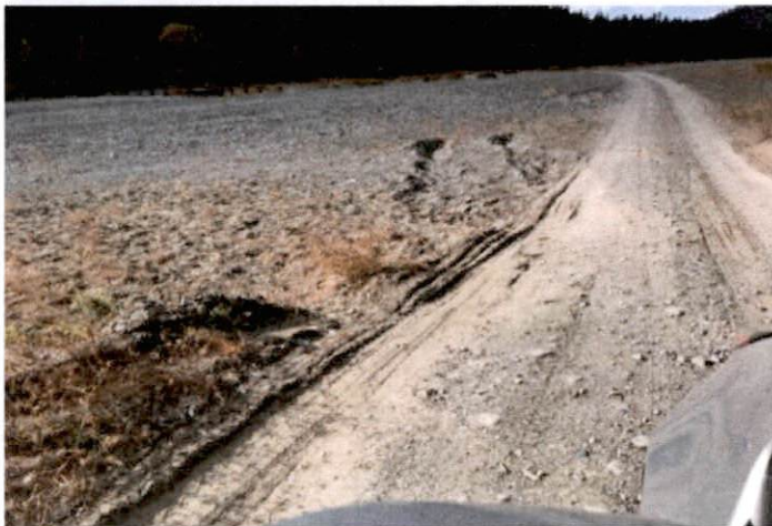
Photo No. 2. 14'-wide travel way across floodplain/gravel bar, unconsolidated shoulders. Tracks are evidence of vehicles getting stuck in the gravel off the travel way.
