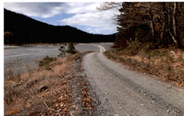
Photo No. 5. Looking back down to the floodplain/gravel bar, travel way is 12', inadequate shoulder, gravel surface.
