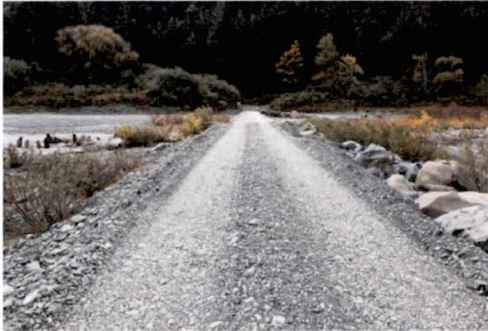
Photo No. 1. 11'-wide, one-lane, low water bridge and approach, no shoulder, gravel surface.
