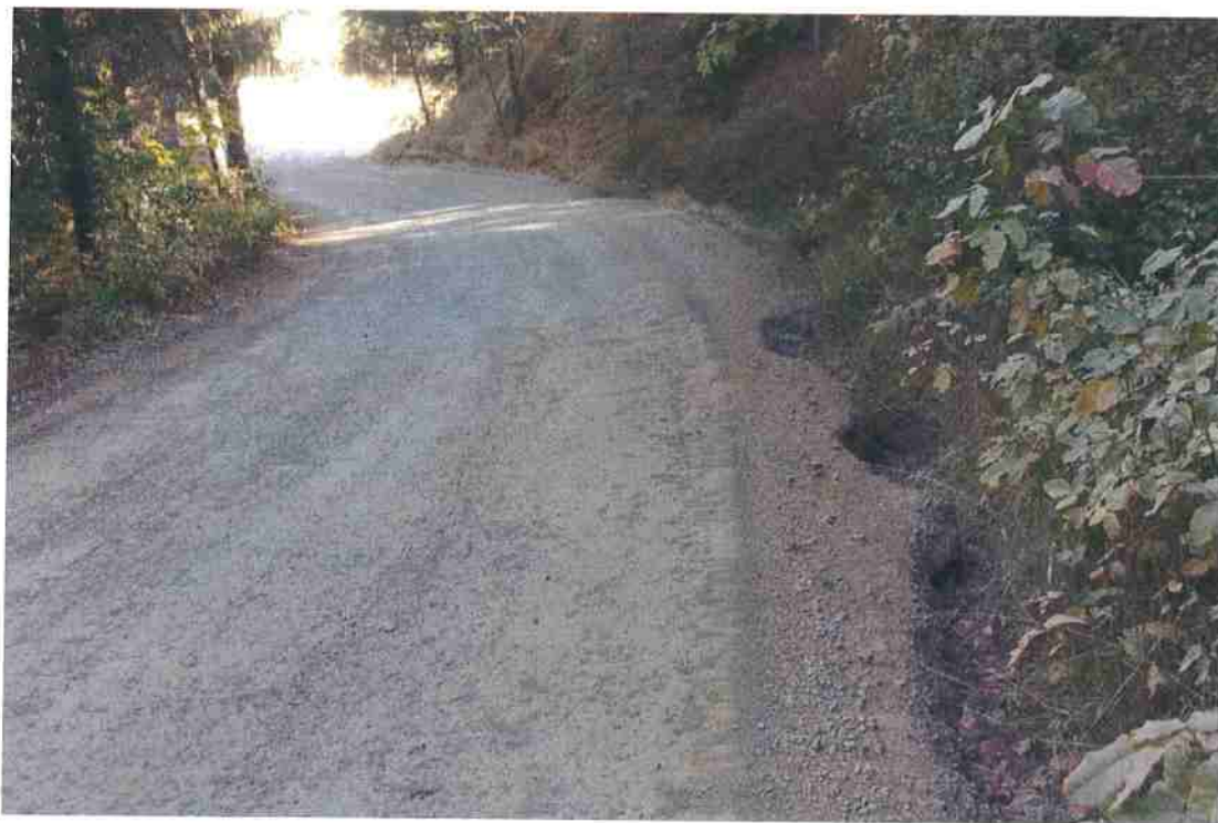
Photo 4. Mile 0.35: Inboard ditch eroding into road.
