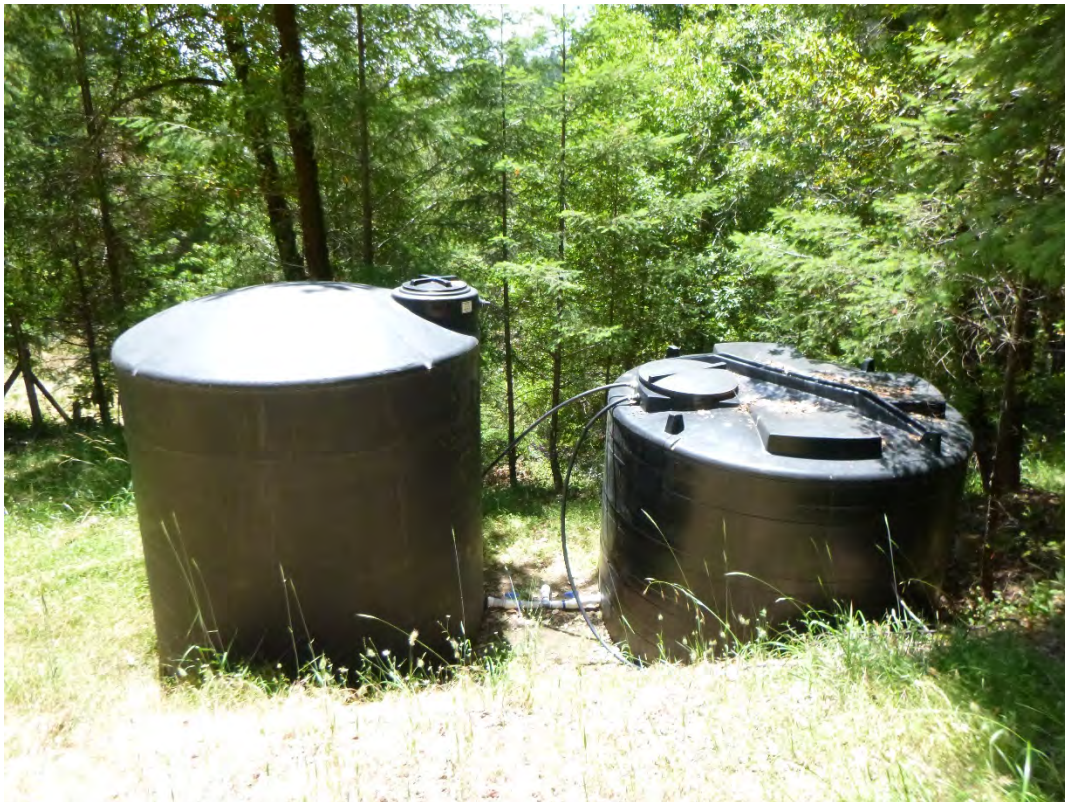
Photo 16. Water storage Middle (2.5K + 3K), Looking West
