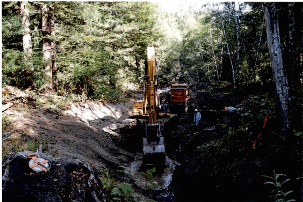
Construction of Lawrence Creek off channel habitat pond. Photo: Leah Mahan, NOAA
