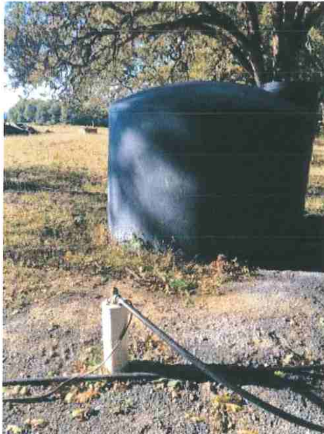
Well 2 and 2500 Gallon Holding tank
