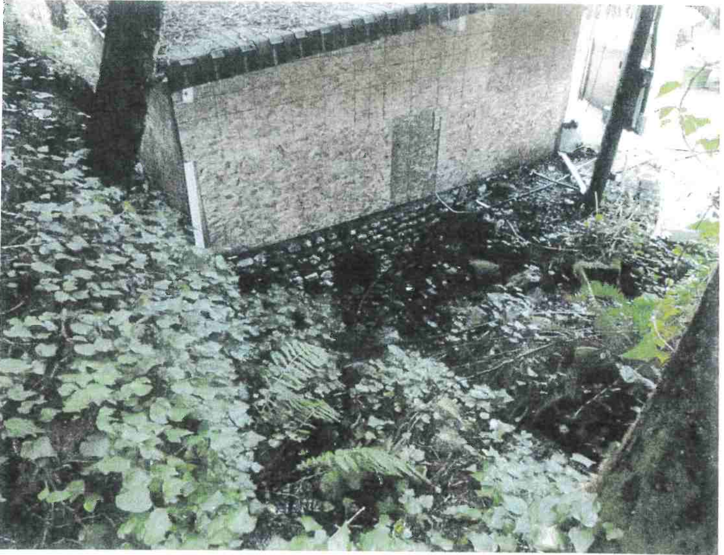
Picture 18: Inlet of 24" diameter Stream Crossing #2. This photograph was taken up stream of SC #2 approximately where the two watercourses converge. Surface water can be seen in the bottom center of this picture at the feet of the photographer. Photo date: 03/09/2018.
