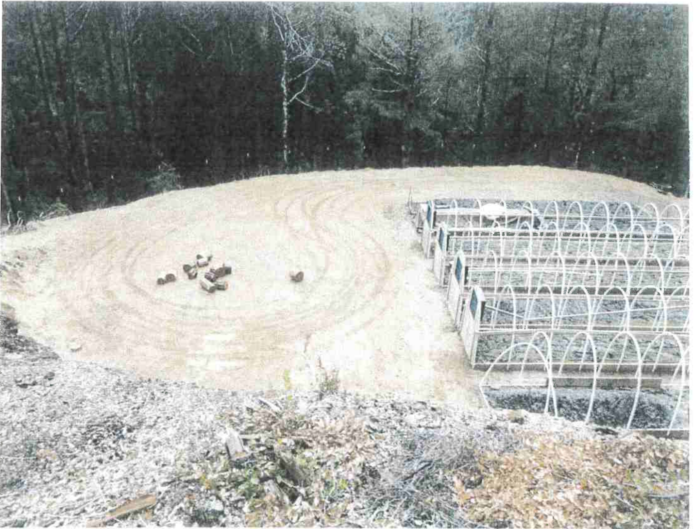
Picture 9: MP #2 is where a French drain shall be installed within the surface of the landing containing CS #1. The French drain will reduce run-off that currently drains along the access road and causing sediment transportation. Photo date: 03/09/2018
