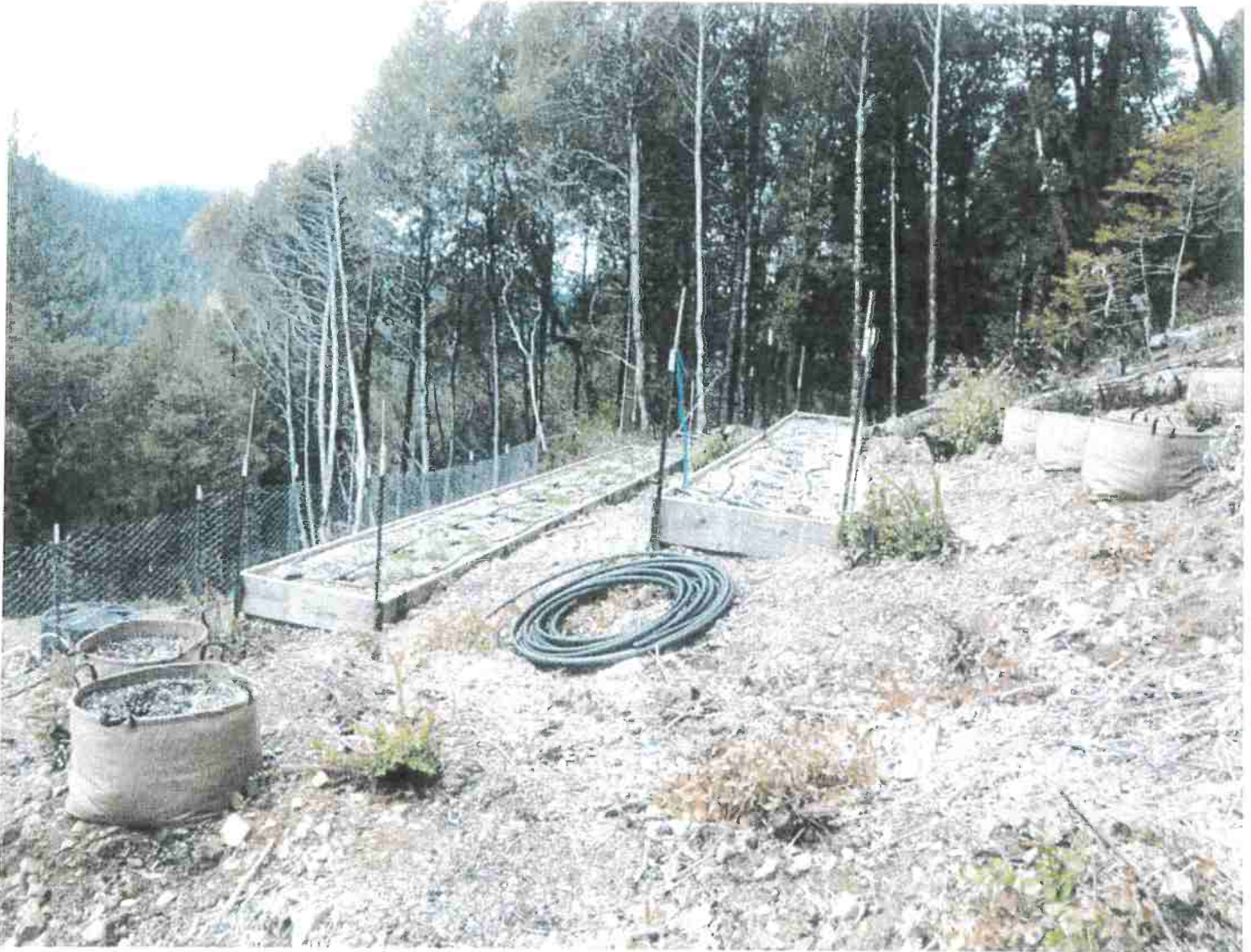
Picture 2: On top of the cut bank above the landing shown in Picture 1 sits another two 4' wide by 40' long soil beds surrounded by two hundred 30 gallon fabric pots for full sun cultivation. Photo date: 03/09/2018
