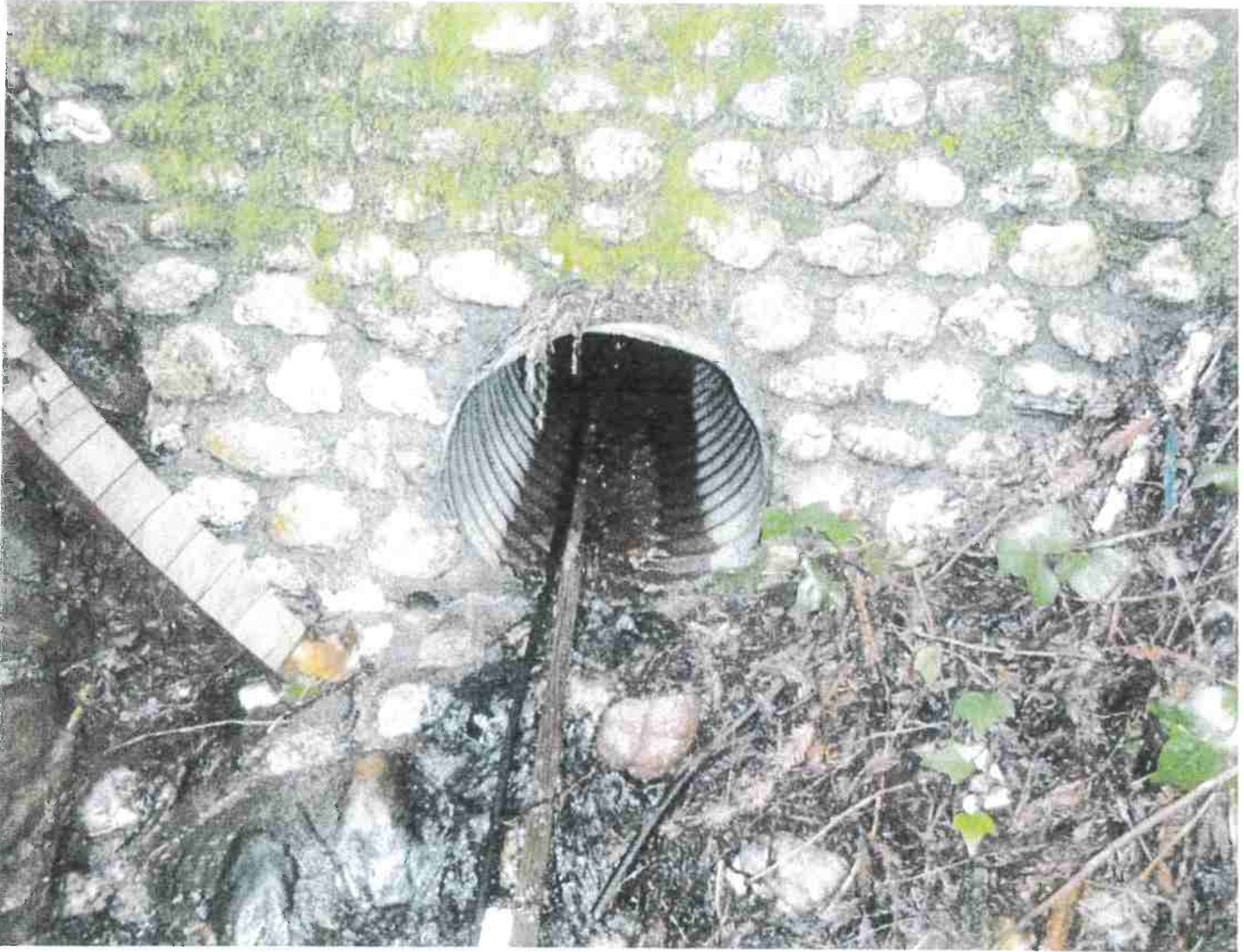
Picture 19: Outlet of 24" diameter Stream Crossing #2. The low rust line in the pipe lends evidence to the average annual flow level. Photo date: 03/09/2018
