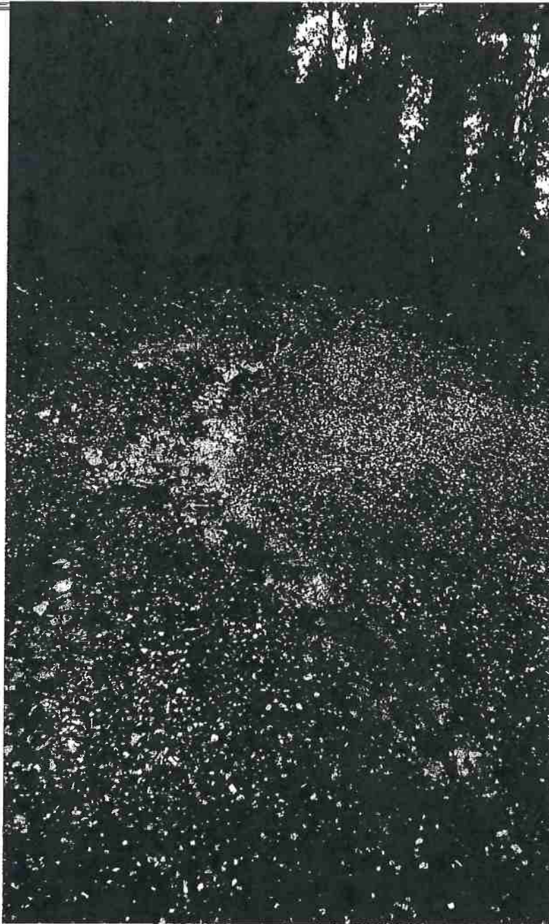
Picture 4: This is a photograph of the lower half of Road Segment 2, taken from near the bottom end and looking up the hill. As described above, there are ample locations where the water can be drained effectively by the installation of waterbars and or rolling dips. This segment of road appears to have had waterbars installed in the past as part past timber harvesting on the property from the early 1990s. Photo date of 1-19-2016.
