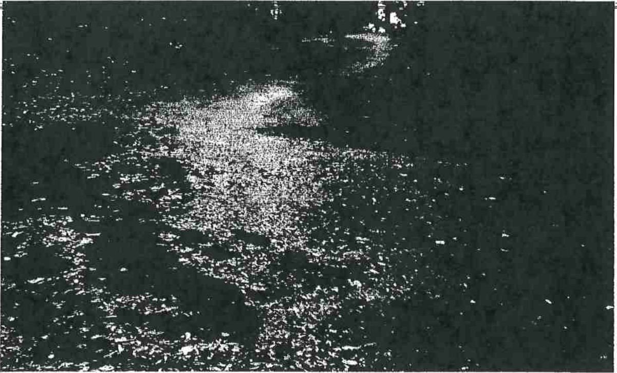
Picture 10: This is a photo of the Class III watercourse crossing at Map Point 8. A rocked ford crossing should be installed at this location to prevent future delivery of sediment during high flows. Photo date of 1-19-2016.
