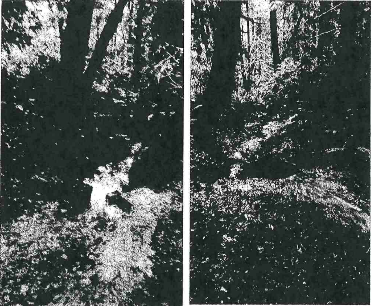
Pictures 8 and 9: The photo on the left is the water exiting the road at the location of Map Point 6. The photo on the right is water exiting the road after traveling down the road surface for approximately 90 feet from Map Point 7. Photo date of 1-19-2016.
