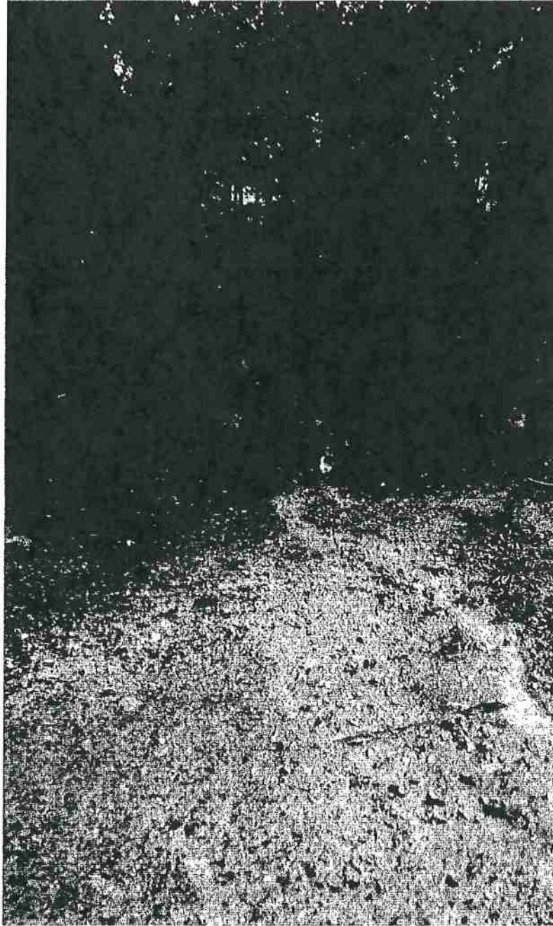
Picture 3: This is a photograph looking down the road at the top of Road Segment 2 taken from the developed cultivation area that is contributing runoff down the road surface during heavy rains (Map Point 4). Road Segment 2 as described above needs the installation of waterbars and or rolling dips. Photo date of 1-19-2016.
