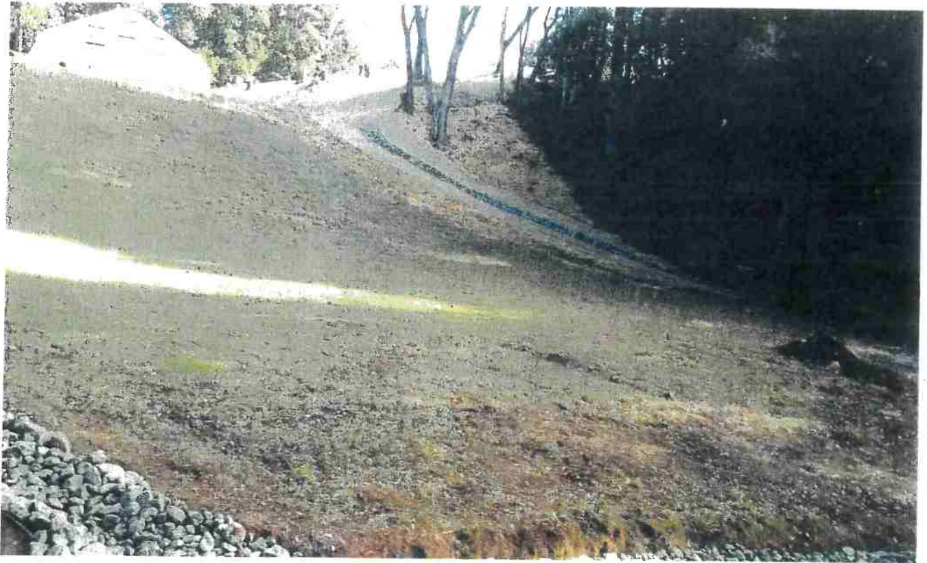
Picture 10: This is a picture of the newly rock lined drainage ditch that drains a "French drain" outlet that collects from the surface of the developed cultivation area. It ends above a swale that contains the top of a Class III watercourse. Photo date 12/2/2016
