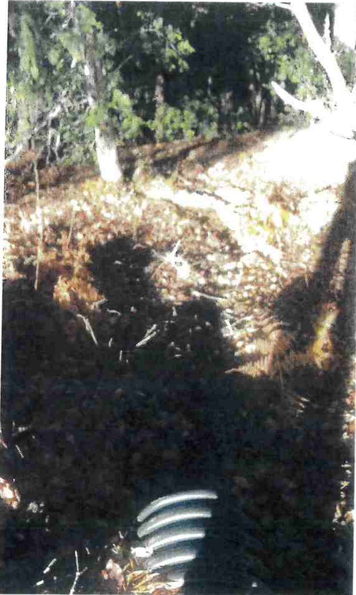
Picture 11: This is a picture of the outlet of the existing ditch relief culvert near in the southeastern corner of the property. The small drainage pictured below this culvert extends and meanders for approximately 300 feet to the small Class III watercourse below. Installation of a 15 inch diameter, ditch relief culvert approximately 120 feet northeast of this location, at Map Point 3, is expected to reduce the volume of water draining from this culvert so that runoff is dispersed prior to it reaching a watercourse. Photo date 11/3/2016
