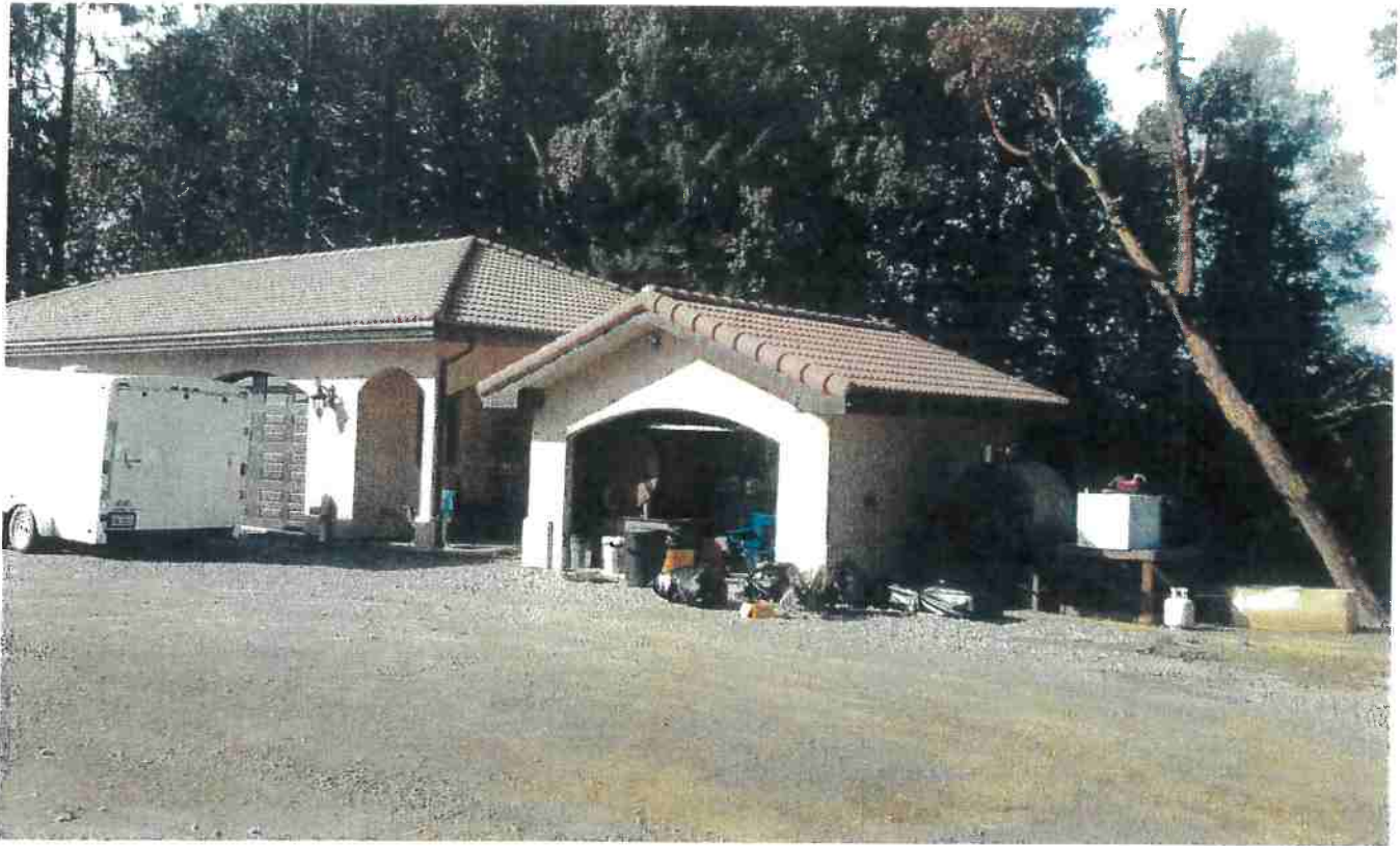
Picture 23: The large building in this picture is the garage / shop and the smaller building is the fuel storage shed. Off of the right side of the fuel storage shed are two gasoline storage tanks. The white square tank on the wooden platform needs secondary containment and both tanks need to be tarped or covered from precipitation during the winter to prevent secondary containment tanks from filling with rain. Photo date 11/3/2016
