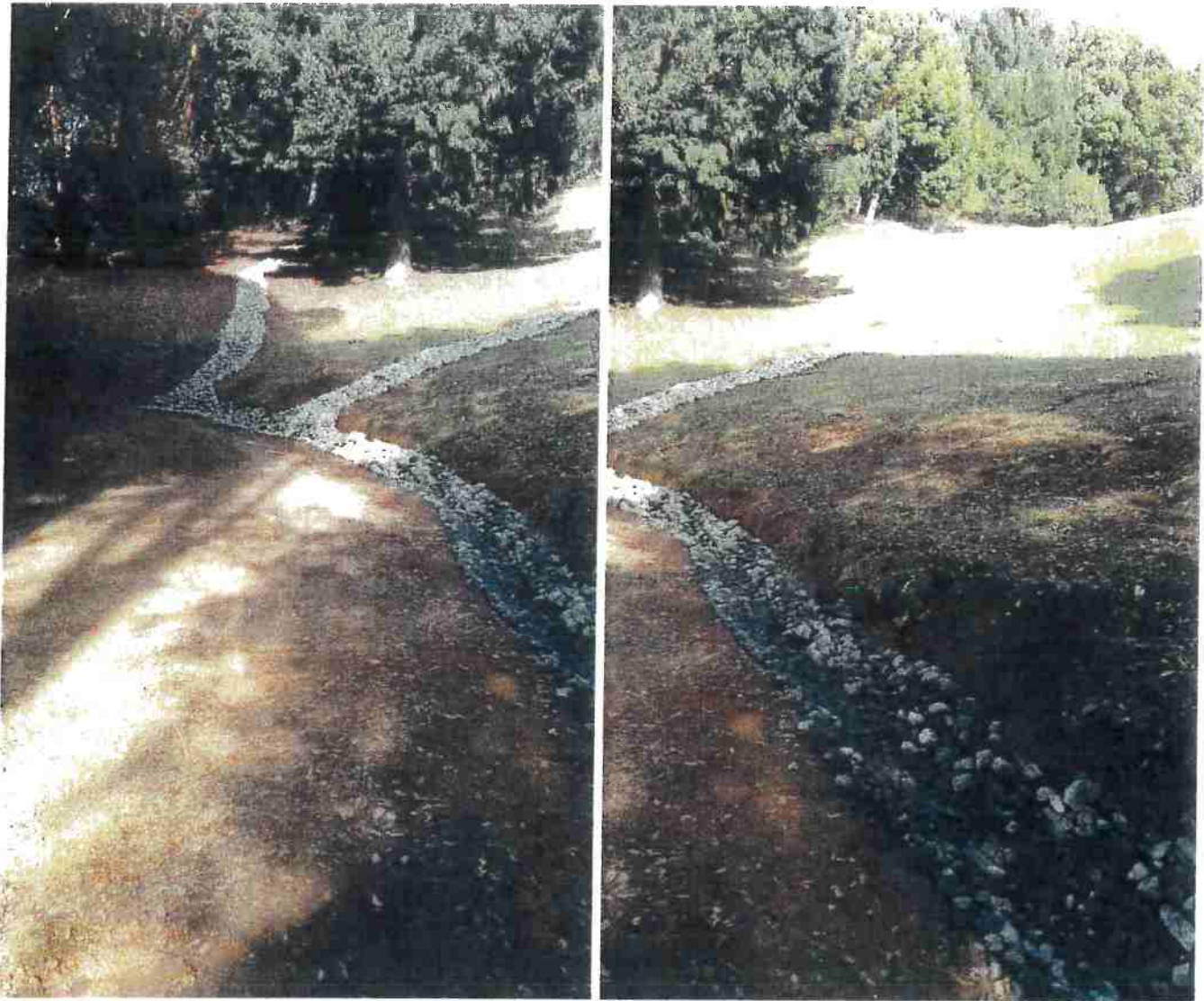
Pictures 4 and 5: These pictures show the bottom of the newly rock lined drainage channels and where they intersect with the newly rock lined inside ditch along Map Point 2. Photo date 12/2/2016
