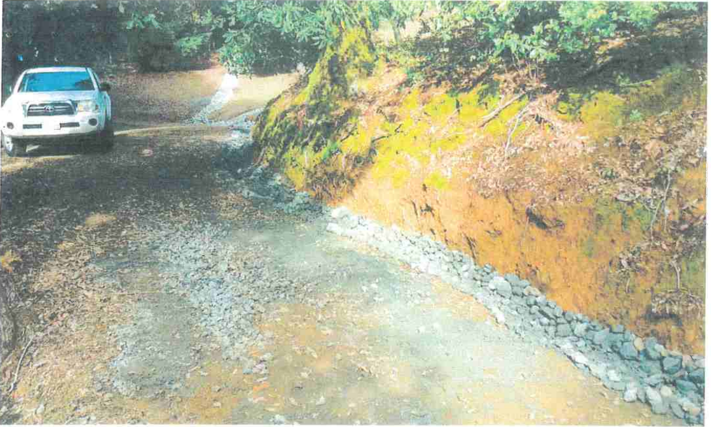
Picture 6: This is a picture along Map Point 2 showing the bottom half of the newly rock lined inside ditch taken from near the location of picture 2 above. Photo date 12/2/2016
