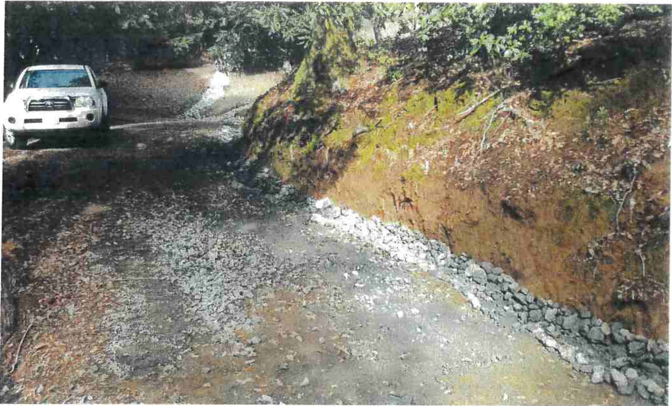
Picture 6: This is a picture along Map Point 2 showing the bottom half of the newly rock lined inside ditch taken from near the location of picture 2 above. Photo date 12/2/2016
