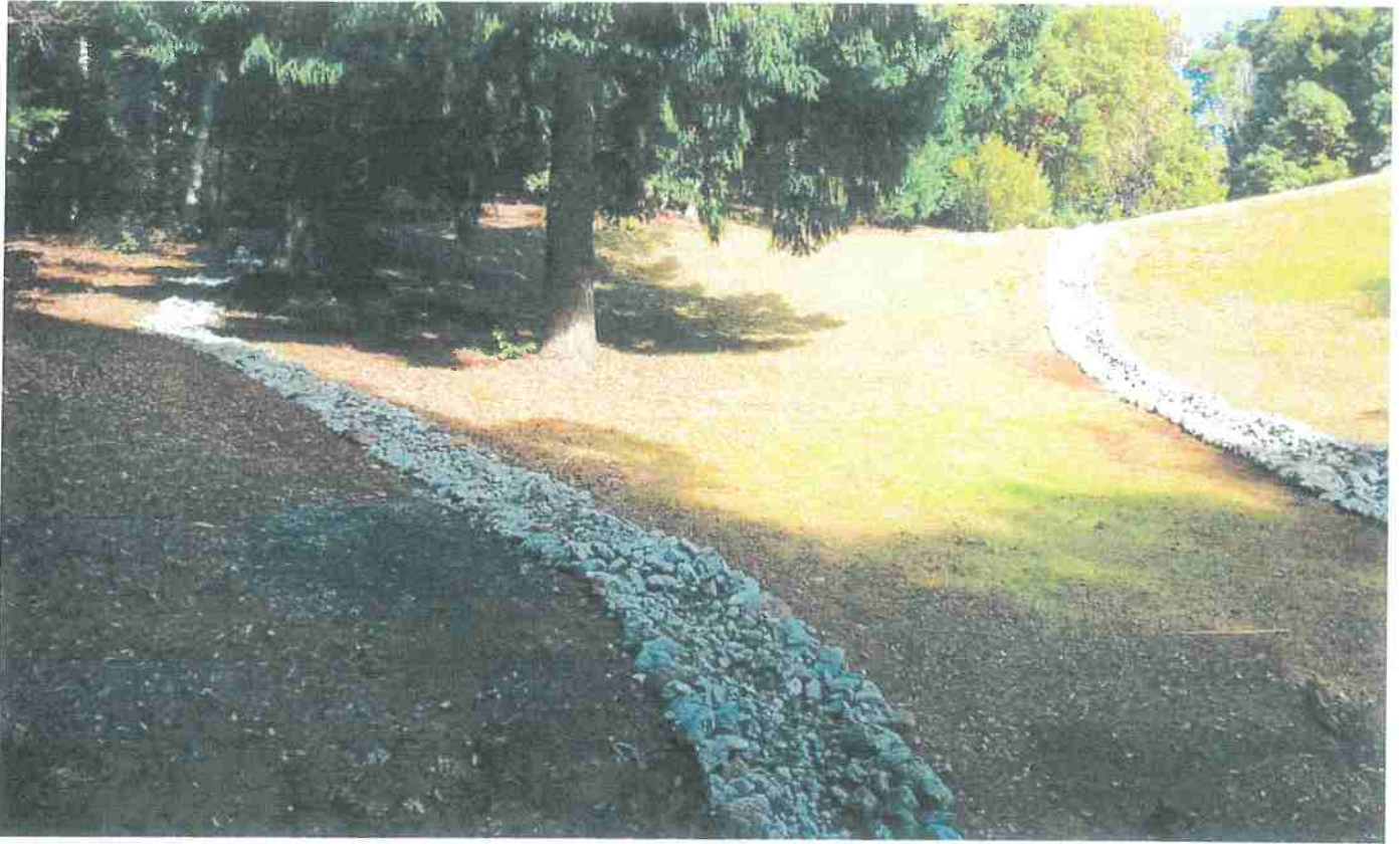
Picture 3: This is a picture of the newly rock lined drainage channels located upslope of Map Point 2. The channel on the left extends from the outlet of an existing ditch relief culvert. The channel on the right extends from the surface of the developed cultivation area. Photo date 12/2/2016
