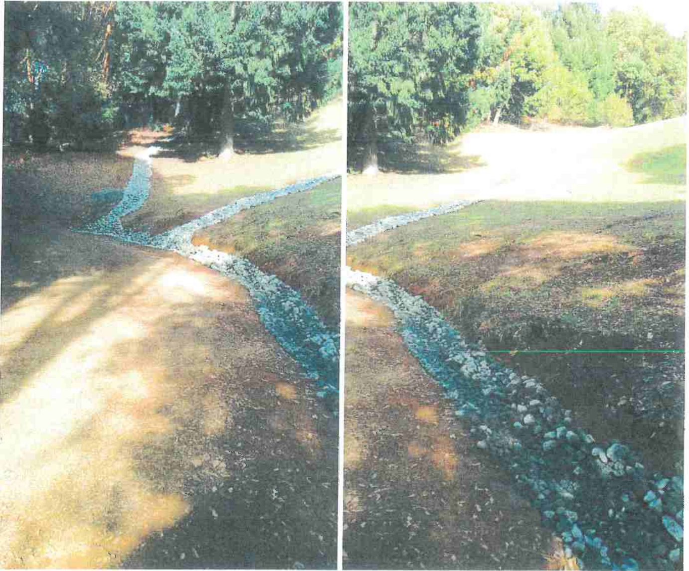
Pictures 4 and 5: These pictures show the bottom of the newly rock lined drainage channels and where they intersect with the newly rock lined inside ditch along Map Point 2. Photo date 12/2/2016
