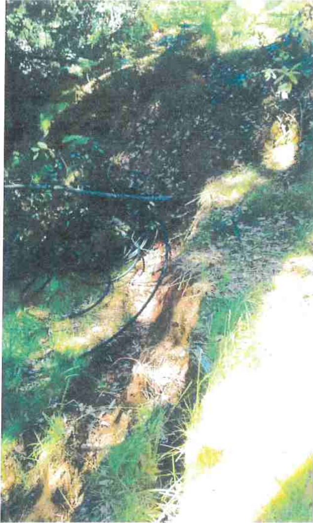
Picture 16: These are pictures of the recently slumped fill material shown as Map Point 6.5 on the WRPP Map. Slopes shall be recontoured as close as possible to the natural grade and aspect. Photo date 6/13/2017
